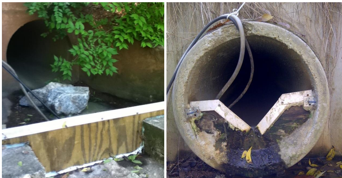
Figure 2.3. Inflow and outflow weirs (credit: Kathryn Shepard). The inflow weir is 112 cm wide and 22.5 cm high. The outflow weir is a 90-degree notch triangular weir. The point of the triangle is 8cm high, and the weir extends across the width of the outflow pipe opening.
