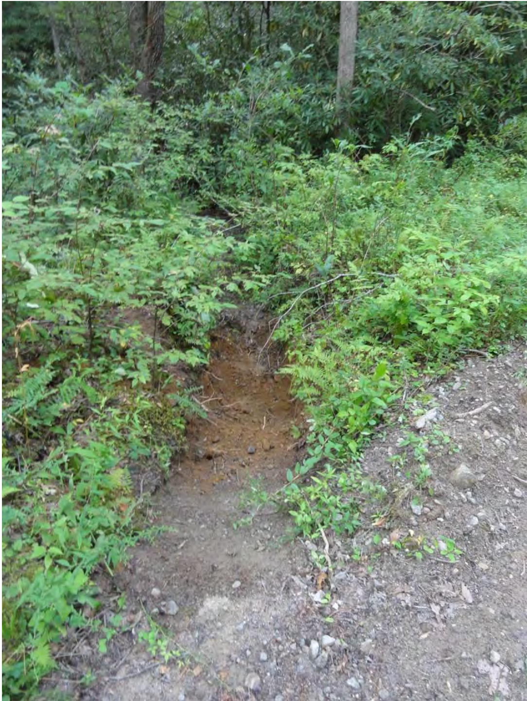
Figure 2.15. Photograph of a roadside sediment trap in Ball Creek Watershed that was recently cleaned out.
