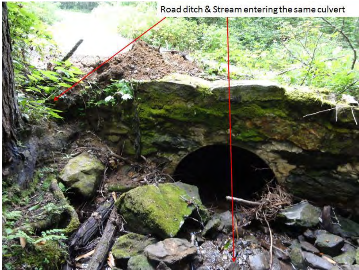
Figure 2.3. Photograph of road ditch sediment entering Reynolds Branch.
