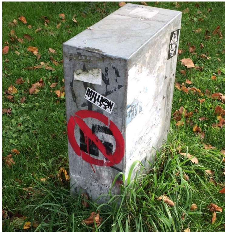
Utility box in Rosengård, Malmö City (November 2015, Own Work). 1
