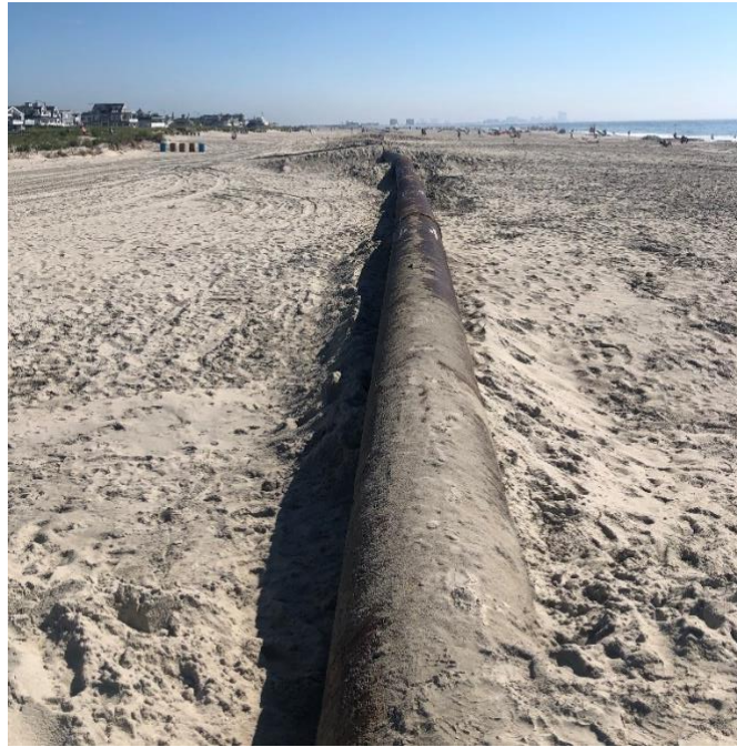
Figure 12: Seen on Ocean City’s beach, this pipe transports sand pumped from a dredge anchored offshore (photo taken by author)
