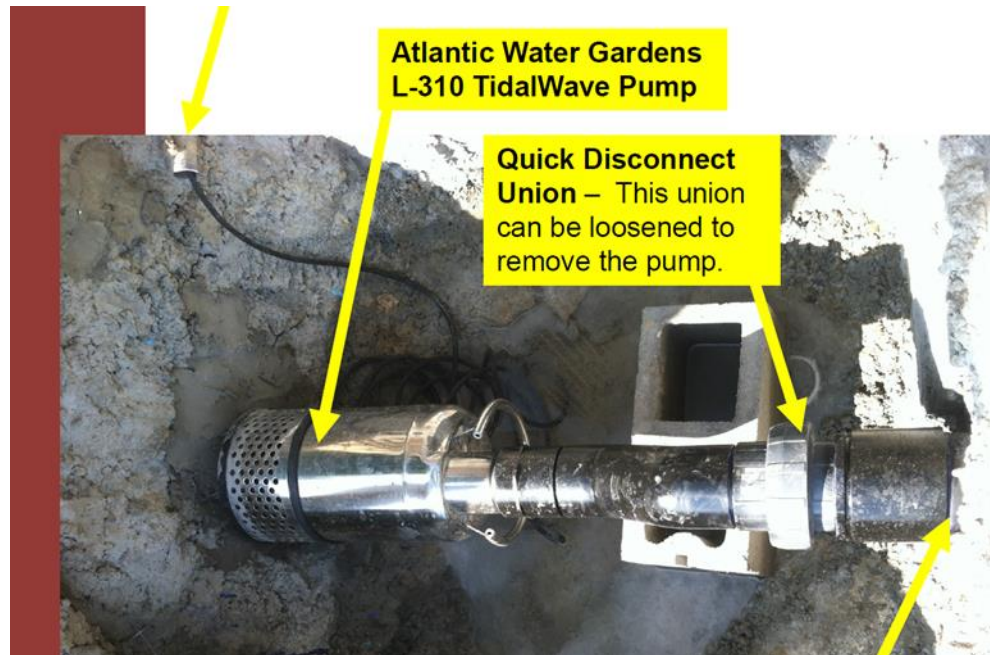
Figure 9. Typical Pump Installation (Photo taken by Reid Ferrero 2013)
