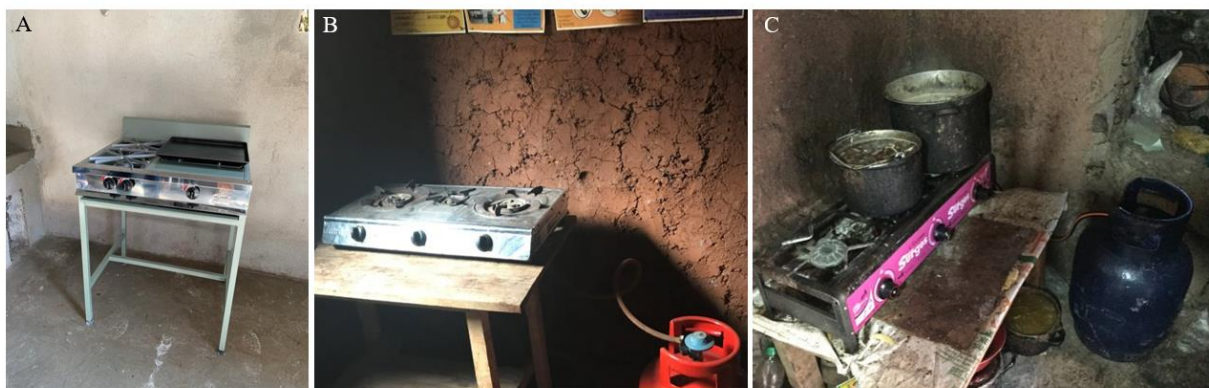
Figure 2.1a. LPG stoves installed in Guatemala (A), Rwanda (B), and Peru (C) in the intervention arm.
