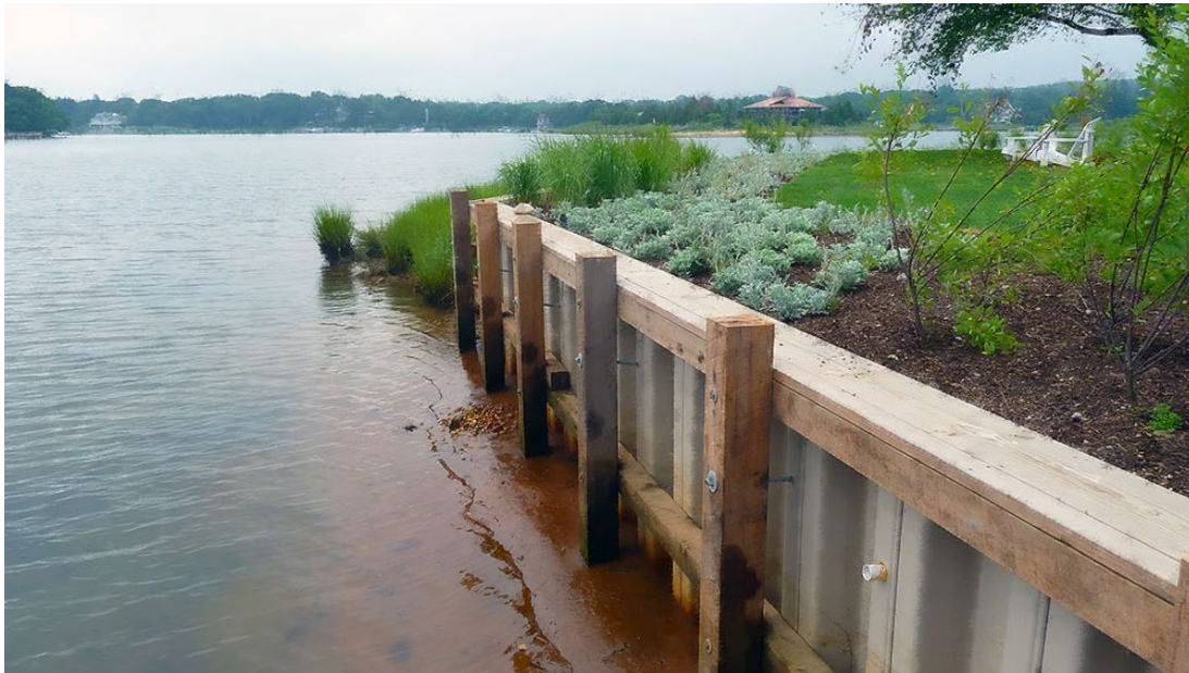
Figure 5: Image of Bulkhead adapted by First Coastal (First Coastal 2016)
