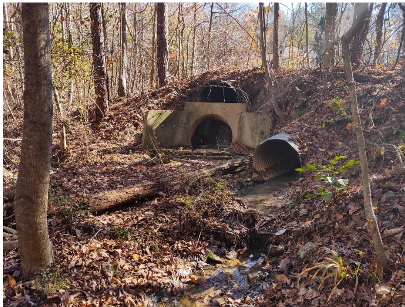
Figure 51 - 36in Corrugated Pipe Located in Residential Cul-de-sac
