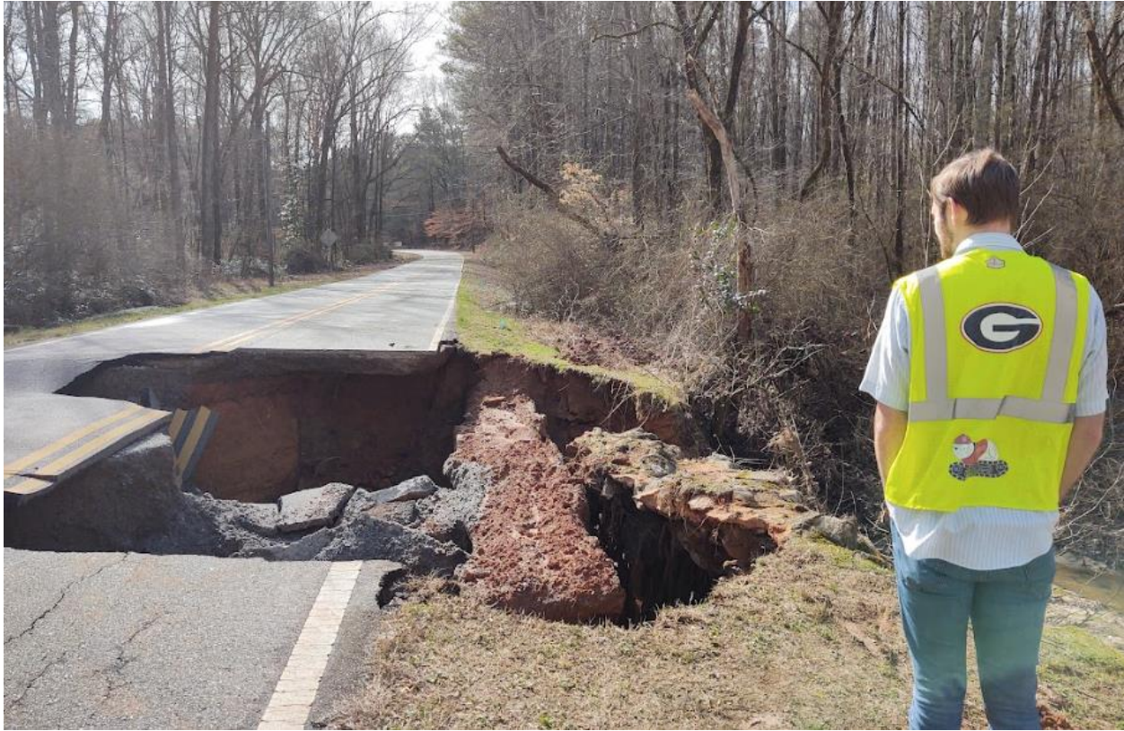
Figure 47 – Collapsed Road Above Corrugated Metal Pipe on Charlie Bolton Road
