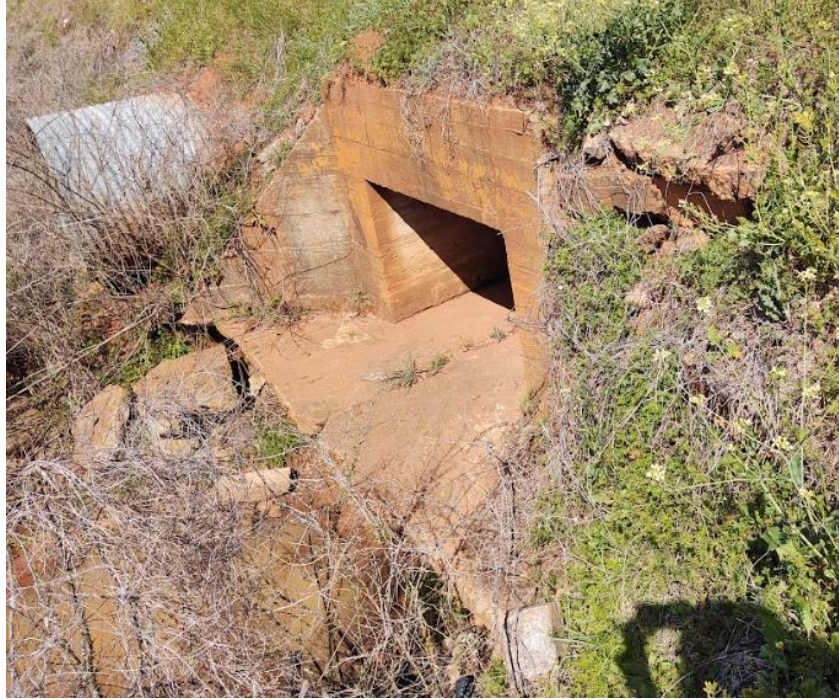
Figure 74 - Reinforced Concrete Asset with Severe Erosion and Stability Issues
