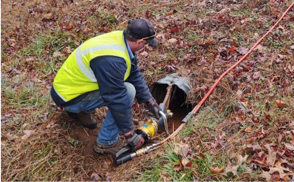
Figure 24 – Hydraulic “Jaws of Life” Tool Used to Reopen Corrugated Pipes
