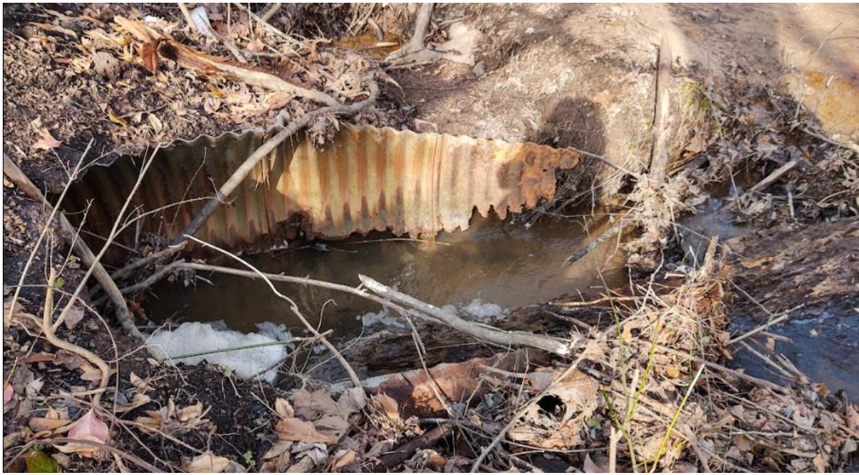
Figure 45 – Inlet of Voyles Road Barrel Culvert Showing Full Deterioration
