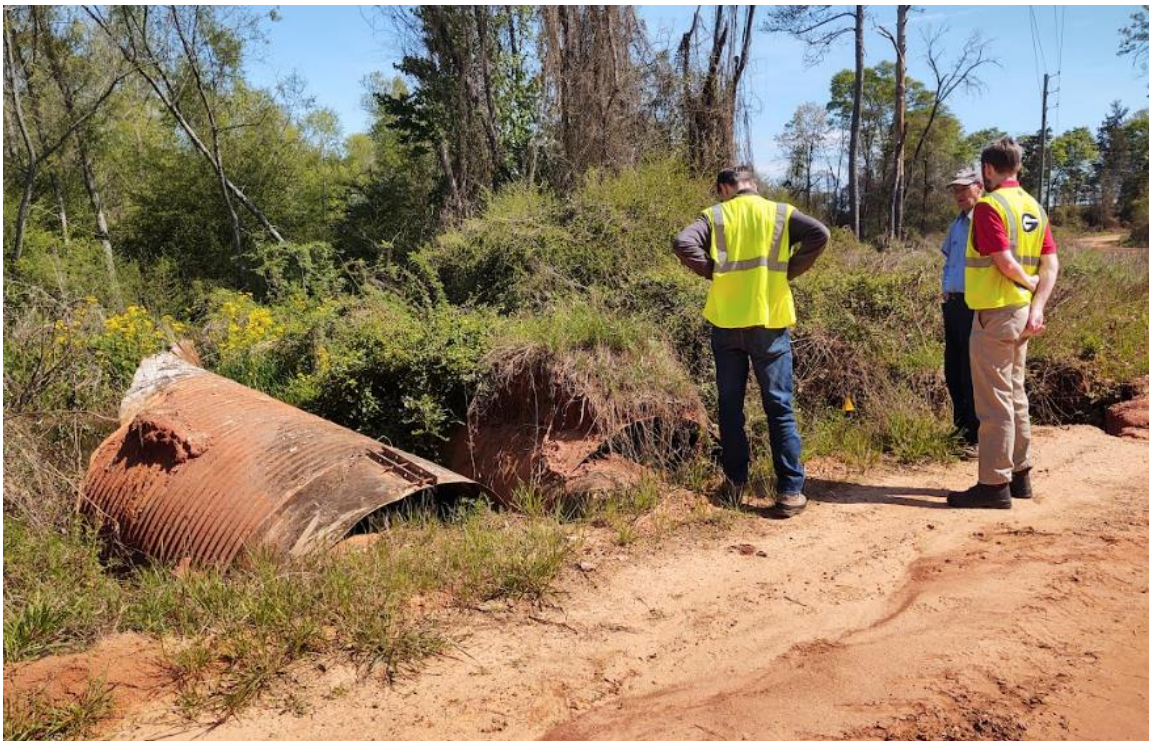
Figure 75 - Collapsed Large CMP Asset Located on Dirt Road
