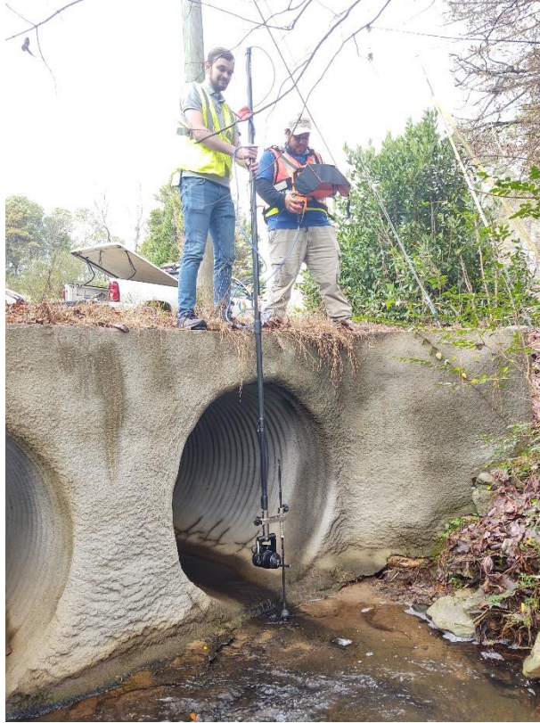
Figure 62 - Jared Palmgren and Fernando Zacarias Conducting a Culvert Inspection using a Pole Camera
