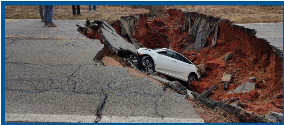
Figure 1 - Washed Out Culvert and Collapsed Road in Georgia
