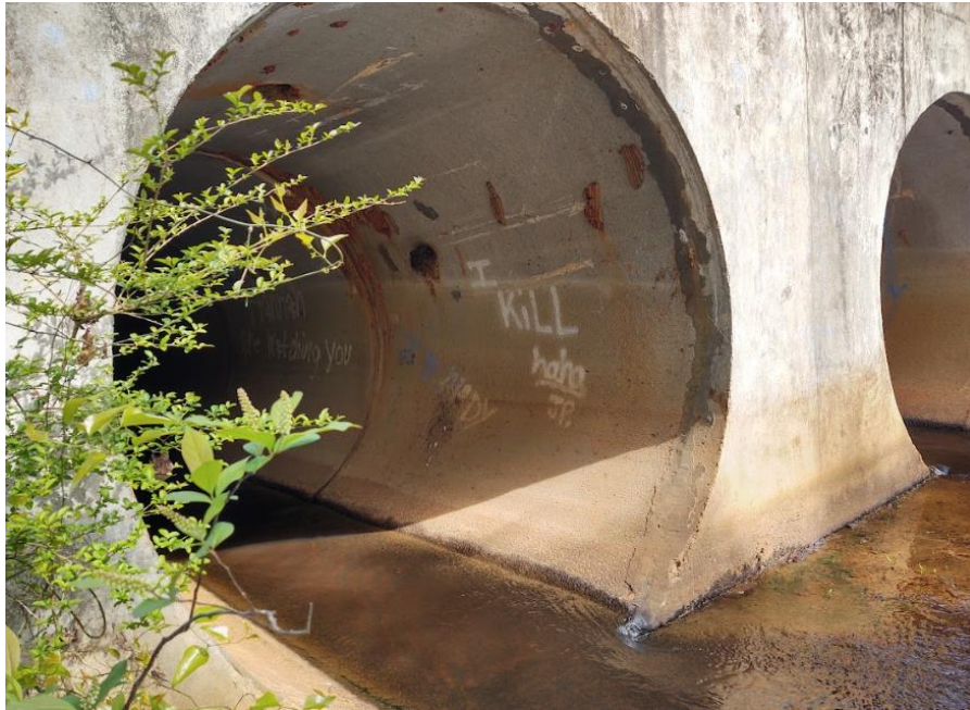
Figure 73 - RCP Asset in Fair Condition, Some Material Deterioration Apparent
