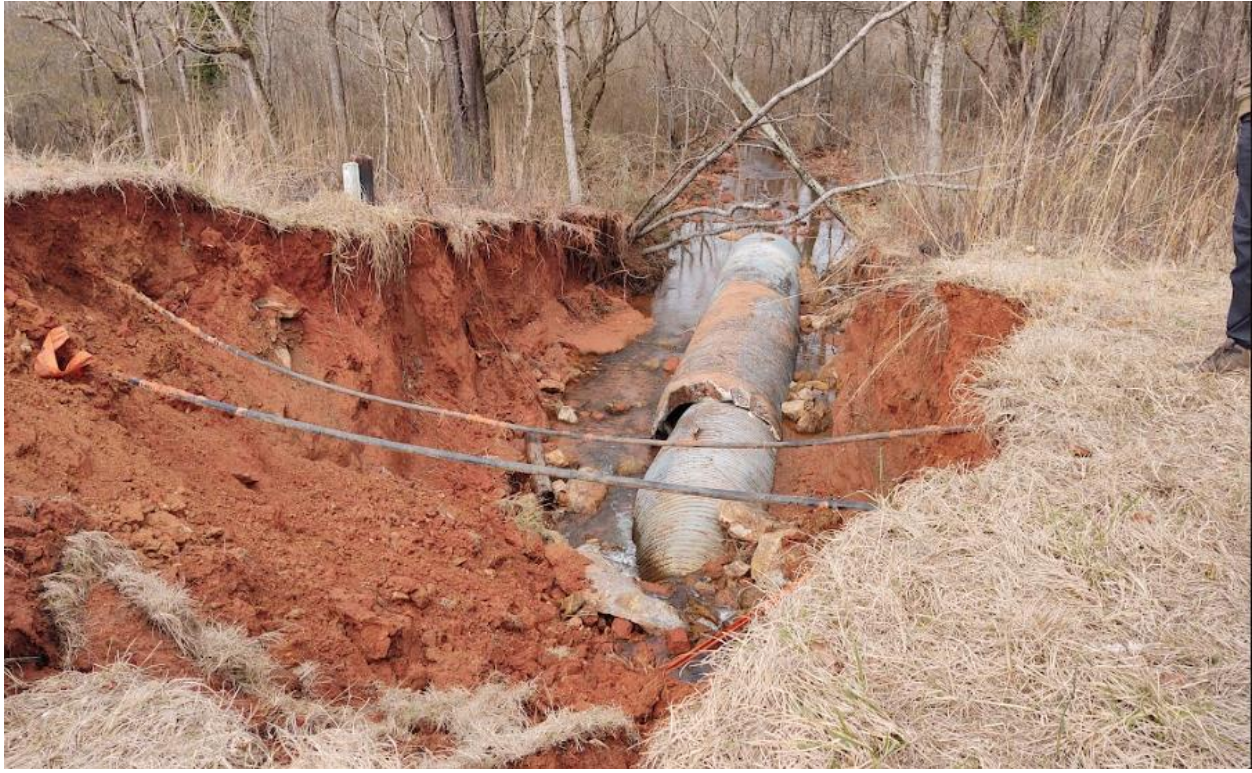
Figure 42 – Culvert Failure on Olympic Drive
