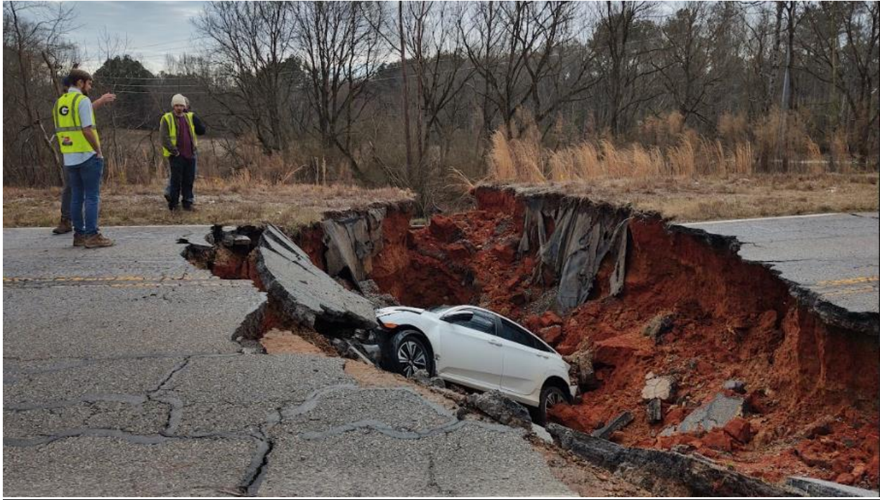
Figure 41 – Road Damage Caused by Culvert Failure on Olympic Drive
