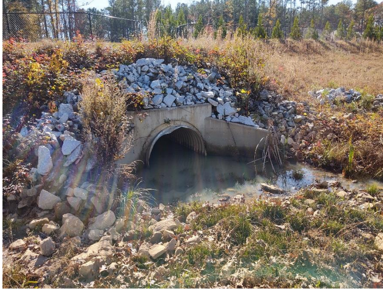
Figure 50 - 36in. Corrugated Metal Pipe Emptying into Retention Pond
