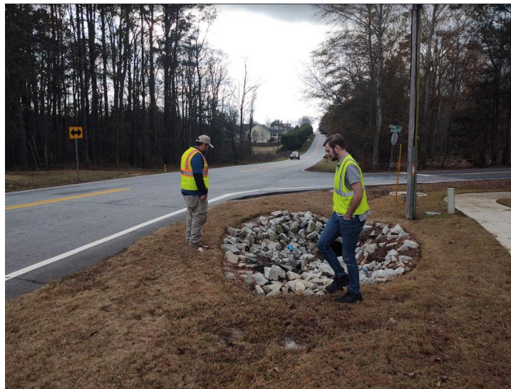
Figure 60 - Fernando Zacarias and Jared Palmgren conduct a Level 1 Inspection of a Flair End Culvert
