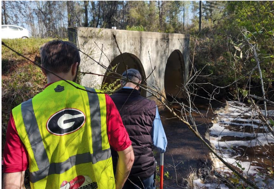
Figure 71 - UGA Research Assistant, Jared Palmgren, and Public Works Director, Jim Littlefield, Preparing to Inspect Asset
