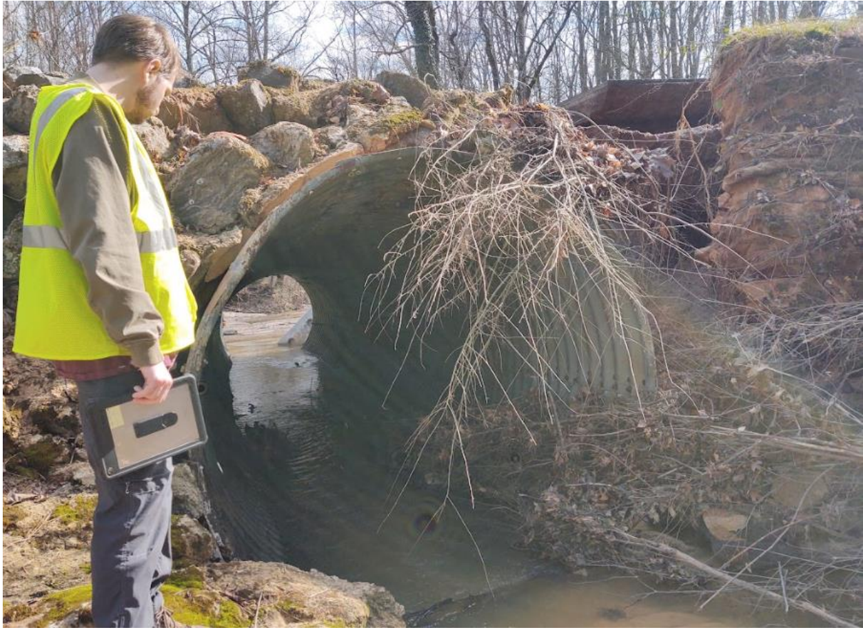
Figure 48 – Interior of Asset #4 and Surrounding Collapsed Roadway.
