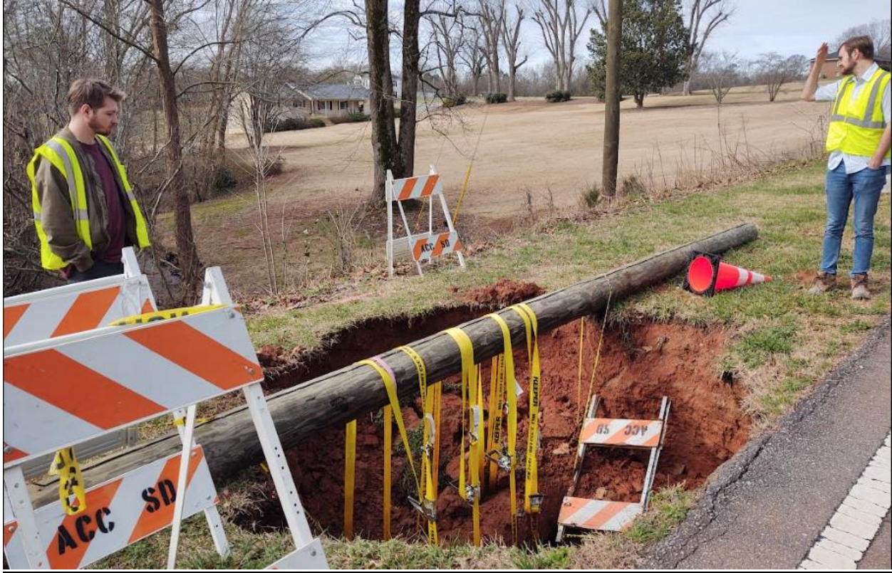
Figure 43 – Sinkhole Caused by Culvert Failure on Voyles Road
