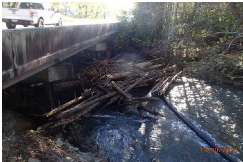
Figure 159 – Logjam at Bridge 187-0006-0 (GDOT, 2020)
