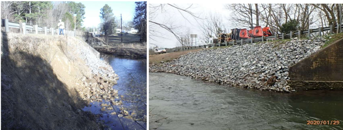
Figure 57: Bridge 213-0033-0 Left Shoulder 2016(Right) vs 2020(Left)
