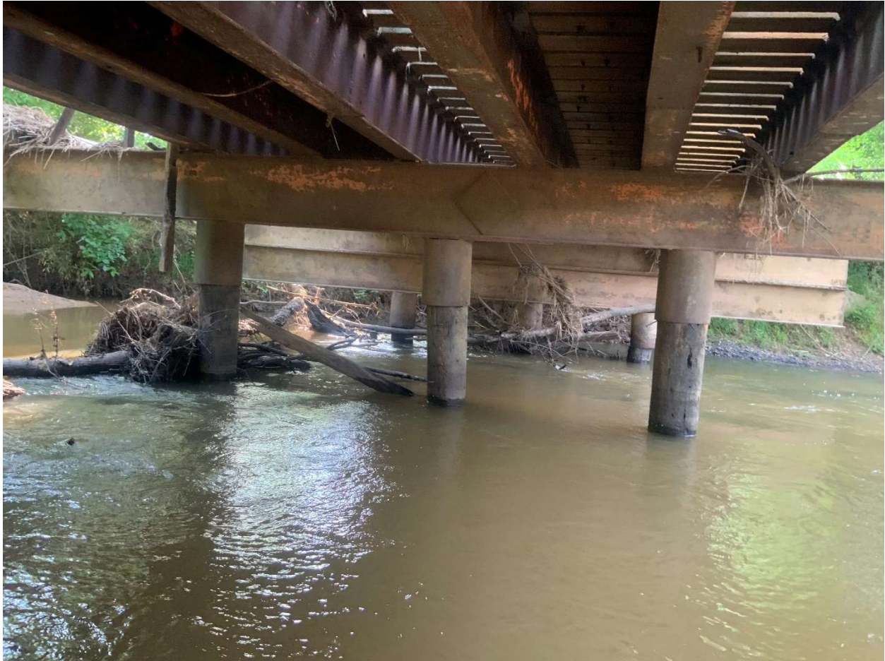
Figure 229 – Bridge 045-5027 Steel Pier Cap Condition (GDOT, 2022)
