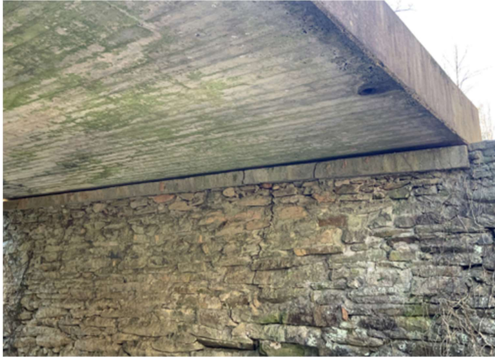
Figure 215 – Bridge 123-0036-0 Settlement Cracking (GDOT, 2022)
