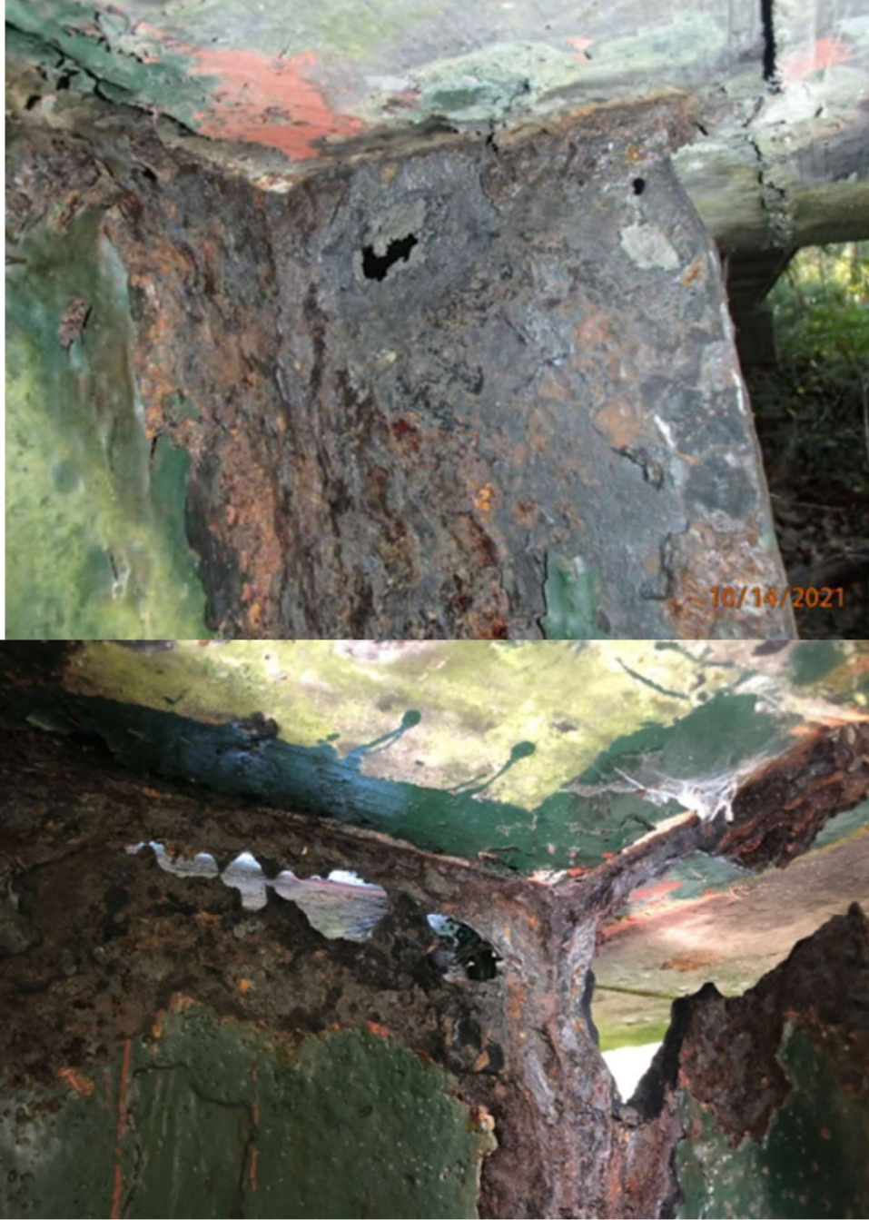
Figure 178 – Bridge 111-5002-0 Steel Pile Conditions (GDOT, 2021)
