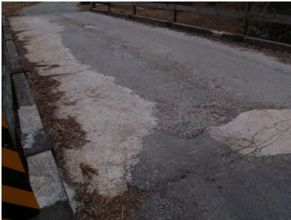
Figure 275- Bridge 291-5044-0 Deck Condition (GDOT, 2014)
