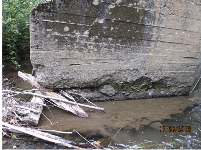
Figure 61 - Concrete Loss on Abutment 3 (GDOT, 2019)
