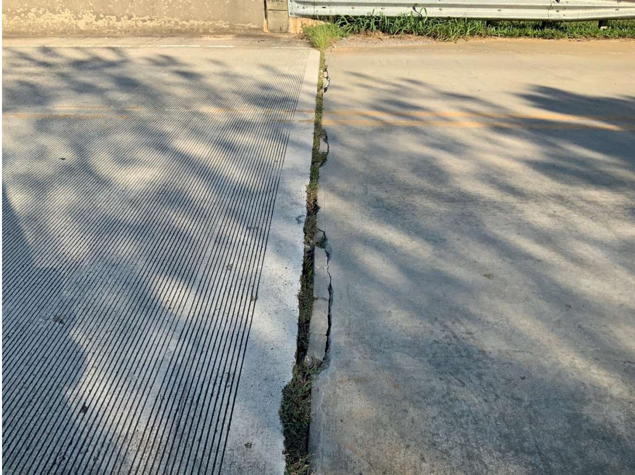
Figure 220 – Bridge 157-5084-0 Failed Compression Joint (GDOT, 2022)
