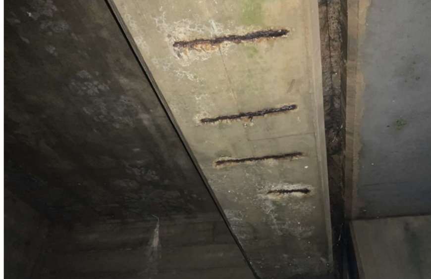
Figure 92 – Bridge 295-0015-0 Typical Girder Spalling (GOT, 2021)
