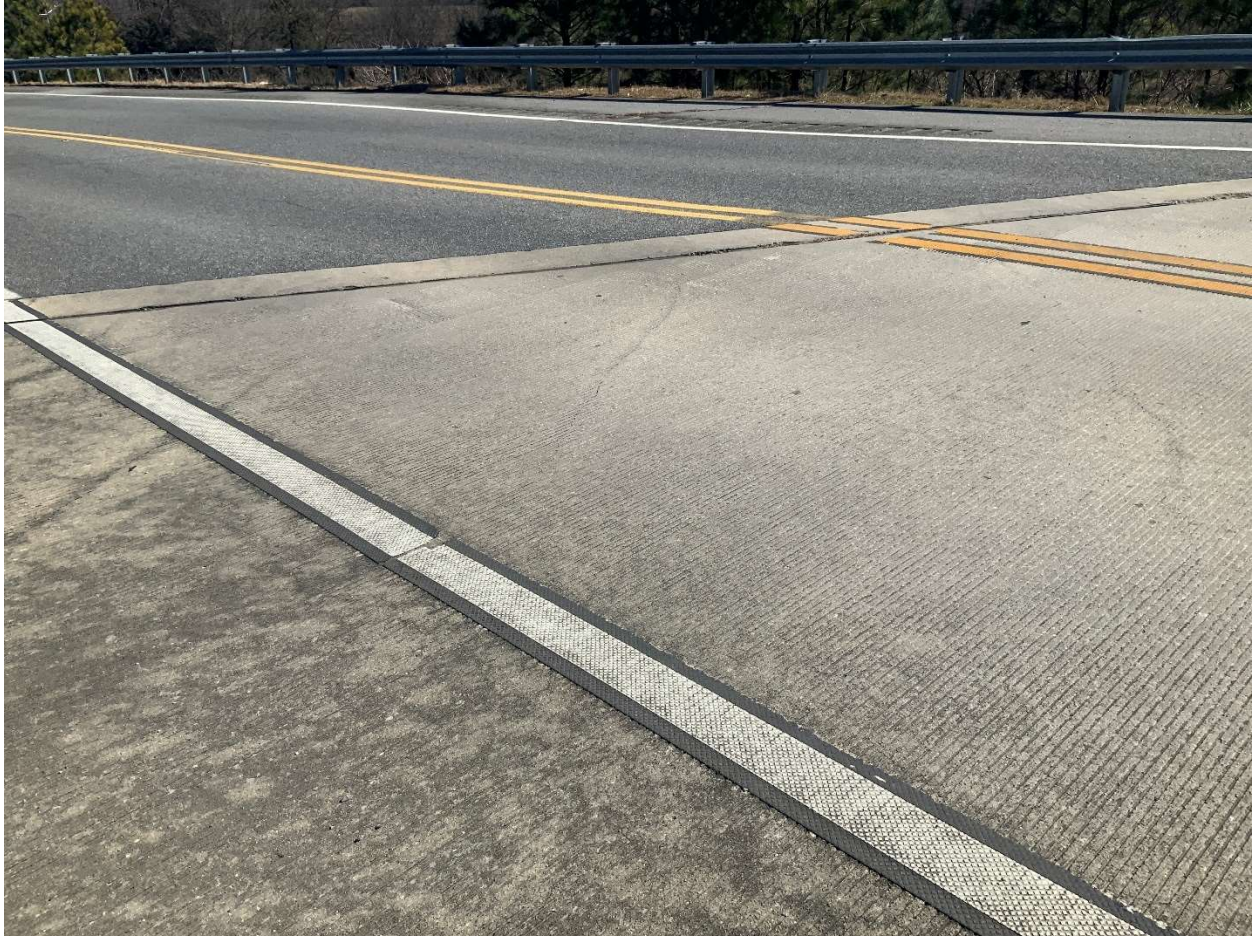
Figure 219 – Bridge 213-5045-0 Bridge Deck Cracking at Abutment (GDOT, 2022)
