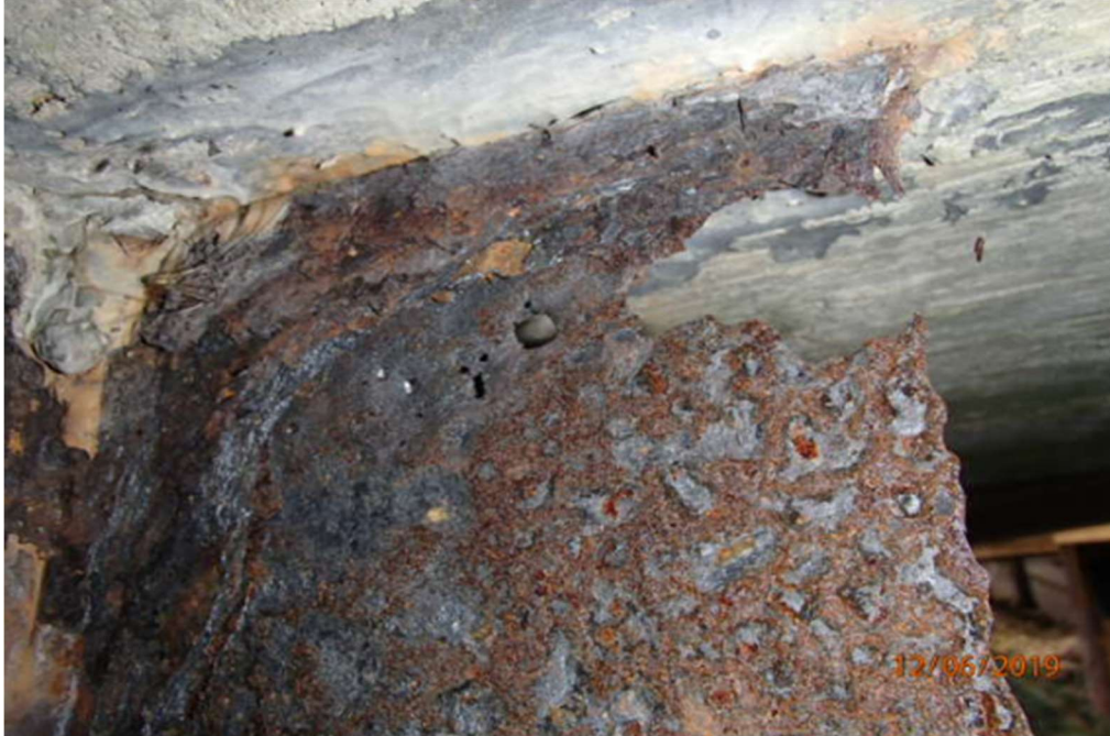
Figure 158 – Bridge 187-0006-0 Pile Condition, 2019
