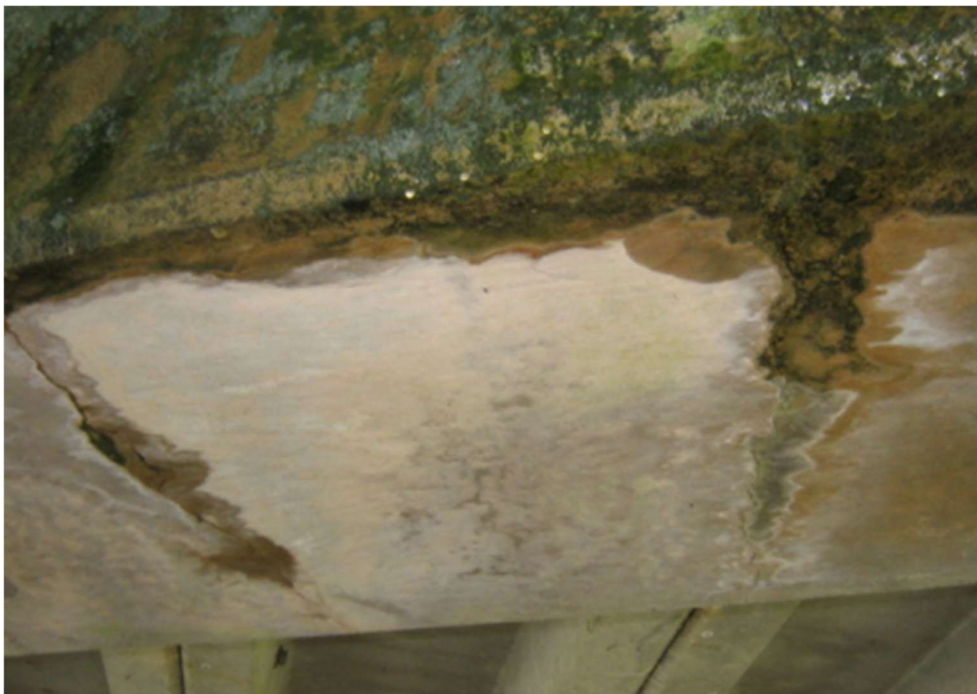
Figure 143 – Bridge 313-5028-0 Pier Cap Cracking (GDOT, 2022)
