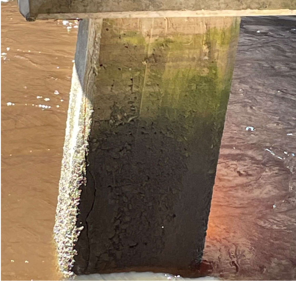
Figure 286 – Bridge 039-0009-0 Prestressed Concrete Pile Typical Cracking and Abrasion (GDOT, 2021)
