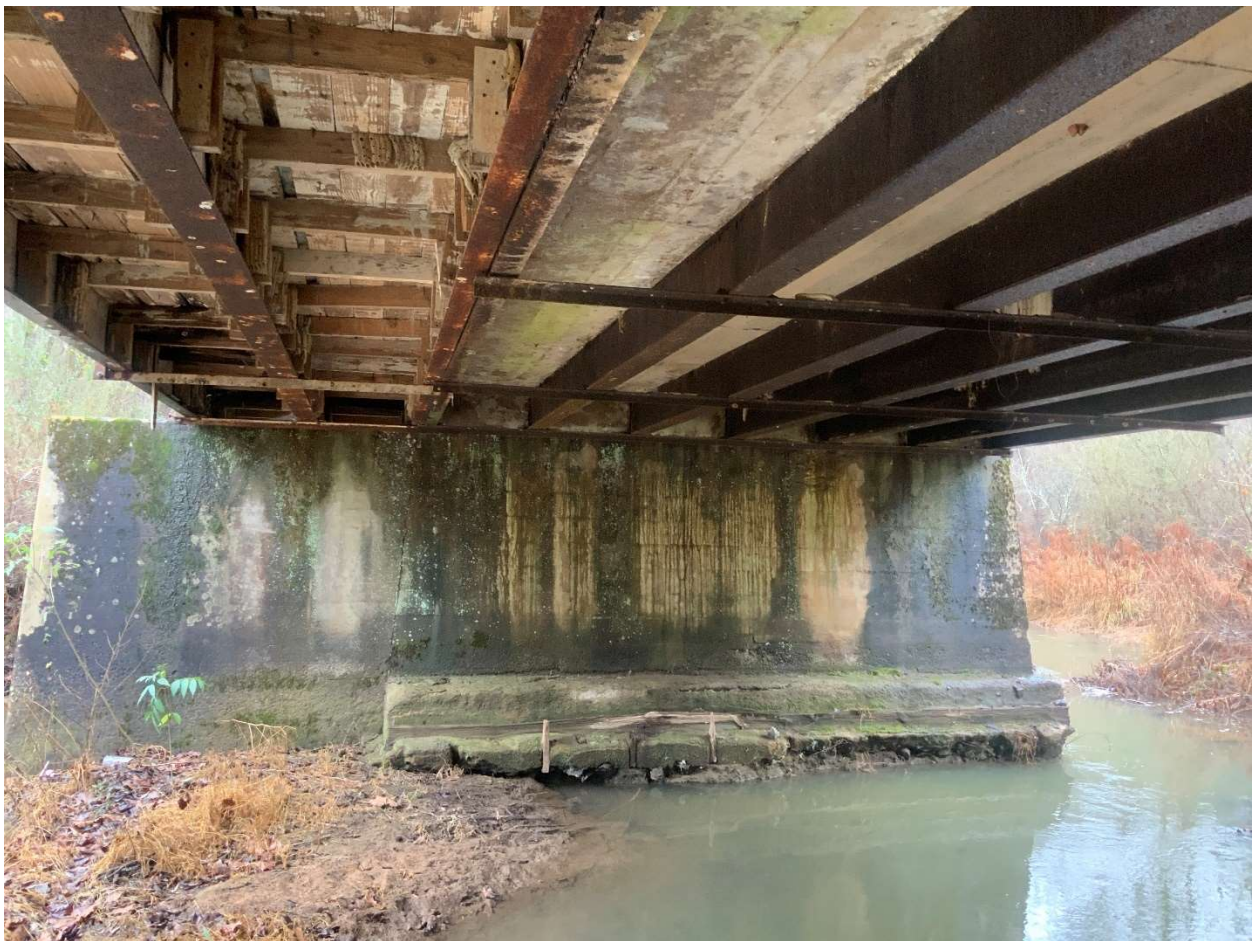
Figure 187 – Bridge 233-5036-0 Pier Wall Scour (GDOT, 2021)
