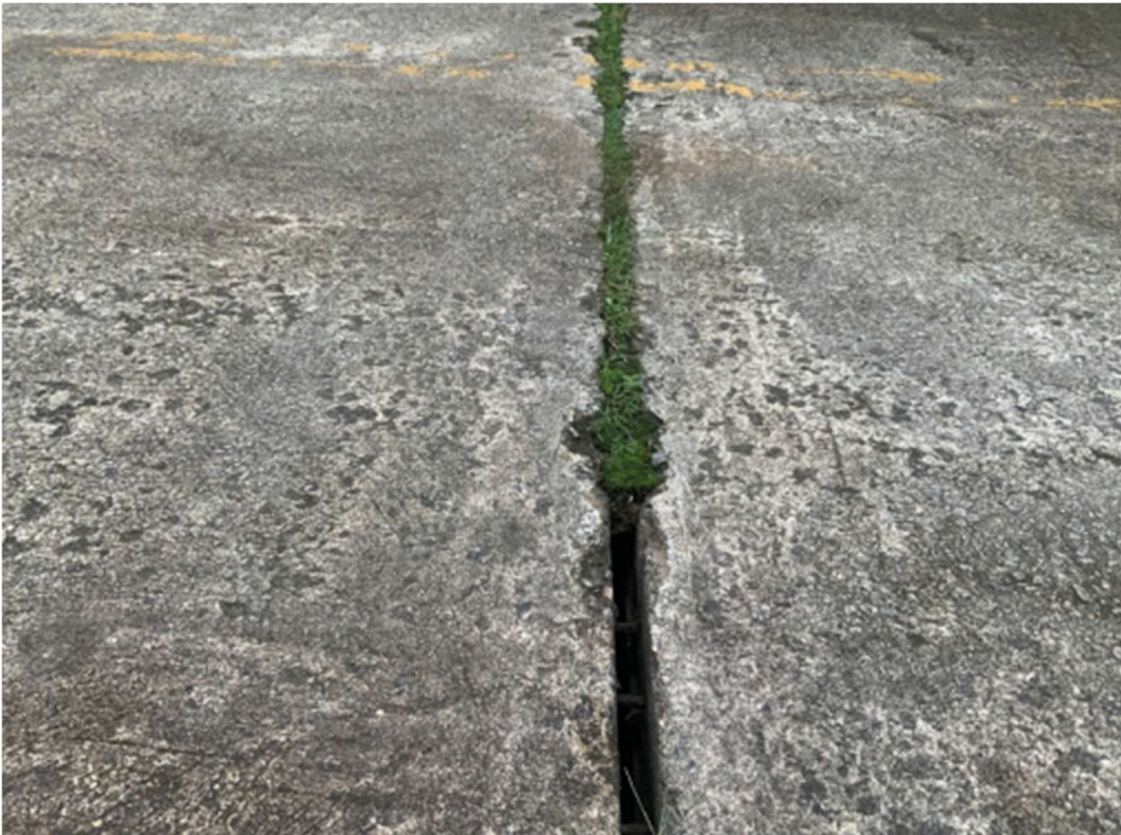
Figure 223 – Bridge 045-5018-0 Joint Condition 2016 (Top) vs 2021 (Bottom)
