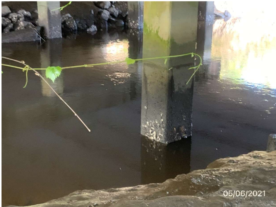
Figure 294 – Bridge 039-0051-0 Typical Prestressed Concrete Pile Cracking (GDOT, 2021)
