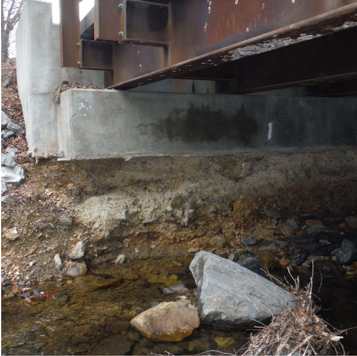
Figure 209 – Bridge 213-5044-0 Abutment One Scour (GDOT, 2018)
