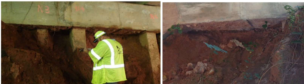
Figure 152 – Erosion at Abutment 5 on Bridge 241-0016-0 (GDOT, 2020)
