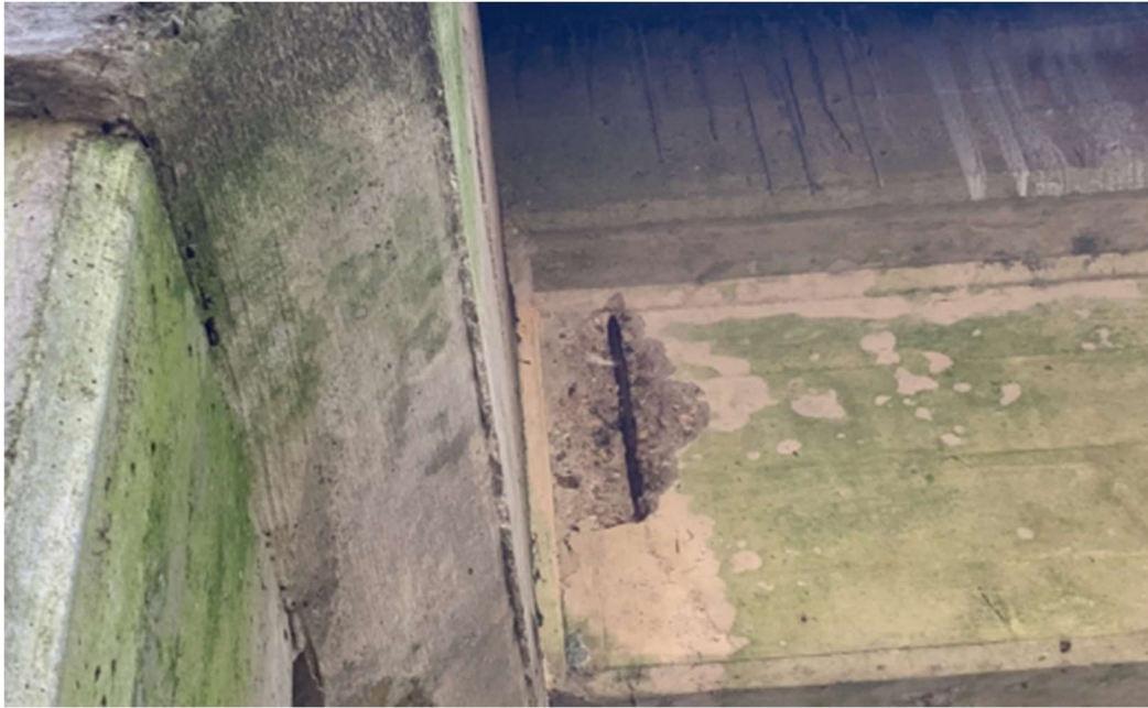
Figure 99 – Bridge 295-0041-0 Reinforced Concrete Girder Spalling (GDOT, 2021)
