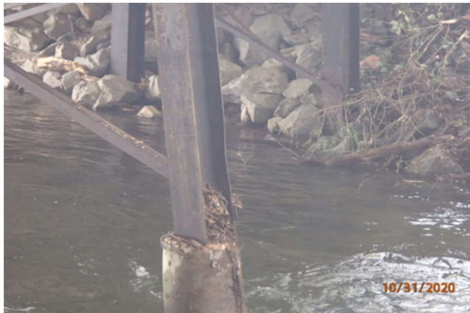
Figure 160 – Minor Bending in Steel Pile in Bridge 187-0006-0 (GDOT, 2020)
