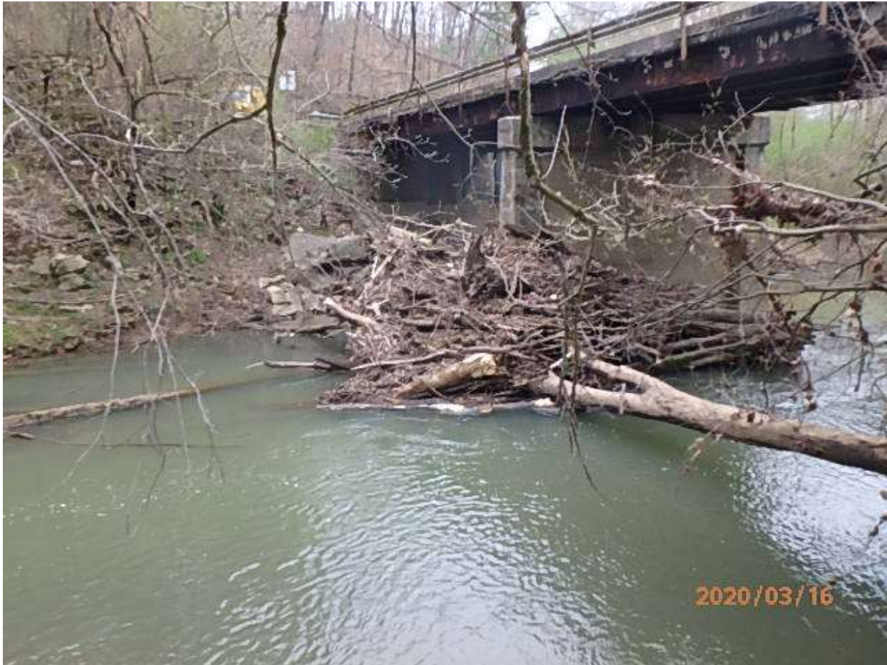
Figure 168 – Bridge 055-5030 Drift at Bent 3 2012 (Top) vs 2020 (Middle & Bottom)
