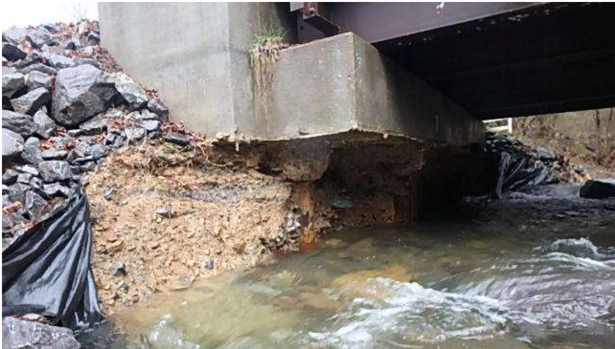
Figure 210 – Bridge 213-5044-0 Abutment One Scour (GDOT, 2020)
