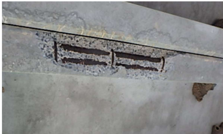
Figure 84 – Bridge 313-5028-0 Reinforced Concrete Girder Spalling 2014 (Top) vs 2020 (Bottom)
