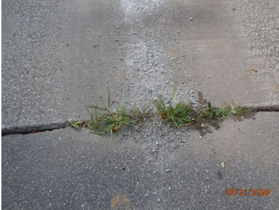
Figure 227 – Bridge 241-5051-0 Joint Condition (GDOT, 2020)
