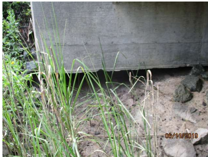
Figure 295- Bridge 039-5029-0 Abutment Undermining (GDOT, 2019)
