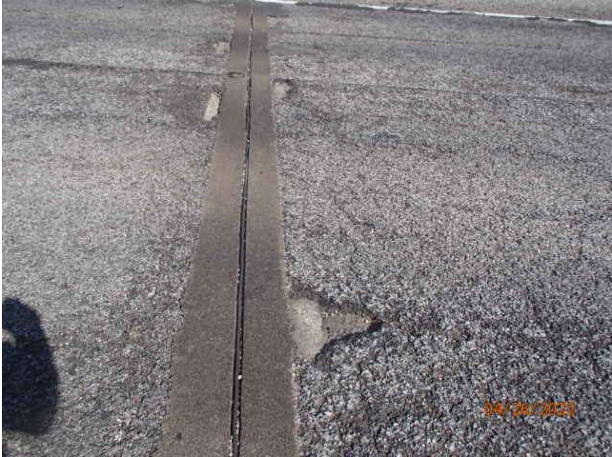
Figure 272 – Bridge 137-0029-0 Protective Wearing Surface at Bent 2 Condition 2014 (Top) vs 2022 (Bottom)
