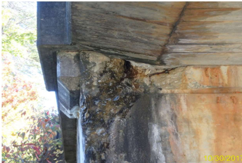
Figure 72: Concrete Spalling and Exposed Rebar in Abutment 1 of Bridge 241-5024-0, 2017
