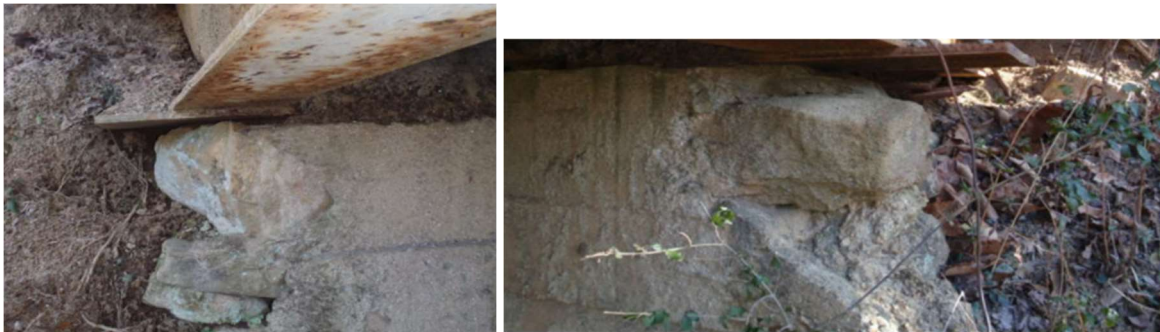
Figure 42: Reinforced Concrete Abutment Area Loss (GDOT, 2021)
