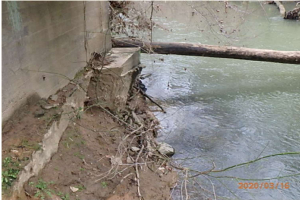
Figure 83 – Scour at Reinforced Concrete Pier Wall on Bridge 055-5030-0 (GDOT, 2020)
