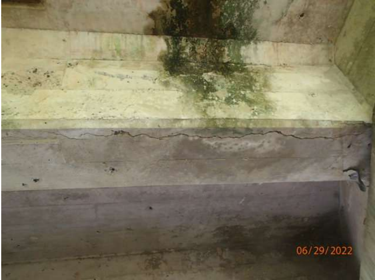
Figure 247 – Bridge 241-5036-0 Span 3 Beam 1 Concrete Cracking 2014 (Top) vs 2022 (Bottom)
