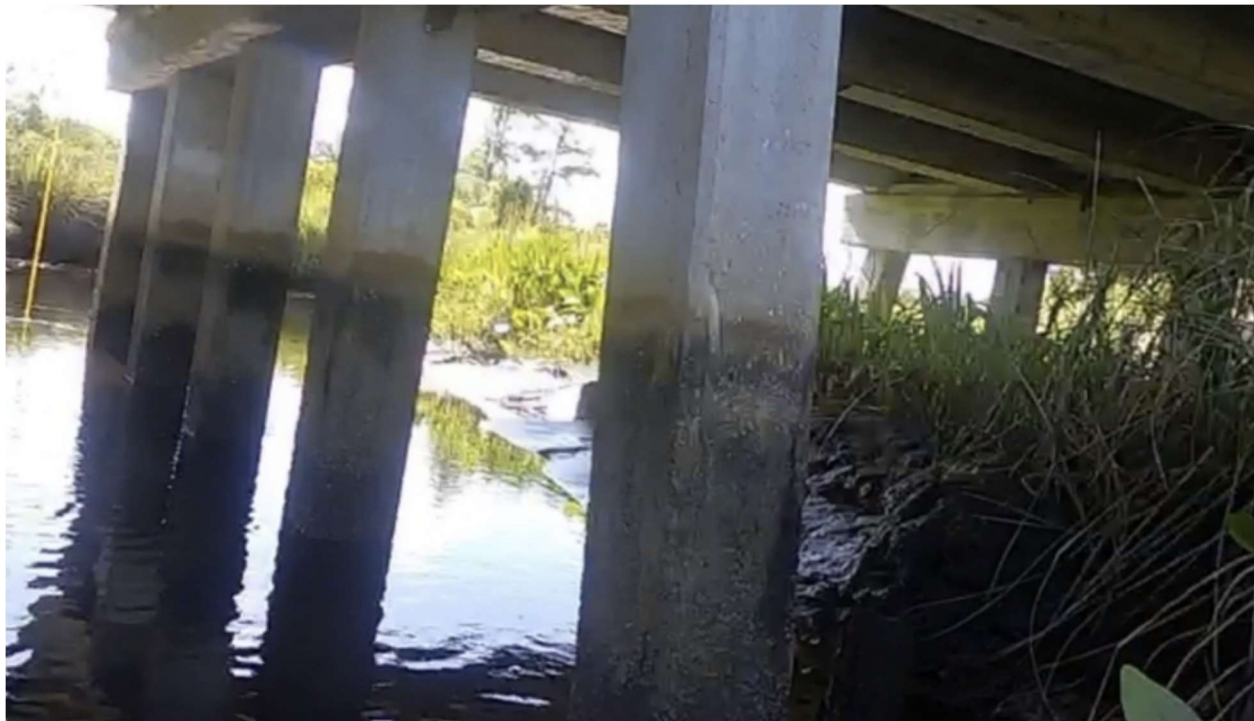
Figure 285 – Bridge 039-0001-0 Prestressed Concrete Piles Typical Condition (GDOT, 2021)
