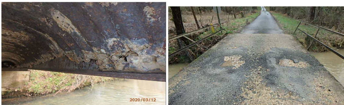
Figure 67: Bridge 055-5041-0 Deck Bottom (Right) and Top (Right) Deterioration (GDOT, 2020).
