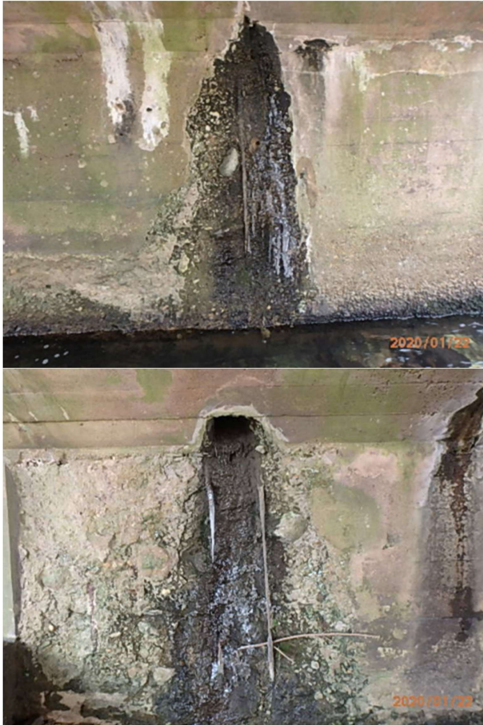
Figure 197 – Bridge 213-0017-0 Pier Wall 2 Abrasion Area (GDOT, 2020)
