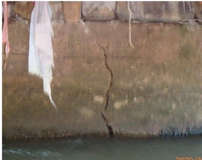
Figure 54: Bridge 055-5045-0 Abutment 1 Settlement Crack (GDOT, 2020)
