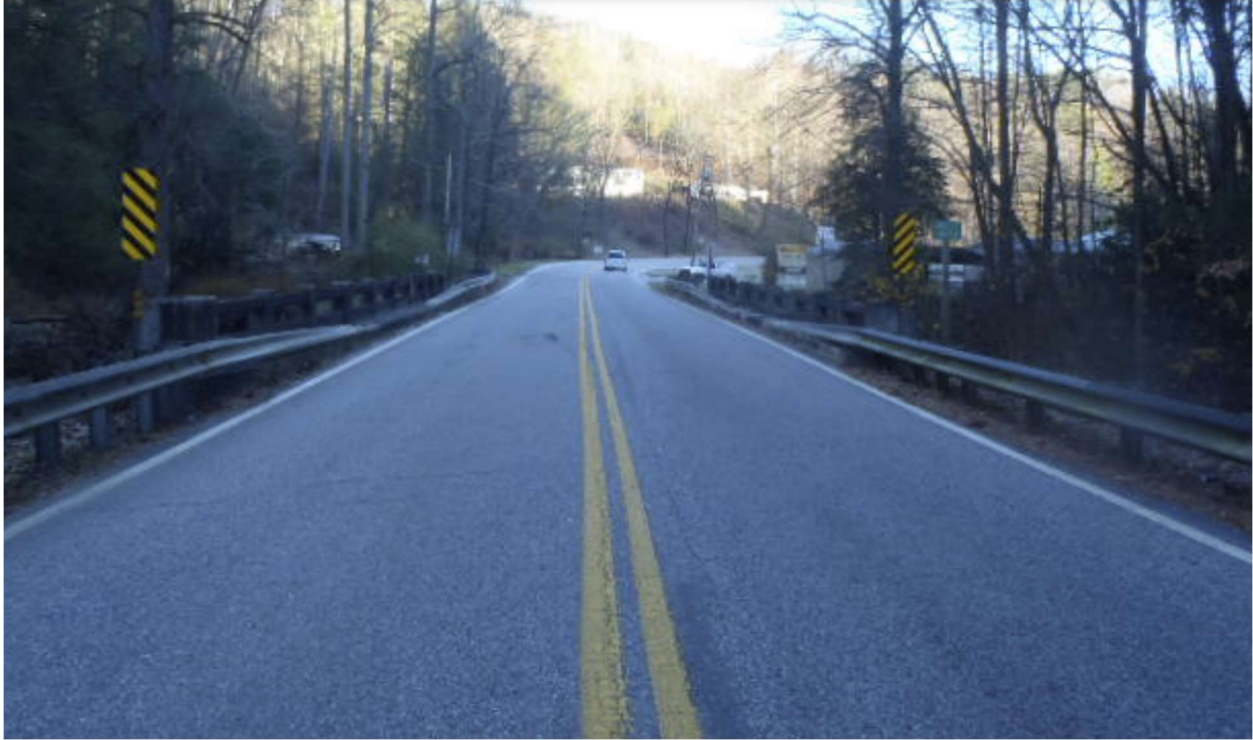
Figure 280 – Bridge 187-0007-0 Deck Condition 2015 (Top) vs 2021 (Bottom)
