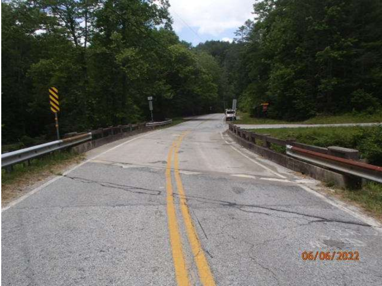
Figure 252 – Bridge 241-0018-0 Deck Condition 2014 (Top) vs 2022 (Bottom)
