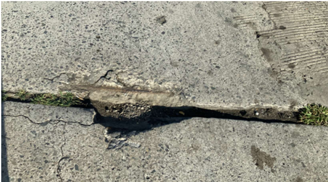
Figure 127 – Bridge 083-0012-0 Joint Failure (GDOT, 2017)
