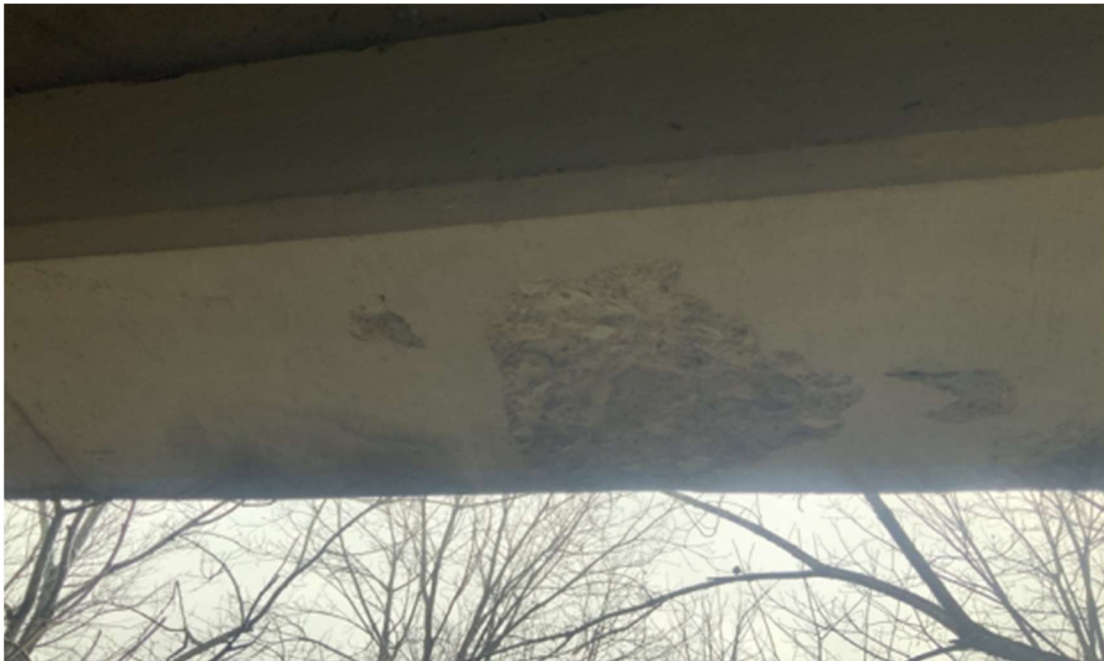
Figure 95 – Bridge 295-0039-0 Concrete Spalling (GDOT, 2021)
