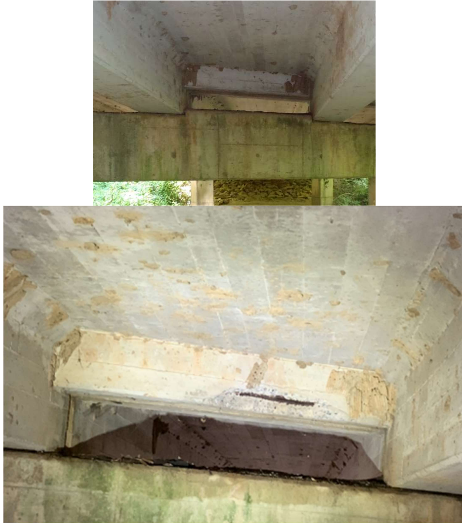
Figure 263 – Bridge 157-5046-0 Reinforced Concrete Top Flange Concrete Spall 2014 (Top) vs 2022 (Bottom)
