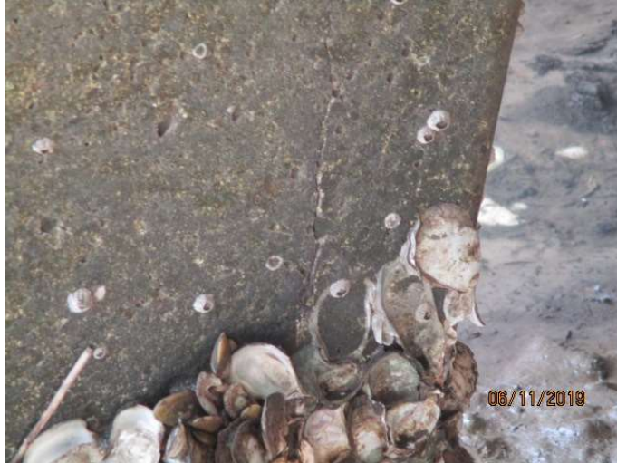
Figure 297- Bridge 039-5029-0 Pile Cracking (GDOT, 2019)
