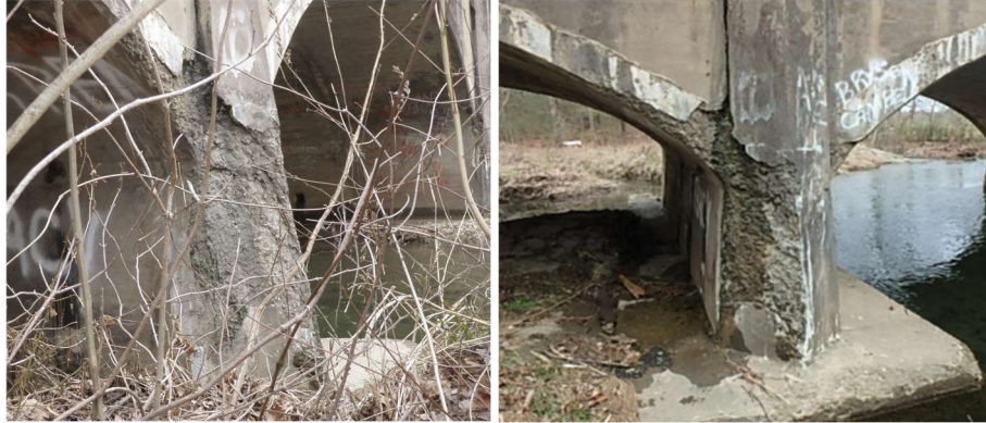
Figure 58: Progression of Pier Degradation 2014(Left) to 2020(Right)
