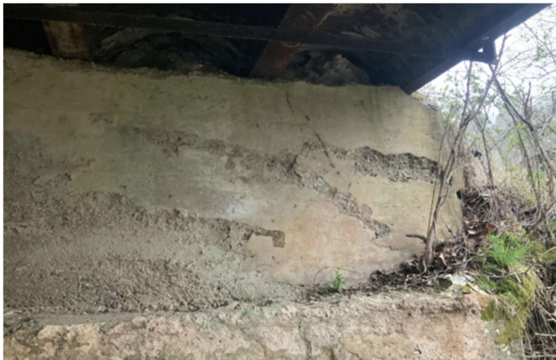
Figure 46: Spalling in Abutment 2 (GDOT, 2022)
