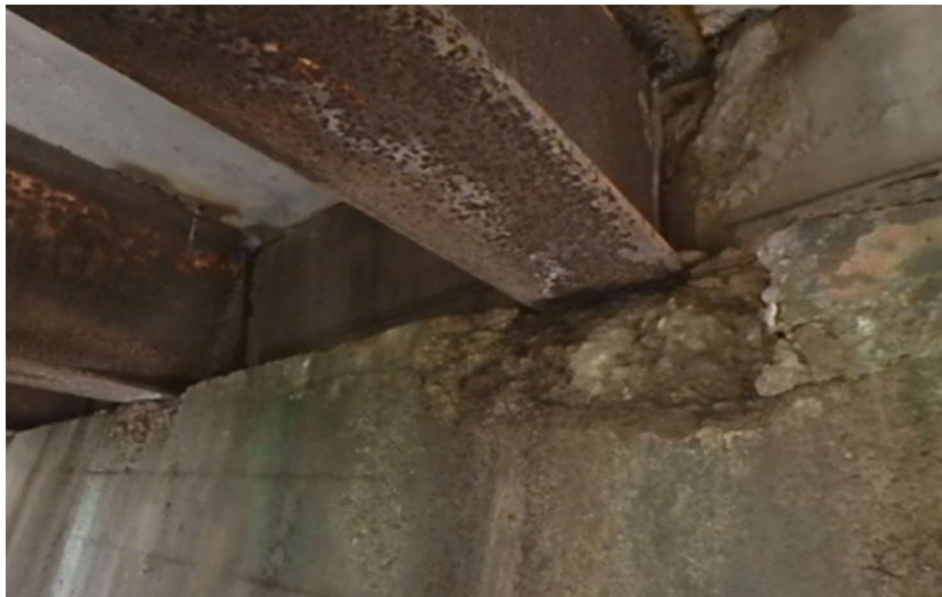
Figure 82 – Spalling in Reinforced Concrete Abutment on Bridge 055-5030-0 (GDOT, 2020)
