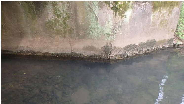
Figure 47: Undermining in Abutment 1 (GDOT, 2020)
