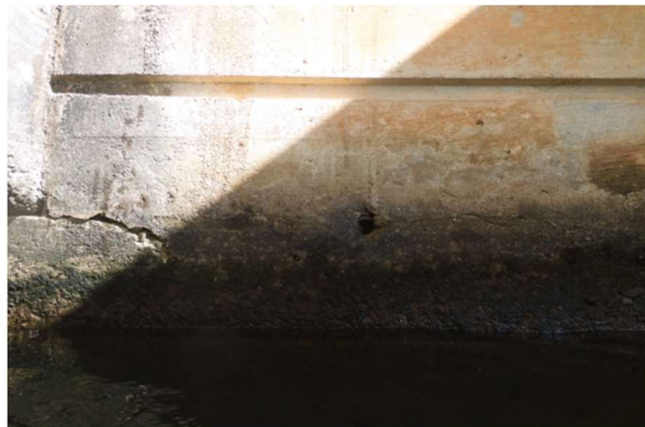
Figure 75: Honeycombing Patch in Abutment 1 of Bridge 241-5024-0 (GDOT, 2022)
