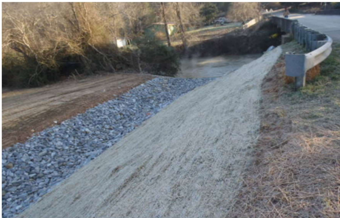
Figure 174 – Bridge 291-5035-0 Erosion, 2015 (Top) and Erosion Repair, 2016 (Bottom)
