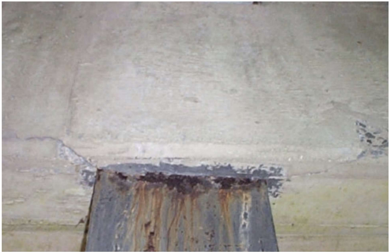
Figure 163 – Bridge 055-5001-0 Steel Pile Connection 2016 (Top) vs 2022 (Bottom)
