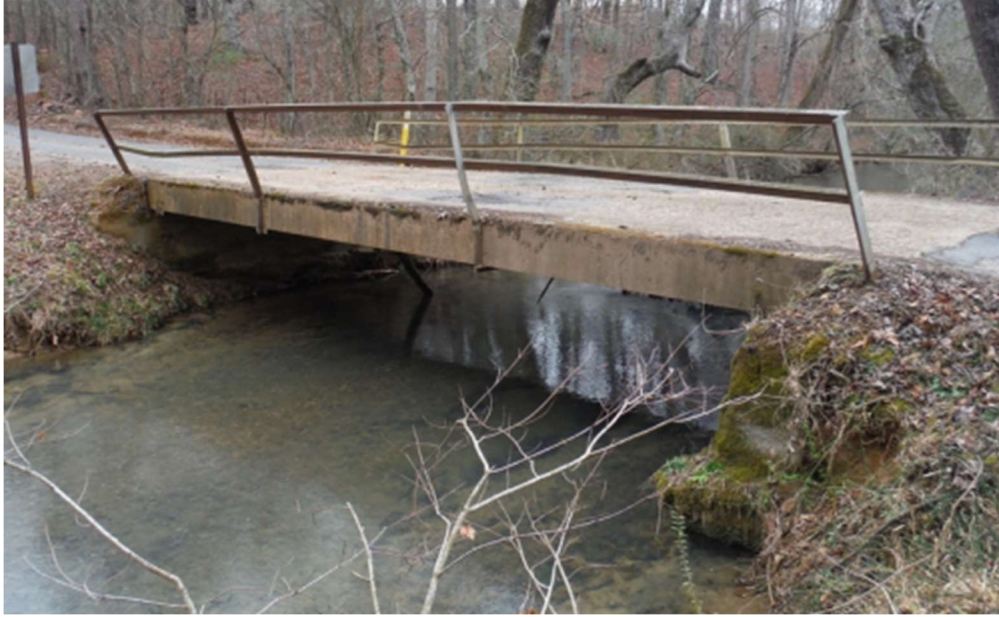
Figure 68: Scour at Abutment 1 (GDOT, 2014)
