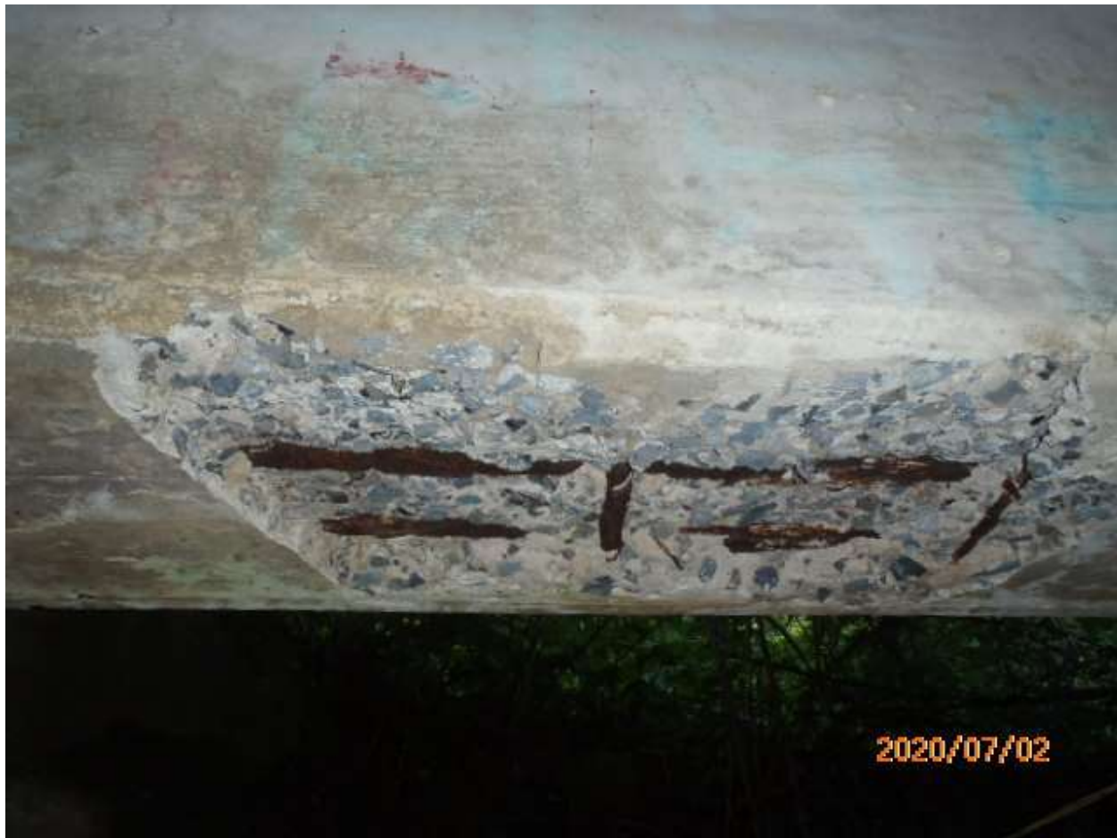
Figure 248 – Bridge 241-5036-0 Span 1 Beam 1 Concrete Spalling 2014 (Top) vs 2020 (Bottom)
