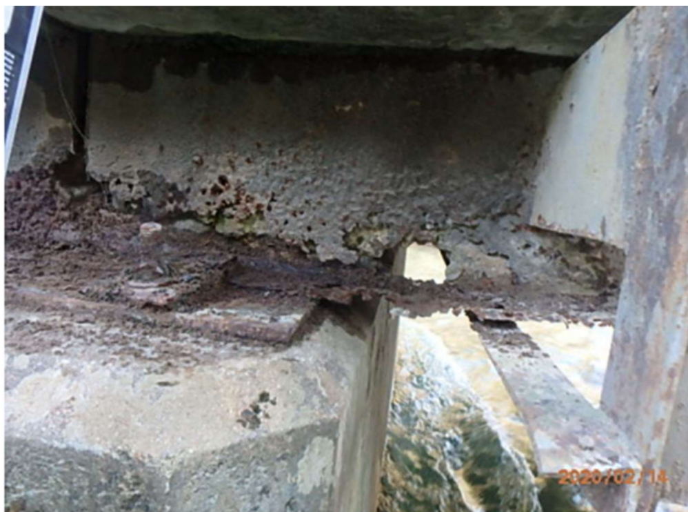
Figure 194 – Bridge 213-0048-0 Steel Girder Corrosion (GDOT, 2020)
