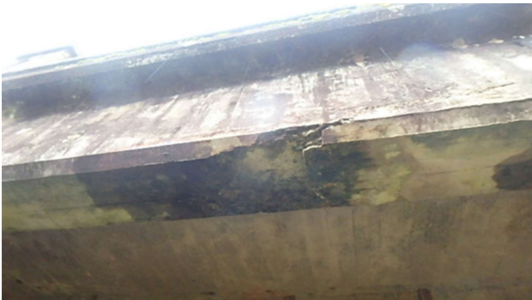
Figure 103 – Bridge 055-5037-0 Reinforced Concrete Girder Spalling (GDOT, 2020)
