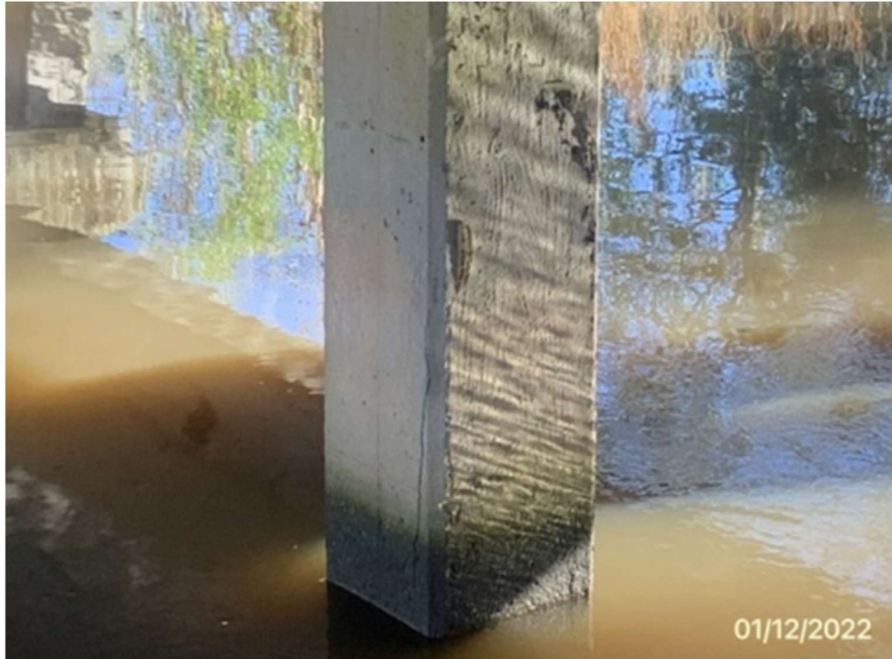
Figure 300 – Bridge 170-0006-0 Typical Cracking in PSC Piles (GDOT, 2022)
