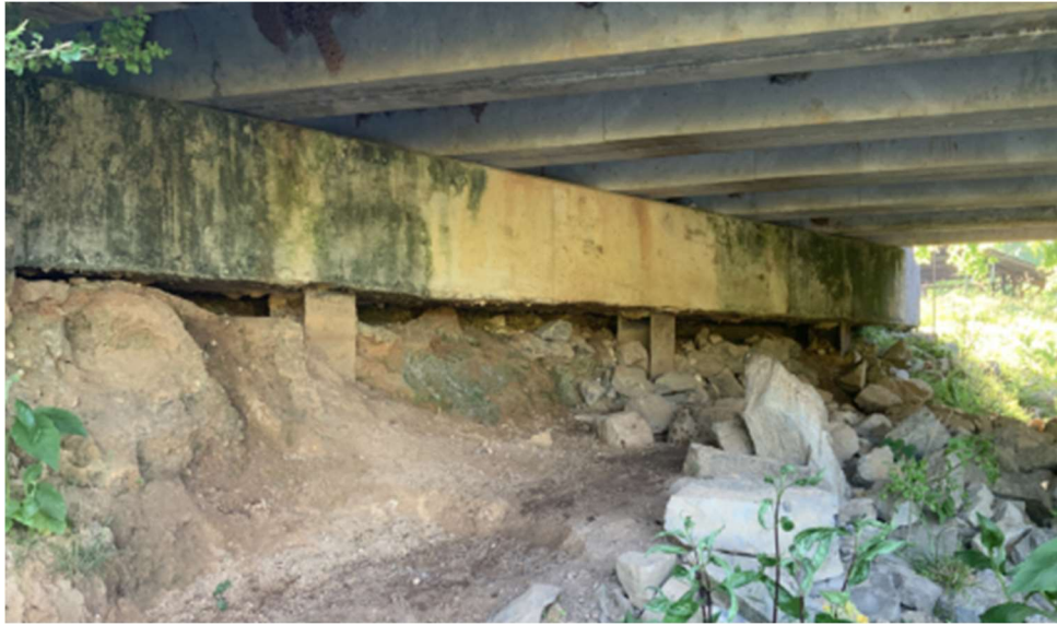
Figure 144 – Bridge 313-5028-0 Abutment 3 Undermining (GDOT, 2022)
