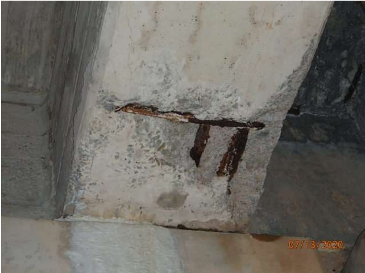
Figure 262 – Bridge 241-0016-0 Beam 9 Concrete Spalling 2016 (Top) vs 2020 (Bottom)
