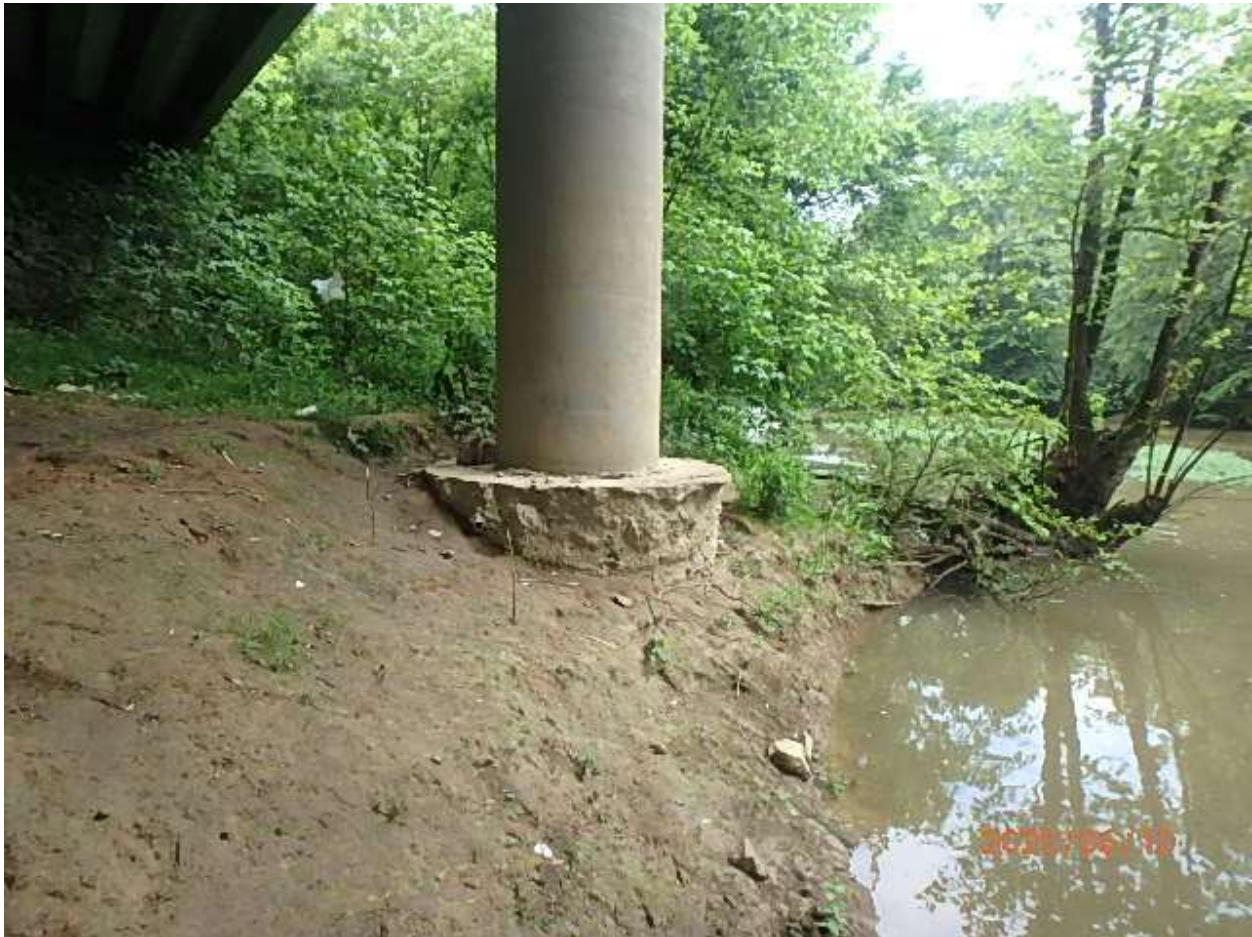
Figure 203 – Bridge 313-5083-0 Bent 2 Scour (GDOT, 2020)
