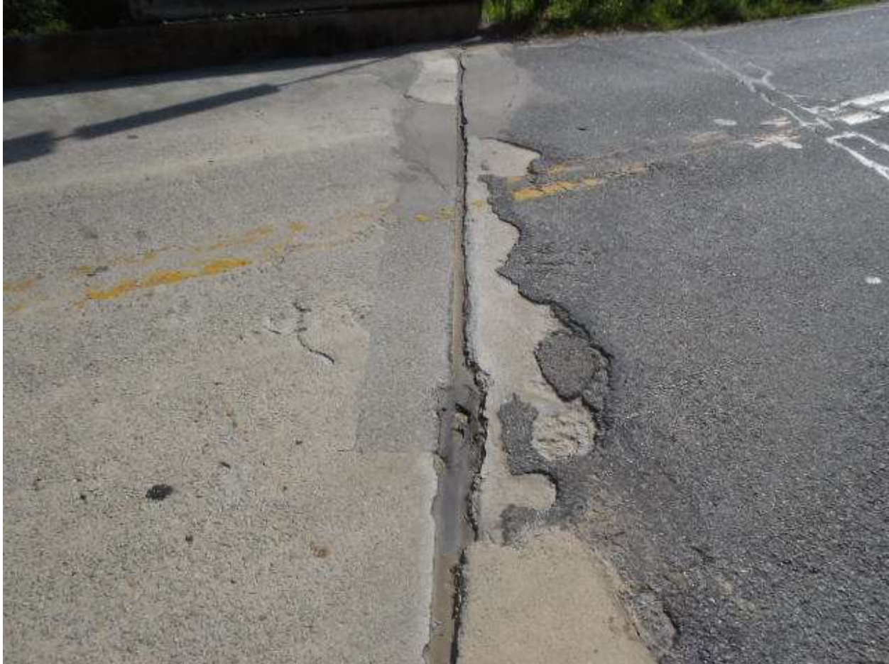
Figure 253 – Bridge 241-0018-0 Bridge Deck Condition 2014 (Top) vs 2022 (Bottom)
