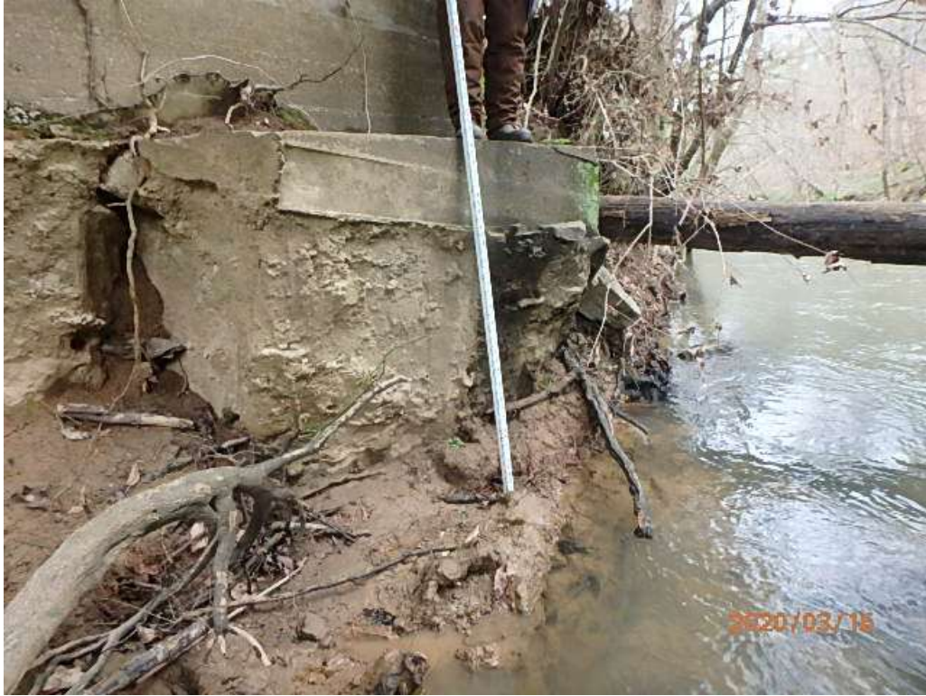
Figure 169 – Bridge 055-5030-0 Bent 2 Scour (GDOT, 2020)
