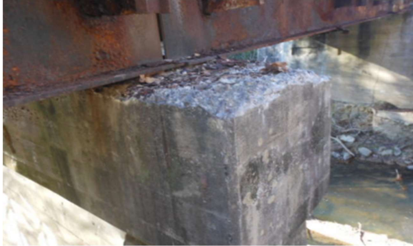
Figure 81 – Reinforced Concrete Pile Cap Wear on Bridge 055-5030-0 (GDOT, 2017)
