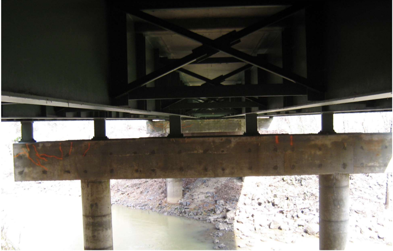
Figure 141 – Bridge 213-0008-0 Pier Cap Concrete Cracking (GDOT, 2022)
