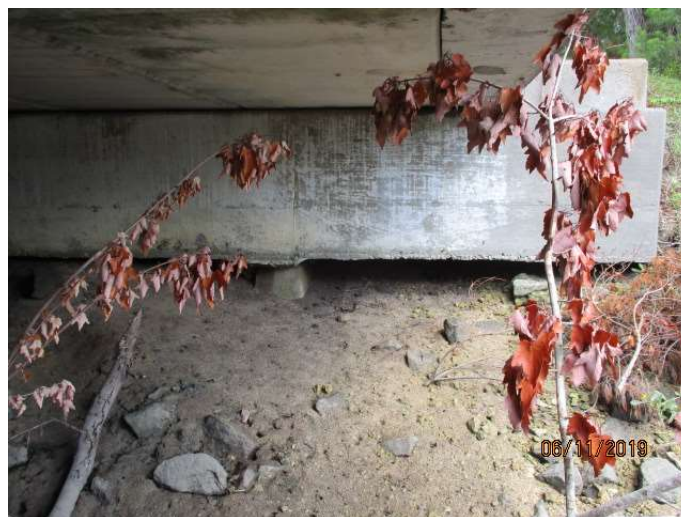
Figure 296- Bridge 039-5029-0 Abutment Undermining (GDOT, 2019)
