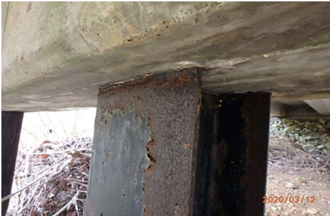
Figure 162 – Bridge 055-5001-0 Typical Steel Pile Section Loss (GDOT, 2020)
