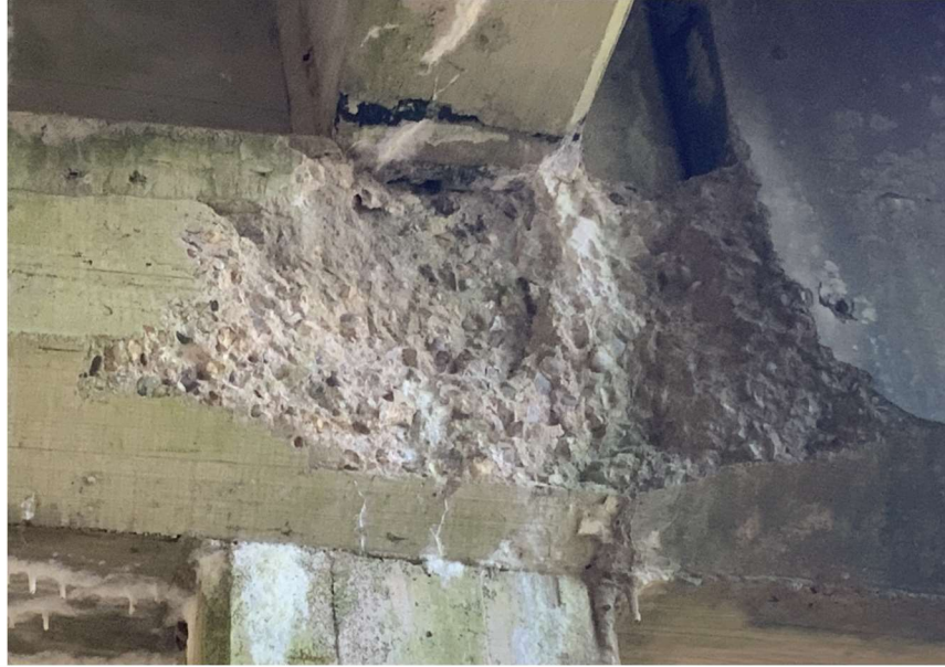
Figure 121 – Bridge 295-5012-0 Reinforced Concrete Pier Cap Spalling (GDOT, 2021)
