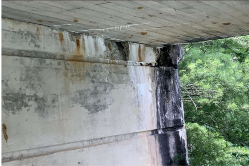
Figure 76: Concrete Spalling in Abutment 1 of Bridge 241-5024-0 (GDOT, 2022)
