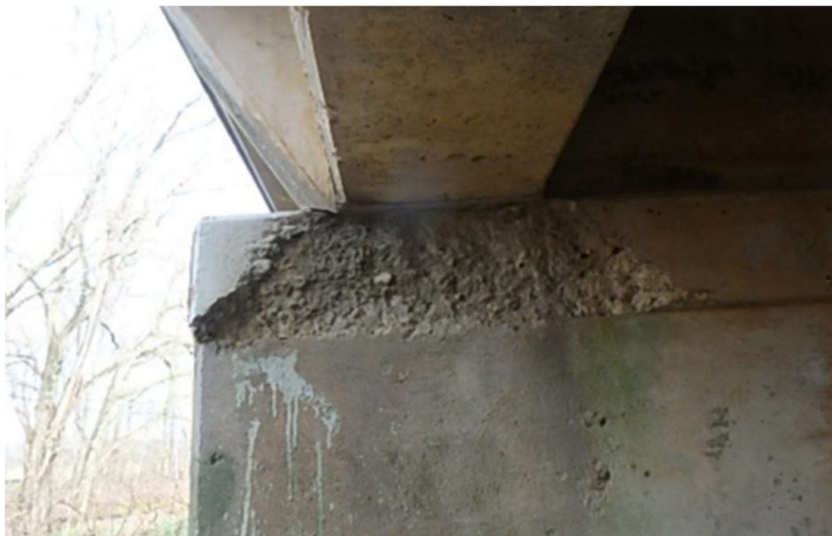
Figure 198 – Bridge 213-0017-0 Bent Cap 4 Spall 2016 (Top) vs 2020 (Bottom)
