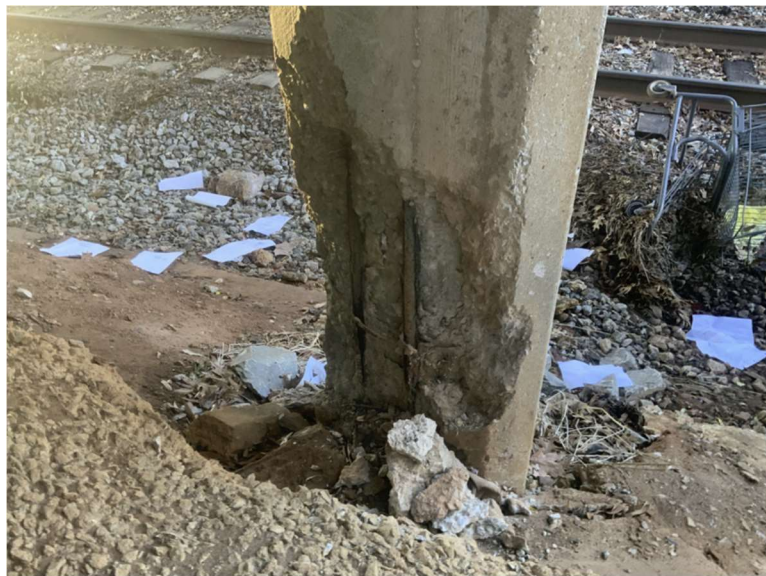
Figure 186 – Bridge 233-055-0 Column 3-2 2016 (Top) vs 2022 (Bottom)
