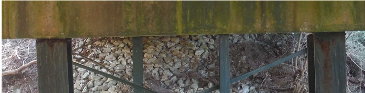
Figure 176 – Bridge 111-5002-0 Steel Pile Condition at Bent 2 (GDOT, 2016)
