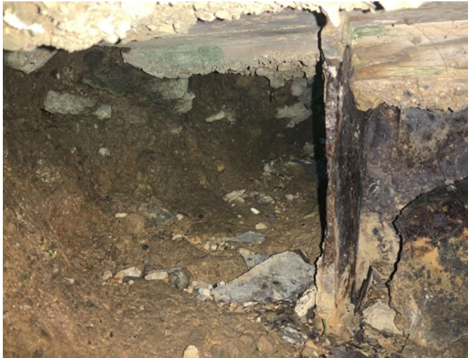
Figure 145 – Bridge 313-5028-0 Abutment 3 Pile 1 Section Loss (GDOT, 2022)
