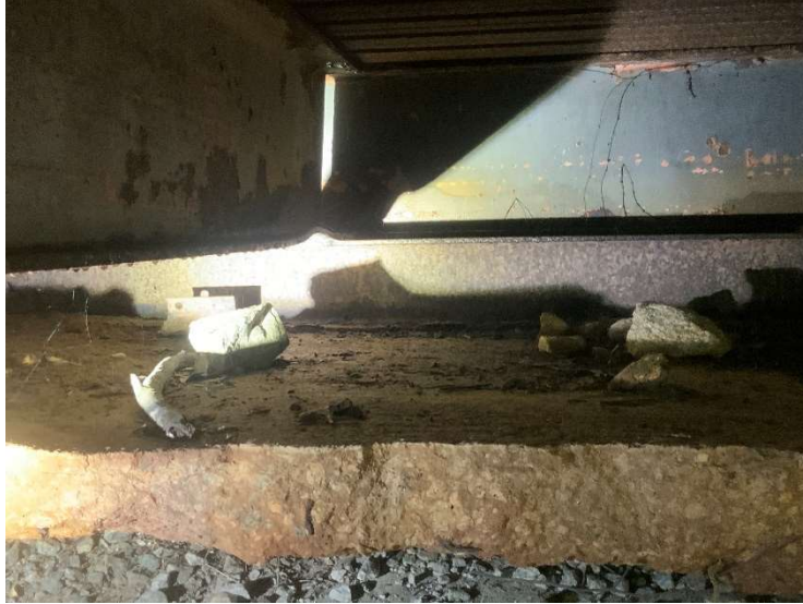
Figure 235 – Bridge 297-5062-0 Steel Abutment Condition 2013 (Top) vs 2021 (Bottom)
