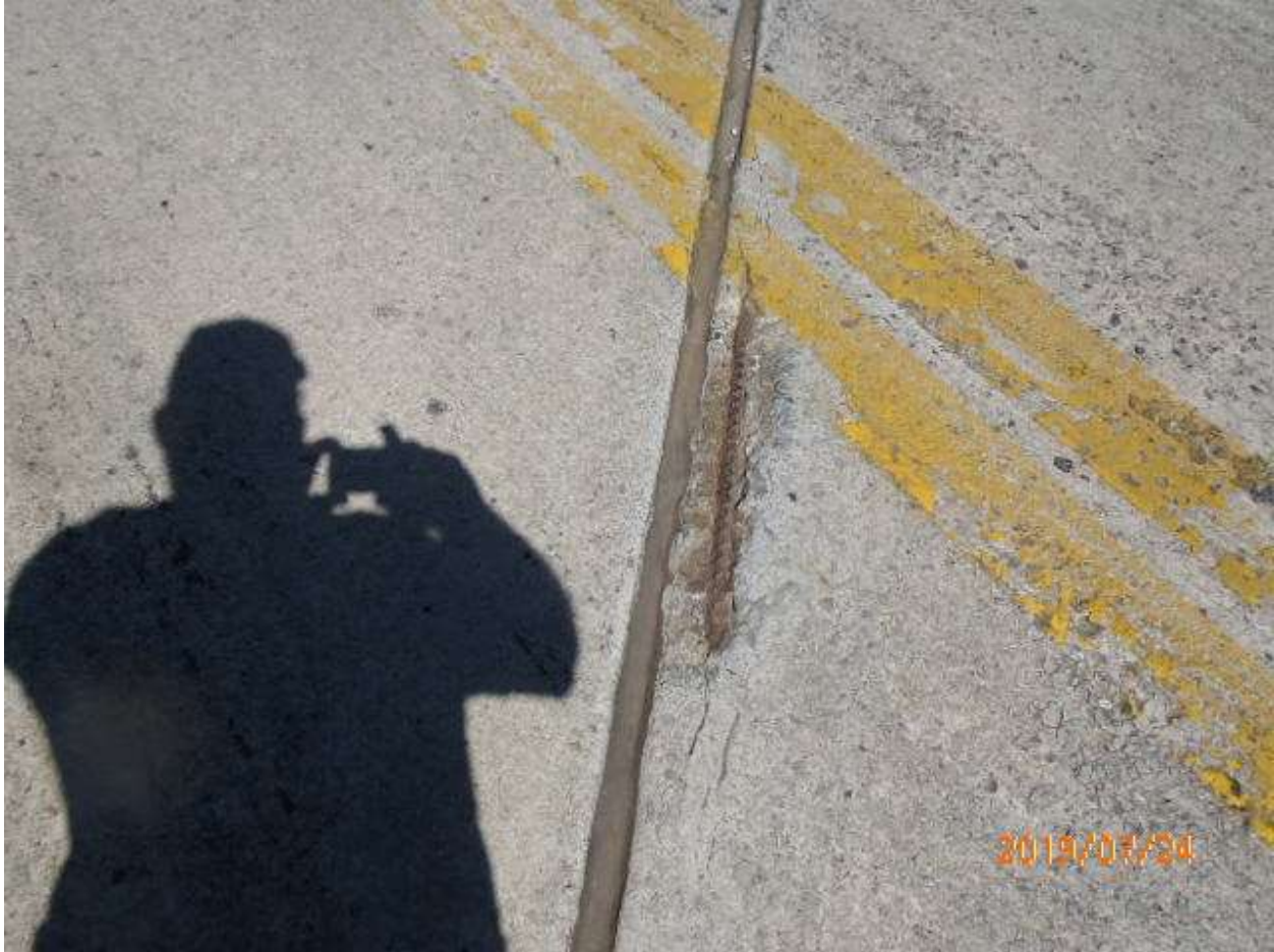
Figure 242 – Deck Spall 2014 (Top) vs 2017 (Middle) vs 2019 (Bottom)
