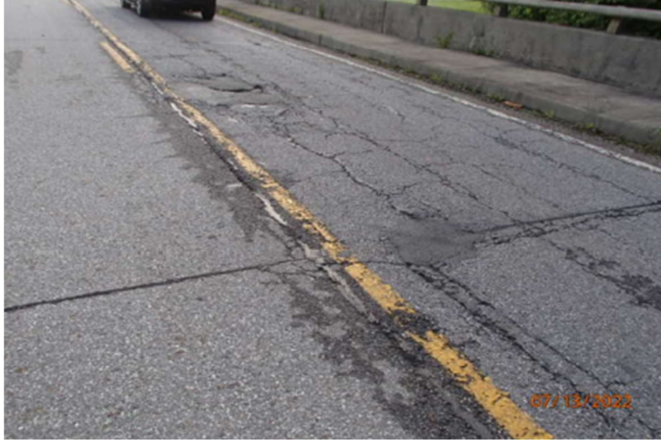
Figure 260 – Bridge 241-0016-0 Typical Deck Cracking (GDOT, 2022)
