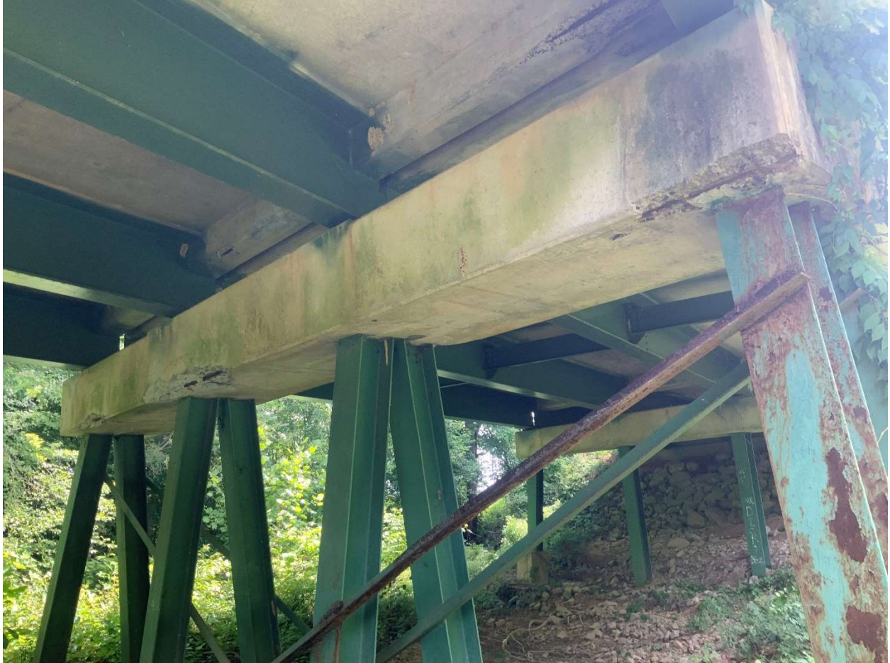
Figure 138 – Bridge 313-0004-0 Reinforced Concrete Pier Cap Spalling, 2022
