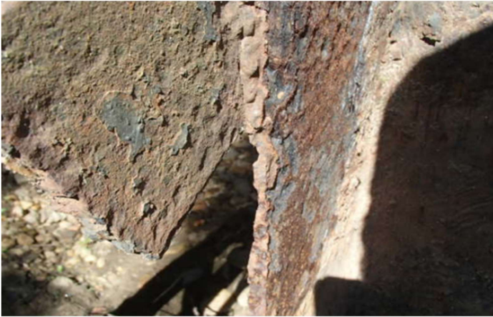
Figure 151 – Bridge 241-0016-0 Steel Pile Section Loss at Ground Level (GDOT, 2022)
