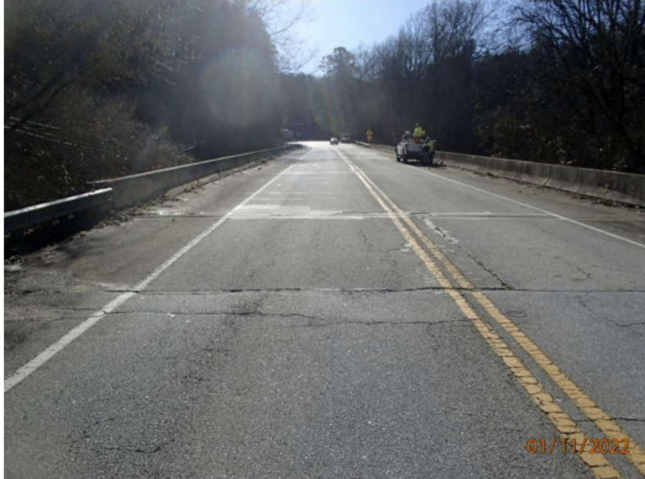
Figure 279 – Bridge 187-0011-0 Deck Condition 2016 (Top) vs 2022 (Bottom)
