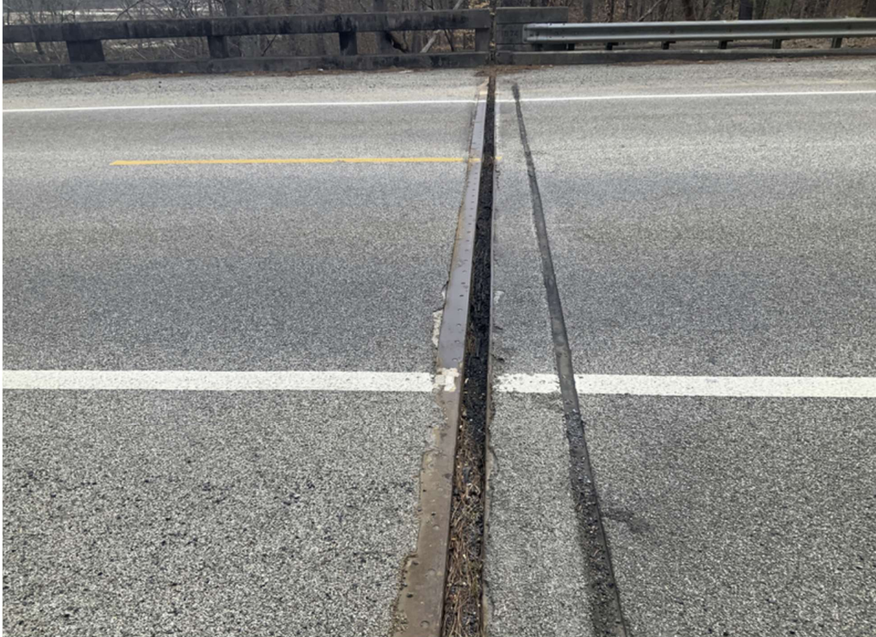
Figure 221 – Bridge 213-0008-0 Compression Joint 2015 (Top) vs 2018 (Middle) vs 2022 (Bottom)
