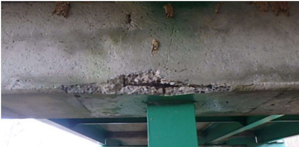
Figure 135 – Bridge 213-0001-0 Reinforced Concrete Pier Cap Spalling with Rebar Section Loss (GDOT, 2020)
