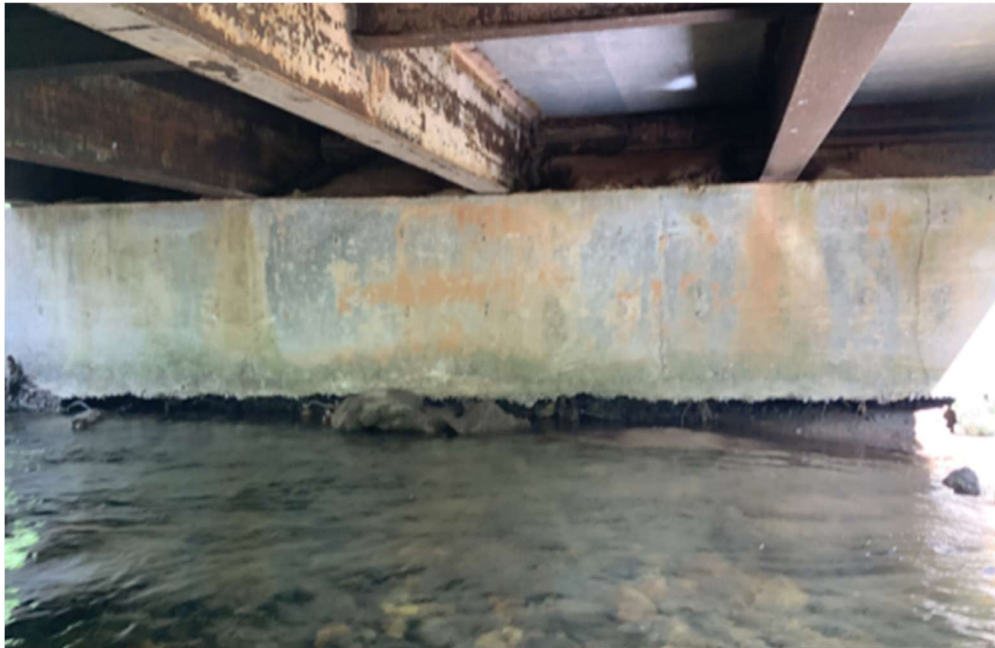
Figure 214 – Bridge 123-5024-0 Abutment 2 Undermining (GDOT, 2021)
