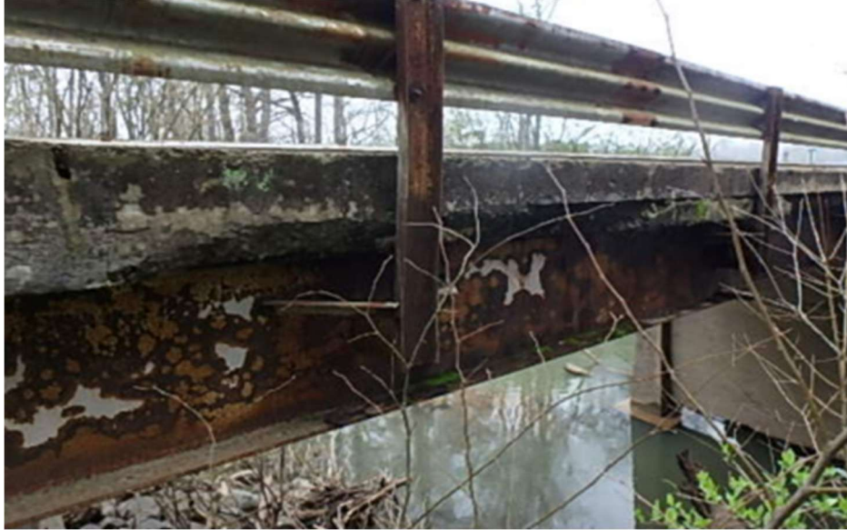
Figure 80 – Bridge 055-5030-0 Wide Flange 100% Section Loss (GDOT, 2022)
