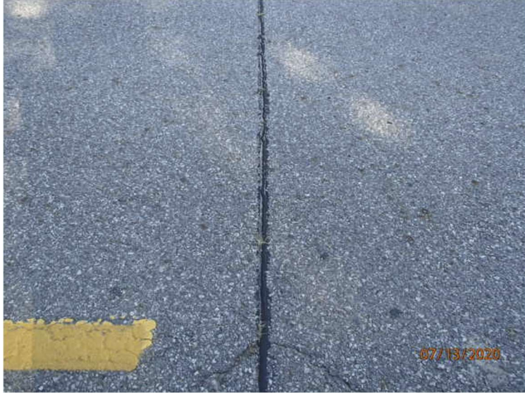
Figure 154 – Bridge 241-0016-0 Failing Joint (GDOT, 2020)
