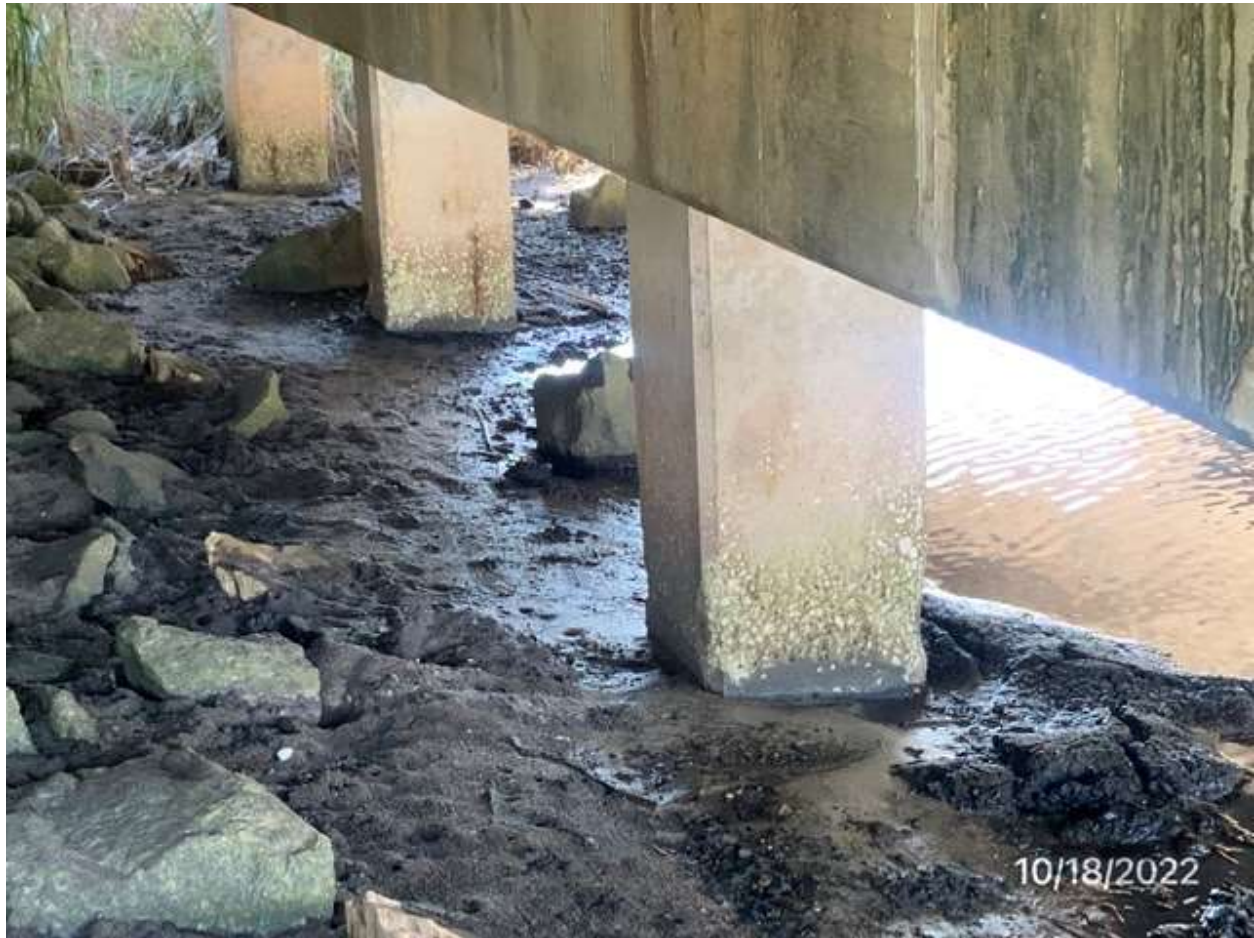
Figure 291 – Bridge 127-0029-0 Typical Pile Cracking (GDOT, 2022)
