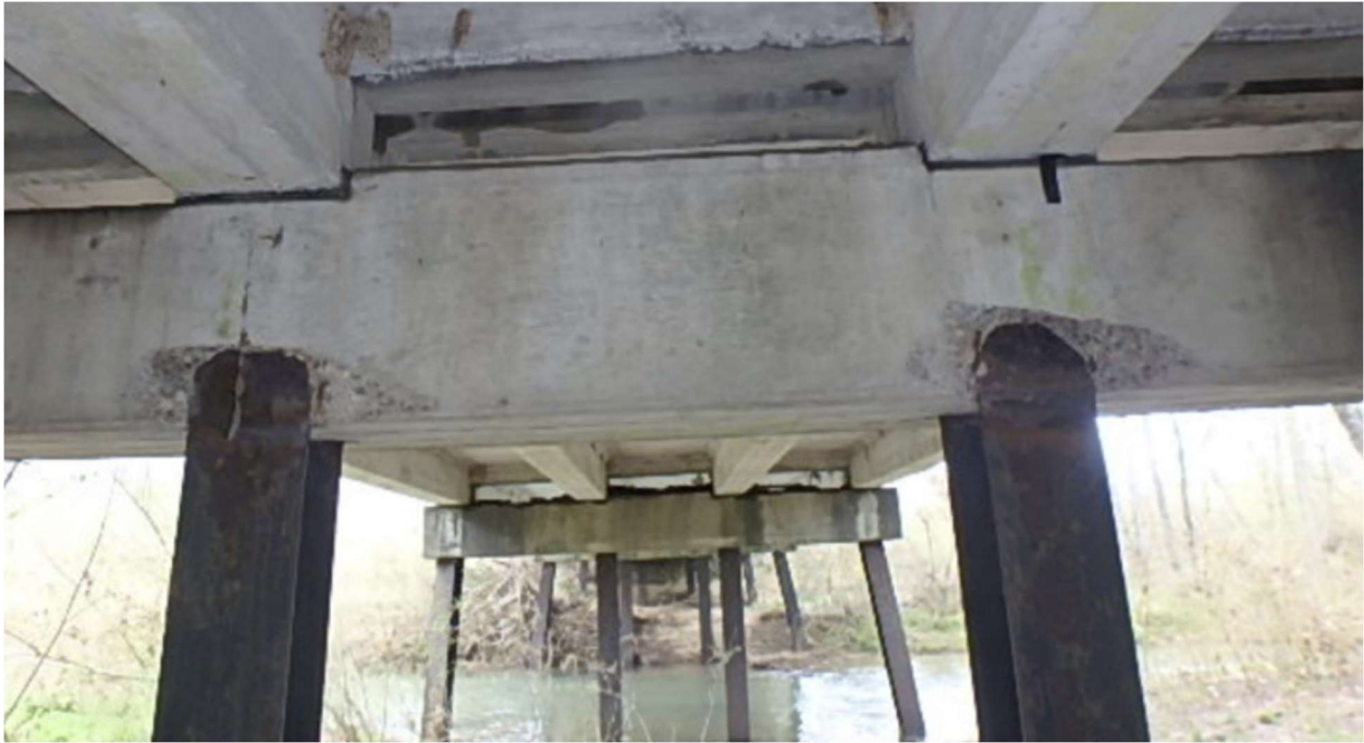
Figure 164 – Bridge 055-5001-0 Steel Pile Connection 2016 (Top & Middle) vs 2022 (Bottom)
