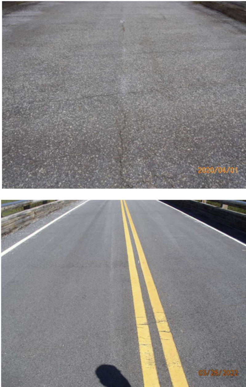
Figure 278 – Bridge 137-5064-0 Deck Condition 2020 (Top)) vs 2022 (Bottom)
