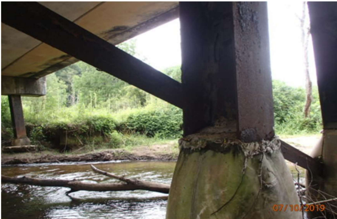
Figure 170 – Bridge 291-5026-0 Steel Pile Condition (GDOT, 2019)
