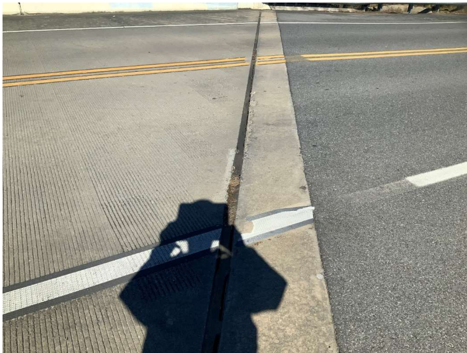
Figure 218 – Bridge 213-5045-0 Failed Compression Joint (GDOT, 2022)
