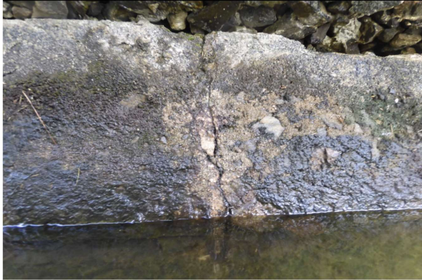
Figure 74: Concrete Cracking and Honeycombing in Abutment 1 of Bridge 241-5024-0 (GDOT, 2022)
