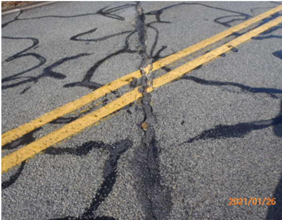
Figure 226 – Bridge 257-0001-0 Typical Joint Condition (GDOT, 2021)
