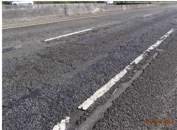
Figure 277 – Bridge 137-0028-0 Deck Condition 2016 (Top) vs 2018 (Middle) vs 2022 (Bottom)
