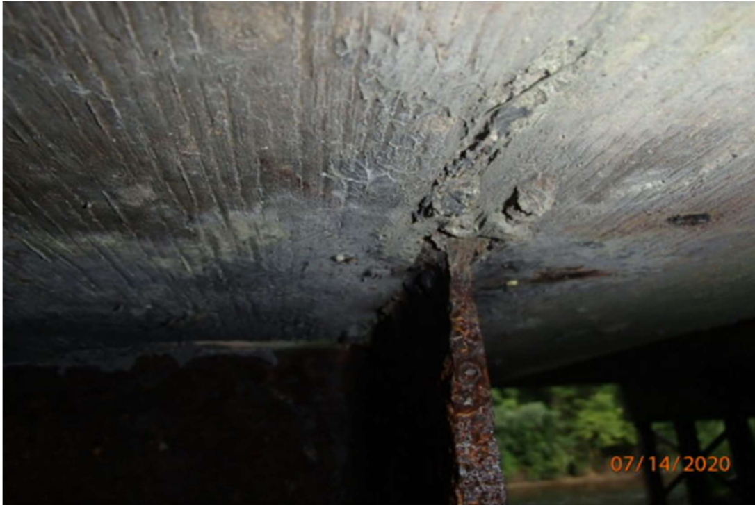
Figure 156 – Bridge 241-0016-0 Steel Pile Section Loss at Deck (GDOT, 2020)
