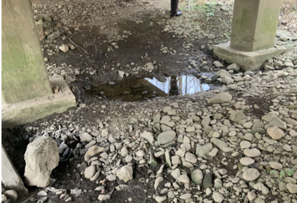
Figure 196 – Bridge 213-0017-0 Scouring at Bent 4, 2022
