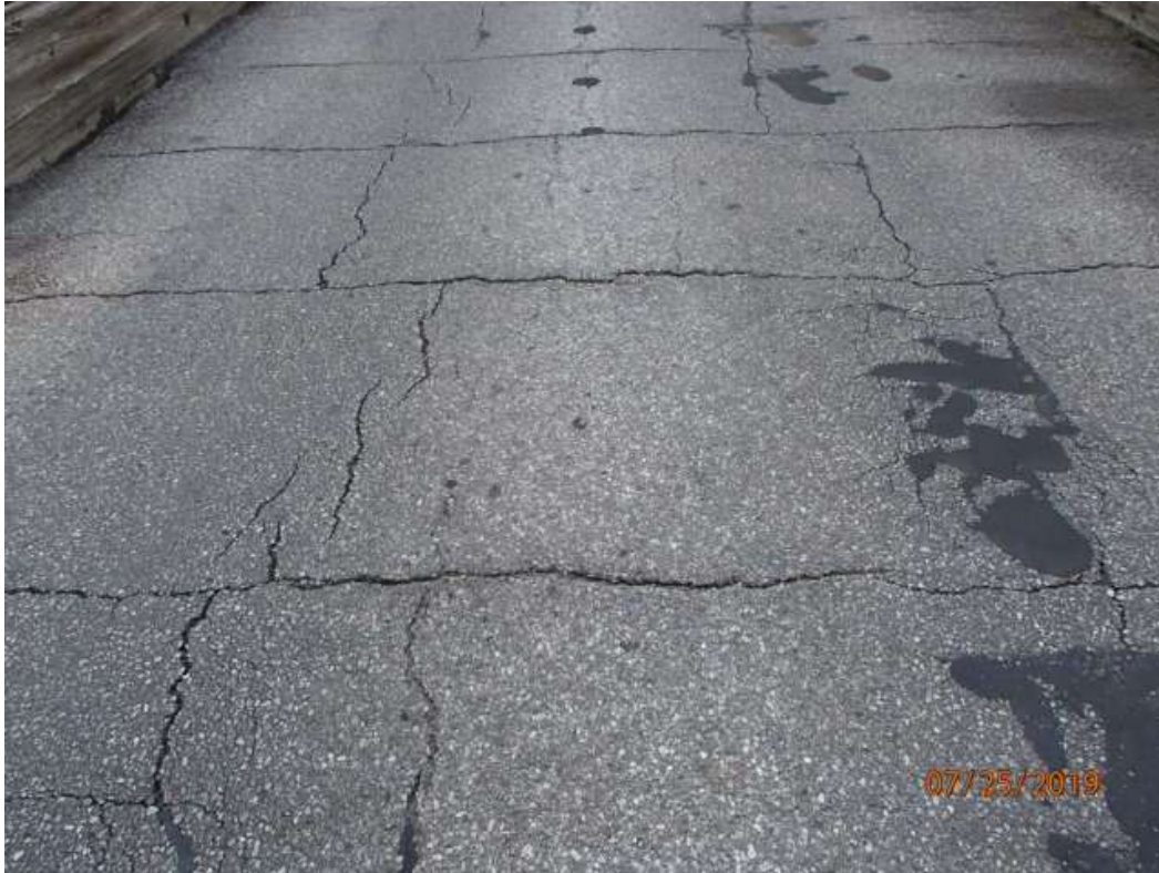
Figure 276 – Bridge 291-5048-0 Asphalt Cracking (GDOT, 2019)
