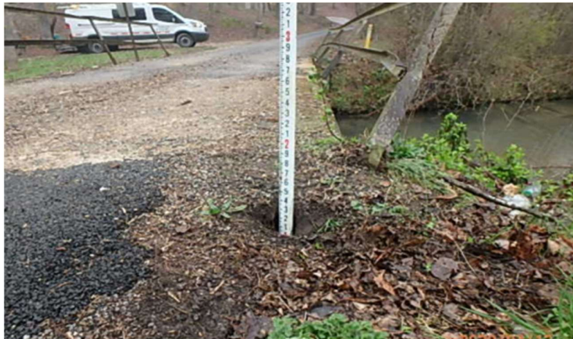
Figure 69: Void at Abutment 1 (GDOT, 2020)
