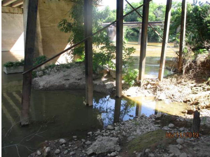
Figure 213 – Bridge 129-0009-0 Scour at Bent 15 2015 (Top) vs 2019 (Bottom)
