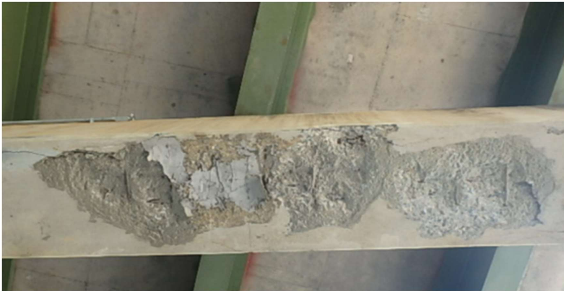
Figure 125 – Bridge 083-0012-0 Reinforced Concrete Pier Cap Failed Spall Repair (GDOT, 2019)
