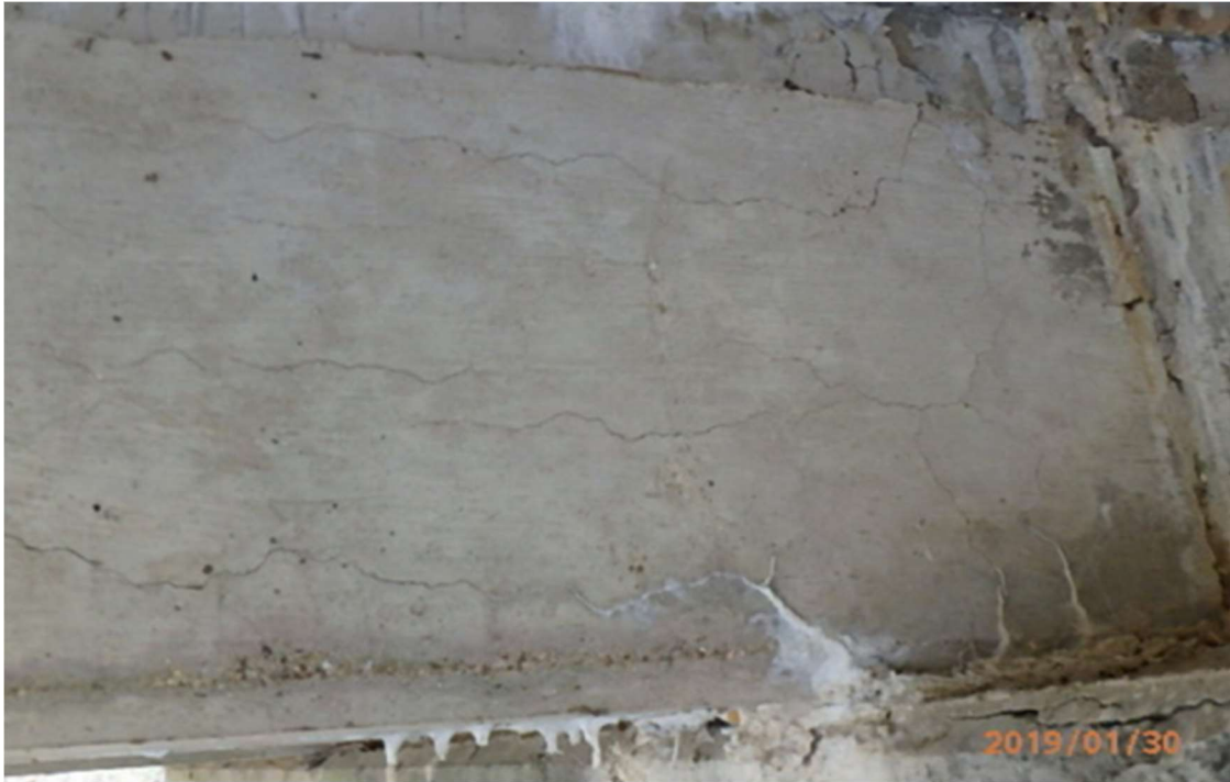
Figure 96 – Bridge 295-0039-0 Concrete Cracking (GDOT, 2019)
