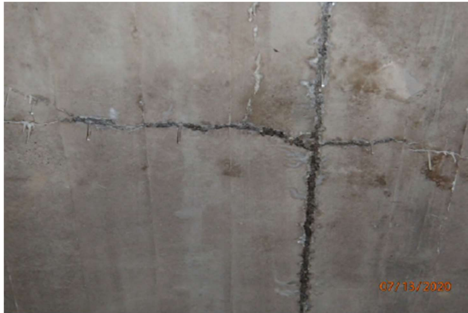
Figure 261 – Bridge 241-0016-0 Deck Cracking Underside (GDOT, 2020)
