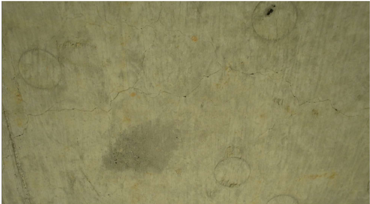
Figure 104 – Bridge 083-0026-0 Reinforced Concrete Girder Typical Cracking (GDOT, 2019)
