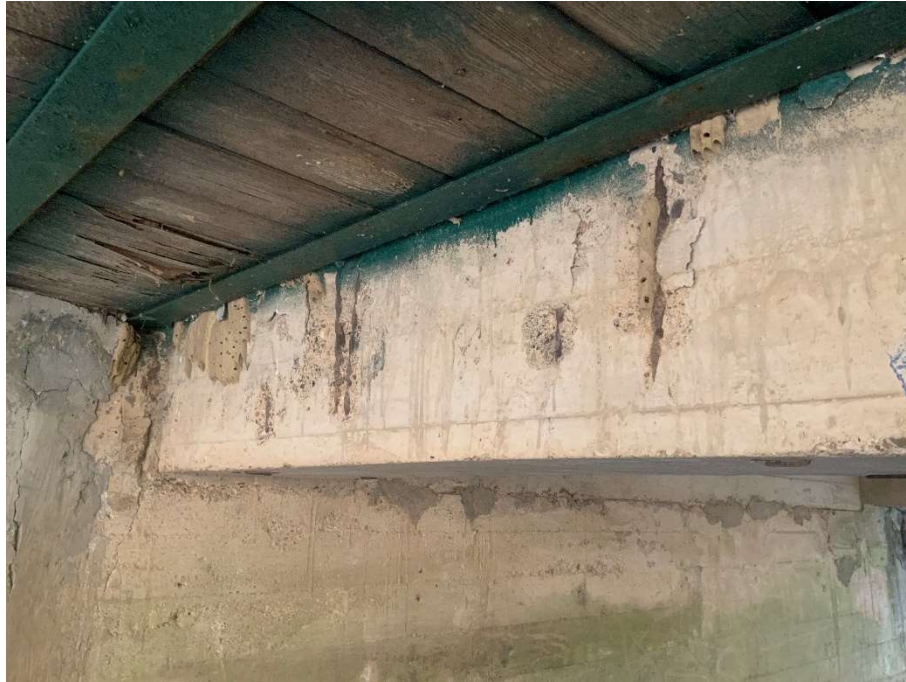
Figure 114 – Bridge 295-0040 Reinforced Concrete Girder Spalling (GDOT, 2023)
