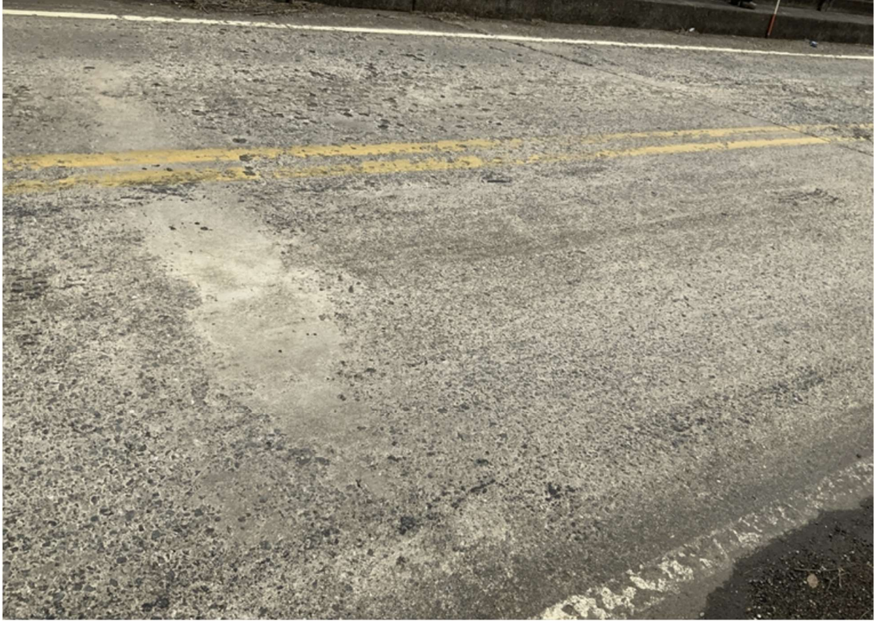
Figure 264 – Bridge 157-5046-0 Reinforced Concrete Top Flange Concrete Spall with Loose Aggregates (GDOT, 2022)
