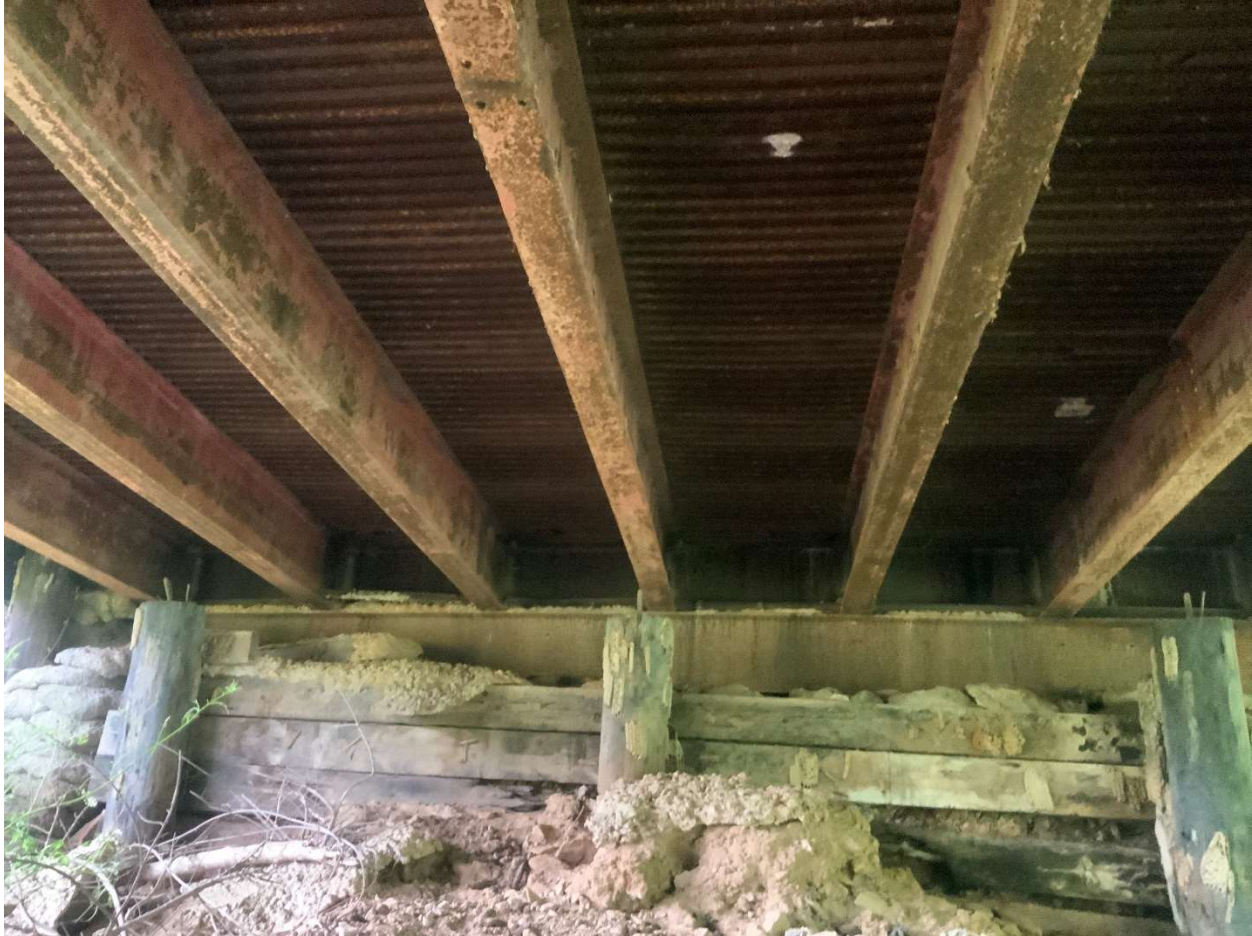
Figure 236 – Bridge 045-5126-0 Steel Abutment Condition (GDOT, 2021)
