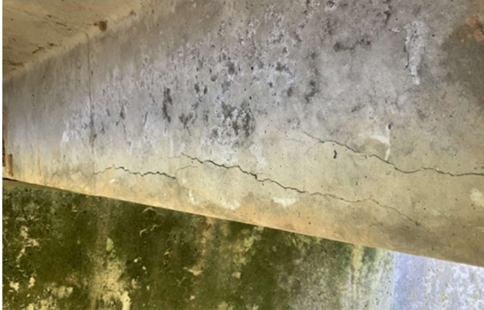
Figure 146 – Bridge 313-5028-0 Span 2 Cracking (GDOT, 2022)
