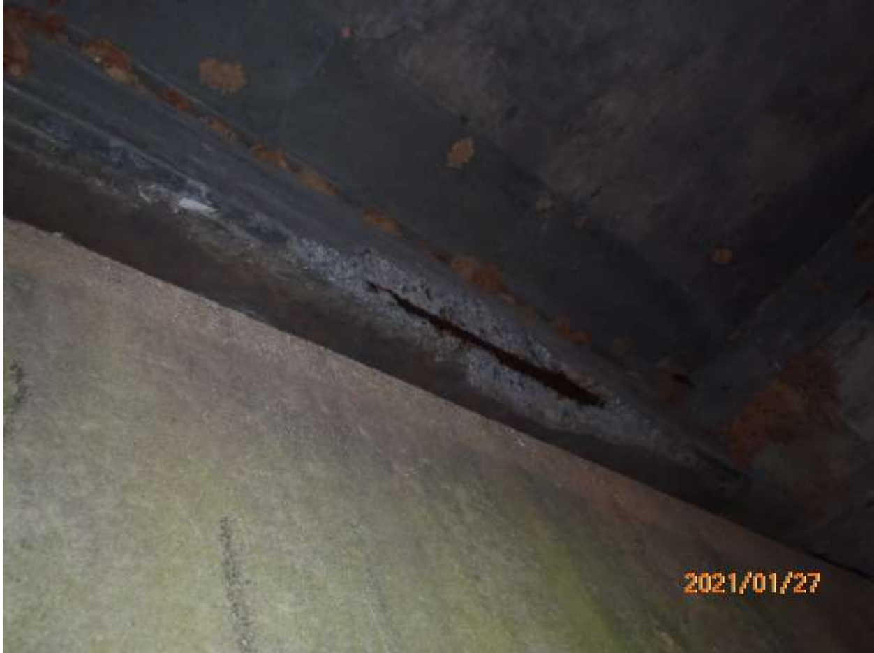
Figure 257 – Bridge 257-0012-0 Concrete Spalling (GDOT, 2021)
