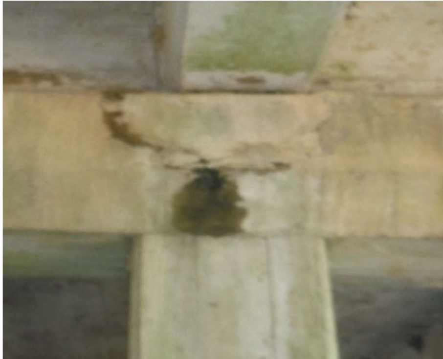
Figure 130 – Bridge 295-5013-0 Reinforced Concrete Pier Cap Cracking (GDOT, 2021)
