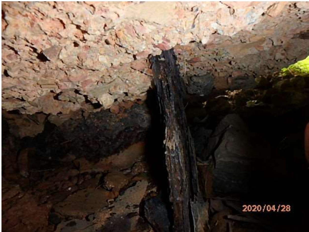
Figure 190 – Bridge 313-5008-0 Abutment pile 100% Section Loss (GDOT, 2020)
