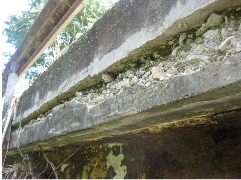
Figure 167 – Bridge 055-5030-0 Deck Condition (GDOT, 2022)
