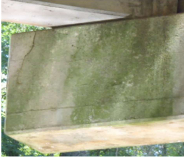
Figure 140 – Bridge 291-0018-0 Reinforced Concrete Pier Cap Cracking (GDOT, 2018)
