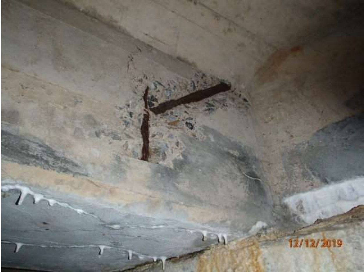
Figure 250 – Bridge 187-0007-0 Concrete Spalling 2013 (Top) vs 2019 (Bottom)
