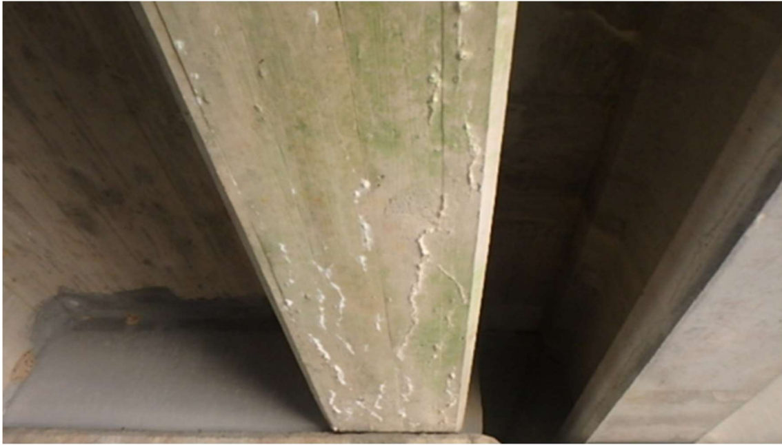
Figure 112 – Bridge 295-0004-0 Reinforced Concrete Girder Cracking with Efflorescence (GDOT, 2020)
