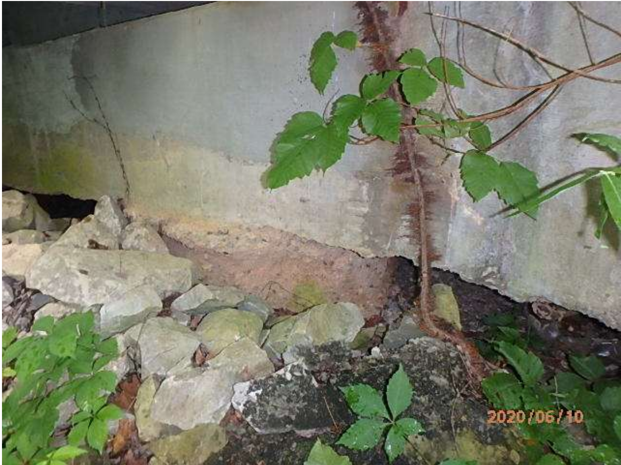
Figure 204 – Bridge 313-5083-0 Abutment Undermining (GDOT, 2020)
