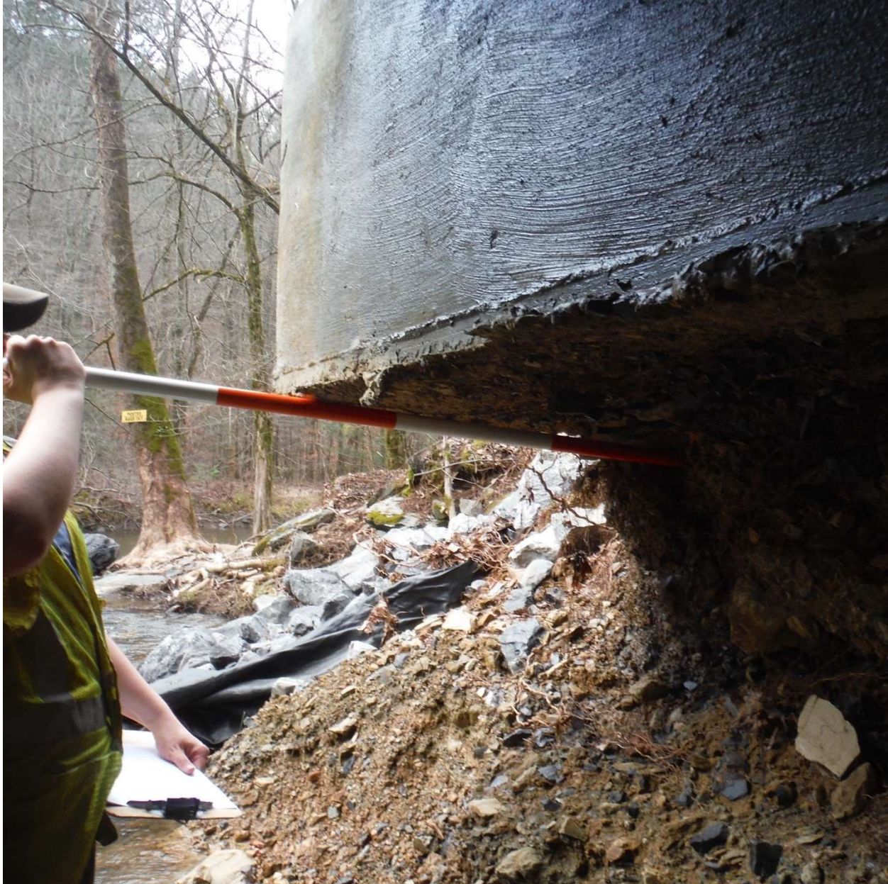
Figure 208 – Bridge 213-5044-0 Abutment One Scour (GDOT, 2016)
