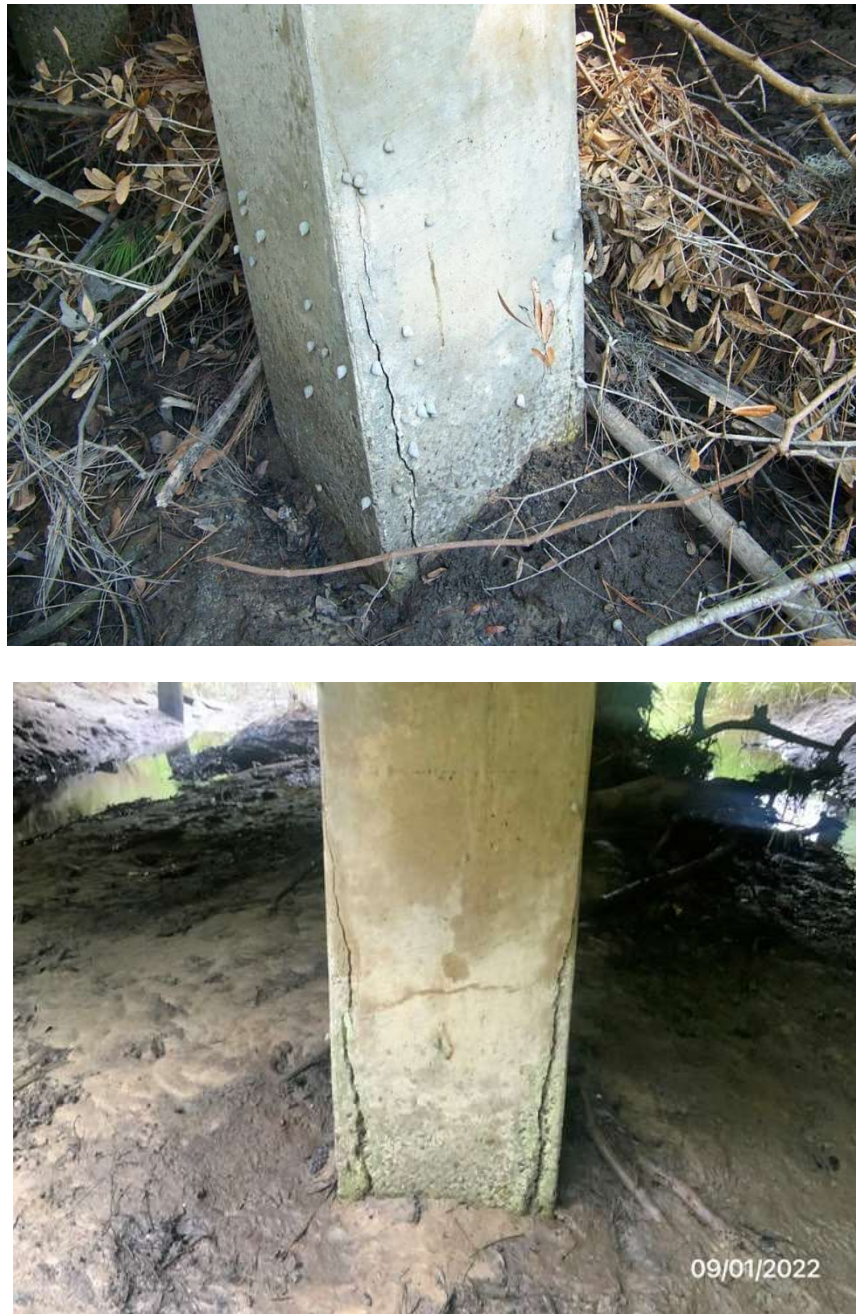
Figure 292 – Bridge 051-0142-0 Pile Cracking 2014 (Top) vs 2022 (Bottom)
