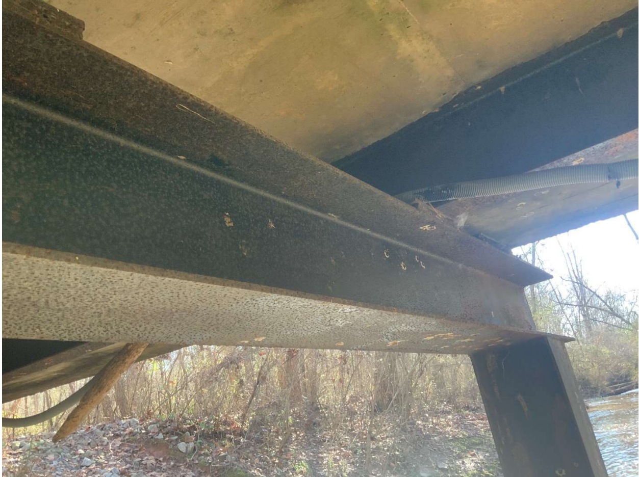
Figure 230 – Bridge 231-5002-0 Steel Pier Cap Condition 2016 (Top) vs 2022 (Bottom)
