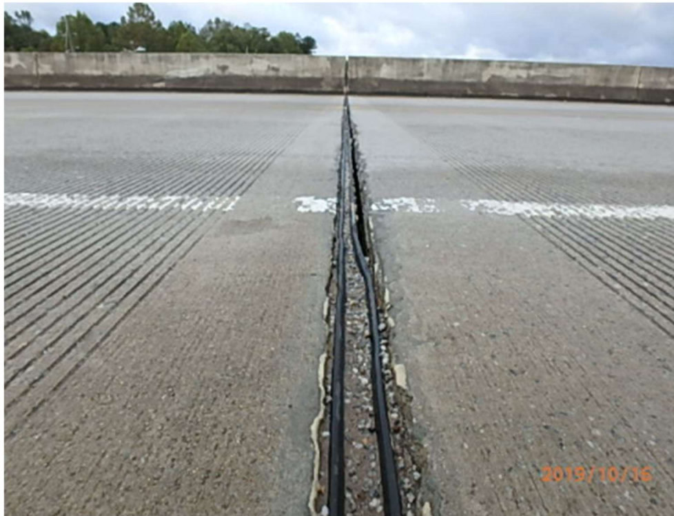
Figure 222 – Bridge 097-5059-0 Failing Joint (GDOT, 2019)
