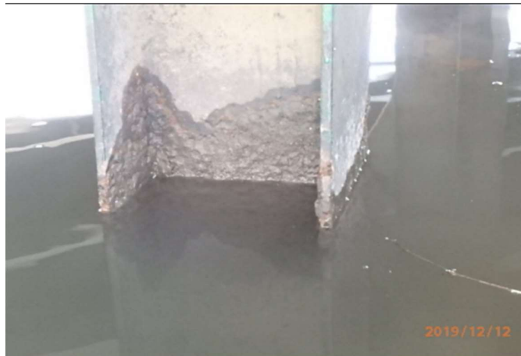
Figure 161 – Bridge 0047-5012-0 Typical Steel Pile Section Loss (GDOT, 2019)
