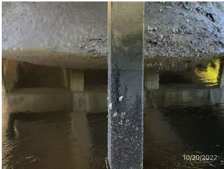
Figure 299- Bridge 127-0034-0 Bent 3 Pile 2 Cracking 2014 (Top) vs 2022 (Bottom)
