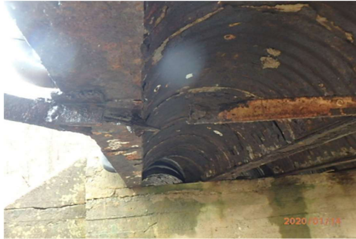
Figure 64 - 100% Section Loss in Lateral Bracing (GDOT, 2020)
