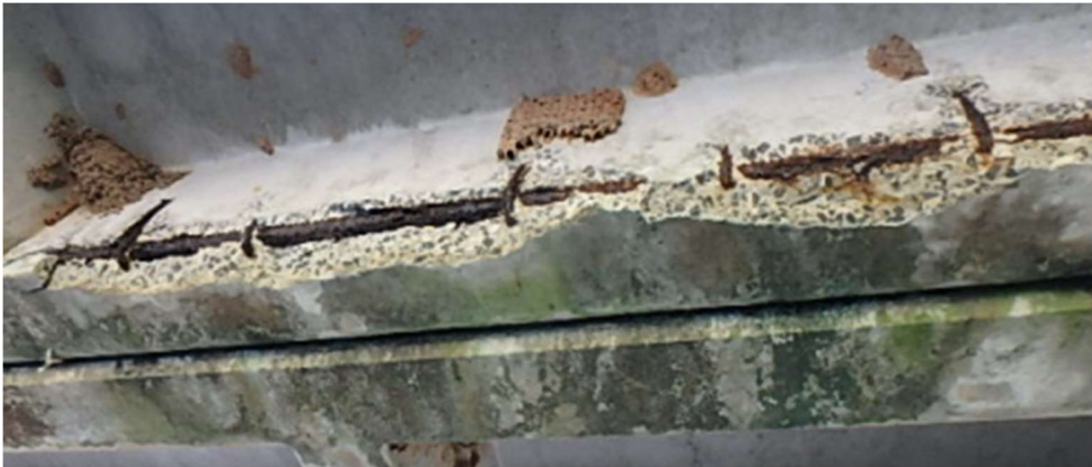
Figure 147 – Bridge 313-5028-0 Span 1 Spalling (GDOT, 2020)
