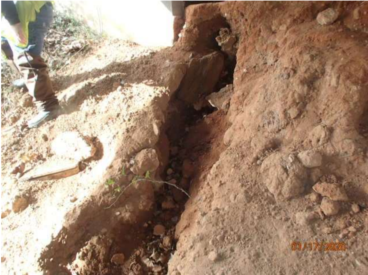
Figure 206 – Bridge 311-0040-0 Erosion (GDOT, 2020)
