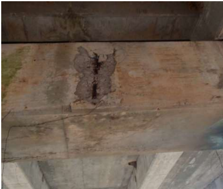
Figure 212 – Bridge 187-0016-0 Bent Cap 9 Spalling 2020 (Top) vs 2022 (Bottom)
