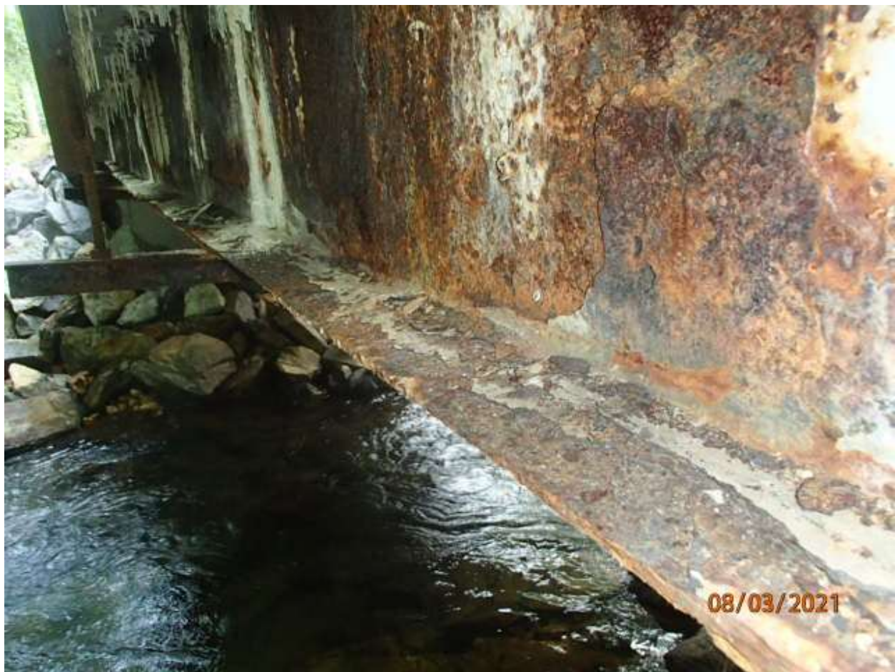
Figure 274 – Bridge 291-5044-0 Steel Beam Corrosion (GDOT, 2021)
