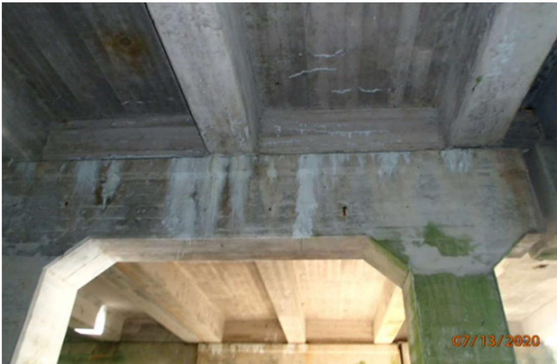
Figure 155 – Bridge 241-0016-0 Efflorescence at Reinforced Concrete Top Flange (GDOT, 2020)
