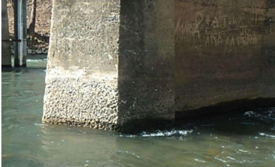
Figure 185 – Bridge 213-0044-0 Typical Pier Wall Abrasion (GDOT, 2020)
