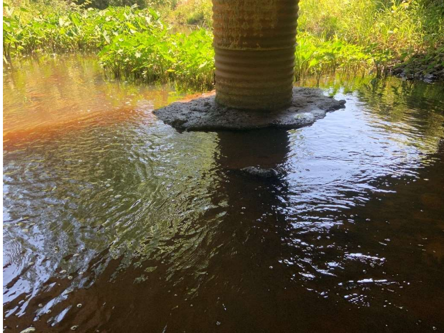
Figure 232 – Bridge 175-5086-0 Scour (GDOT, 2021)
