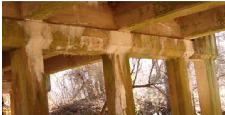
Figure 122 – Bridge 295-5012-0 Reinforced Concrete Pier Cap Efflorescence (GDOT, 2017)
