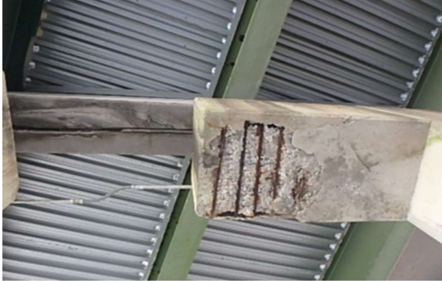
Figure 124 – Bridge 083-0012-0 Reinforced Concrete Pier Cap Spalling with Exposed Rebar (GDOT, 2019)
