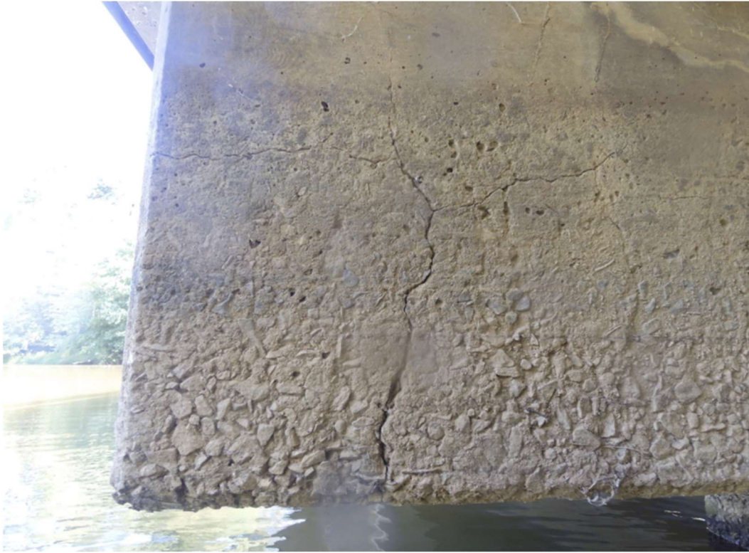
Figure 133 – Bridge 311-5001-0 Pier Cap Cracking (GDOT, 2018)
