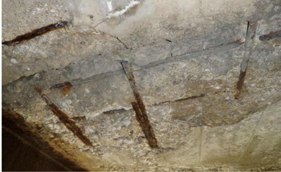
Figure 79 – Bridge 055-5030-0 Deck Spalling (GDOT, 2022)
