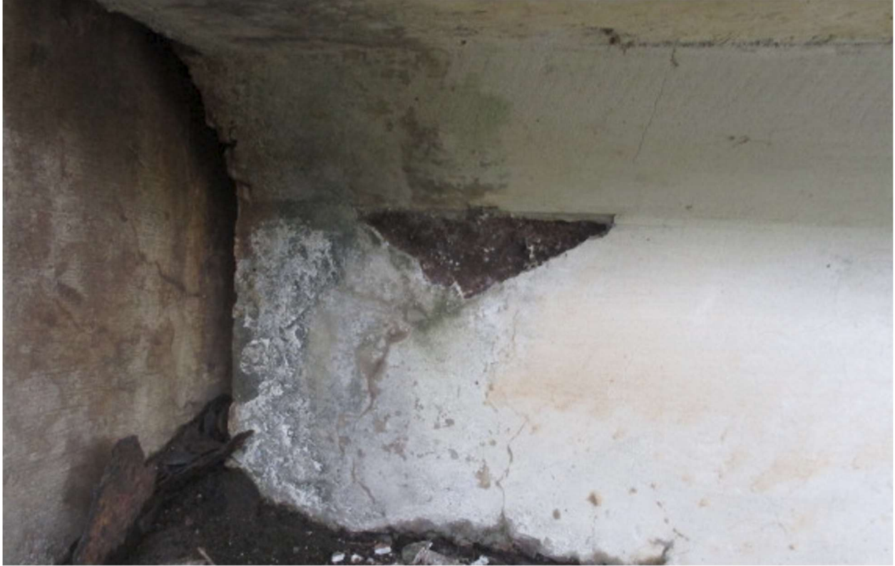
Figure 108 – Bridge 083-0027-0 Reinforced Concrete Girder Spalling (GDOT, 2019)
