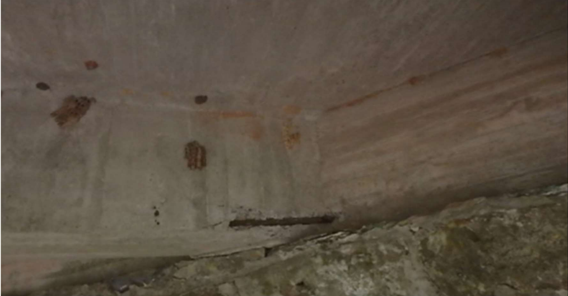
Figure 102 – Bridge 055-5037-0 Reinforced Concrete Girder Spalling (GDOT, 2020)
