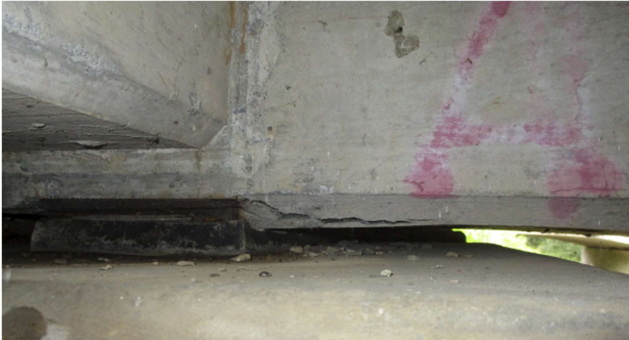
Figure 110 – Bridge 083-0027-0 Reinforced Concrete Girder Spalling (GDOT, 2019)
