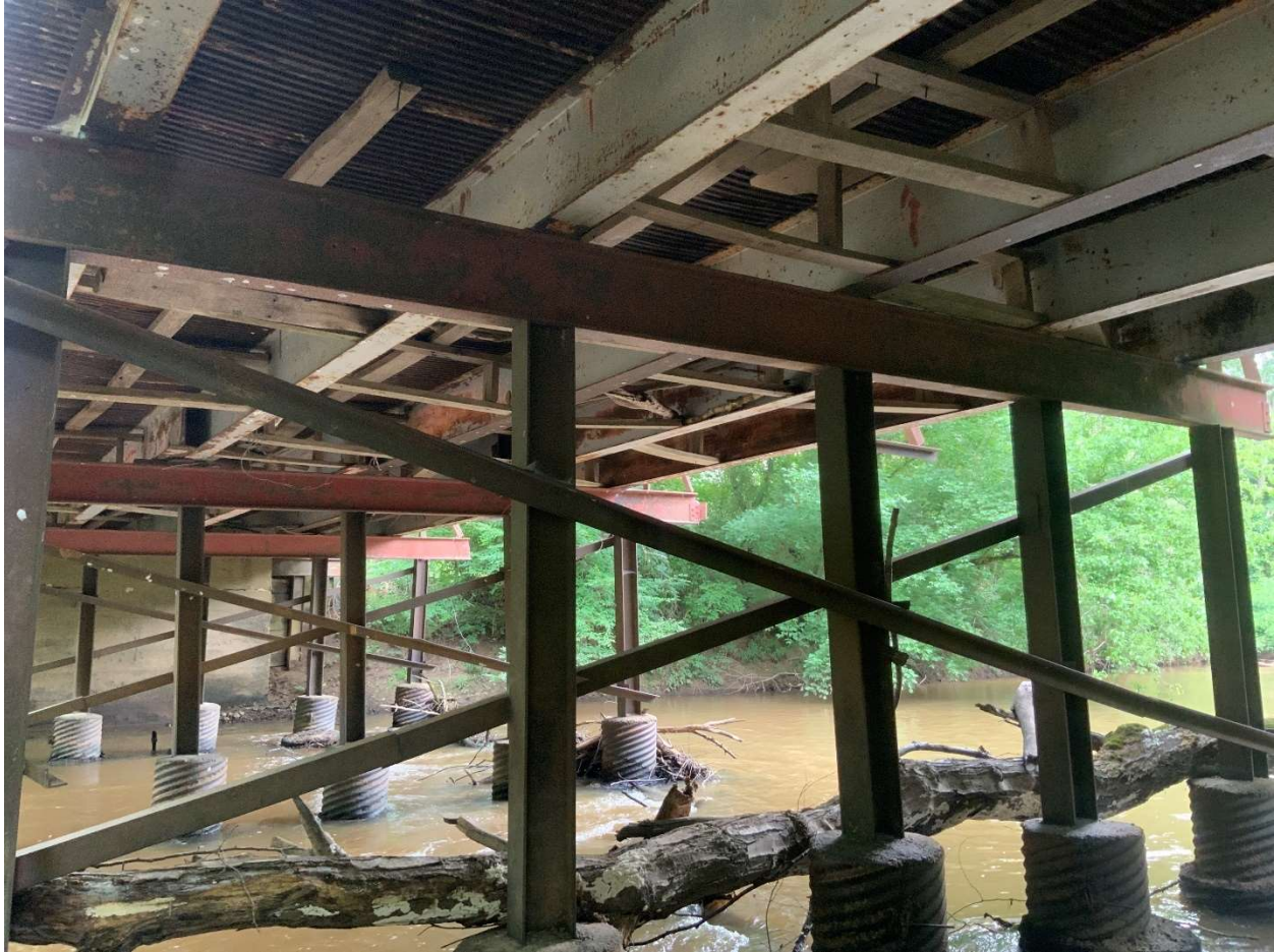
Figure 228 – Bridge 045-0079-0 Steel Pier Cap 2014 (Top) vs 2022 (Bottom)
