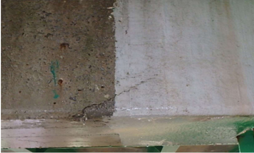
Figure 136 – Bridge 213-0001-0 Reinforced Concrete Pier Cap Cracking in Wrap Repair (GDOT, 2020)
