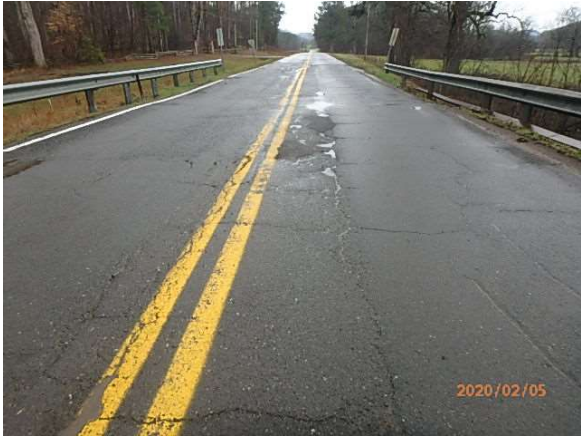
Figure 273 – Bridge 213-0044-0 Deck Condition 2014 (Top) vs 2016 (Middle) vs 2020 (Bottom)
