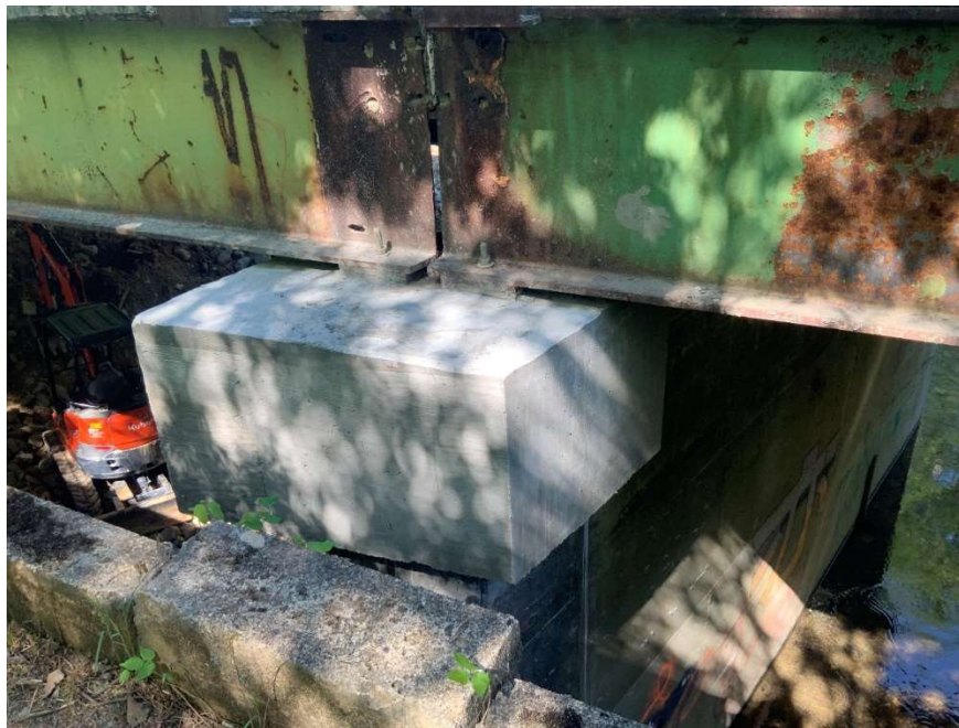
Figure 189 – Bridge 313-5008-0 Pier Wall Spall (Top) vs Repaired (Bottom)
