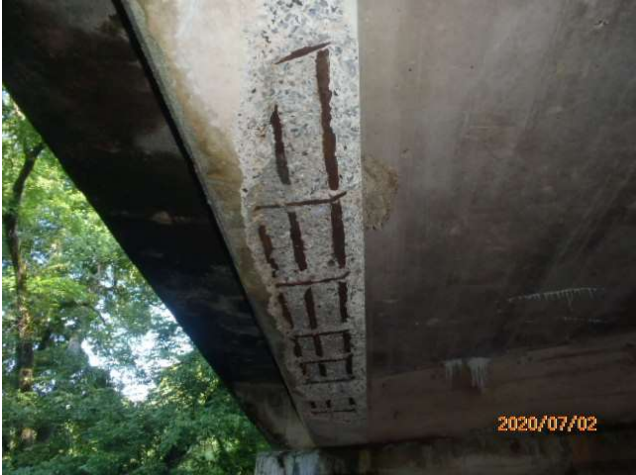
Figure 246 – Bridge 241-5036-0 Span 3 Beam 3 Concrete Spall 2014 (Top) vs 2020 (Bottom)
