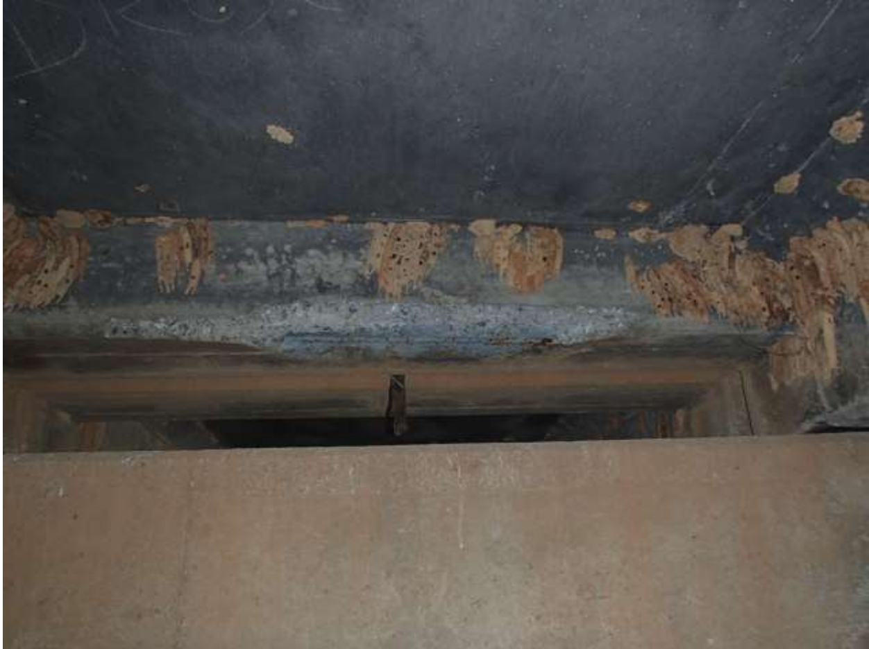
Figure 258 – Bridge 257-0012-0 Concrete Spalling with Epoxy Painting (GDOT, 2021)
