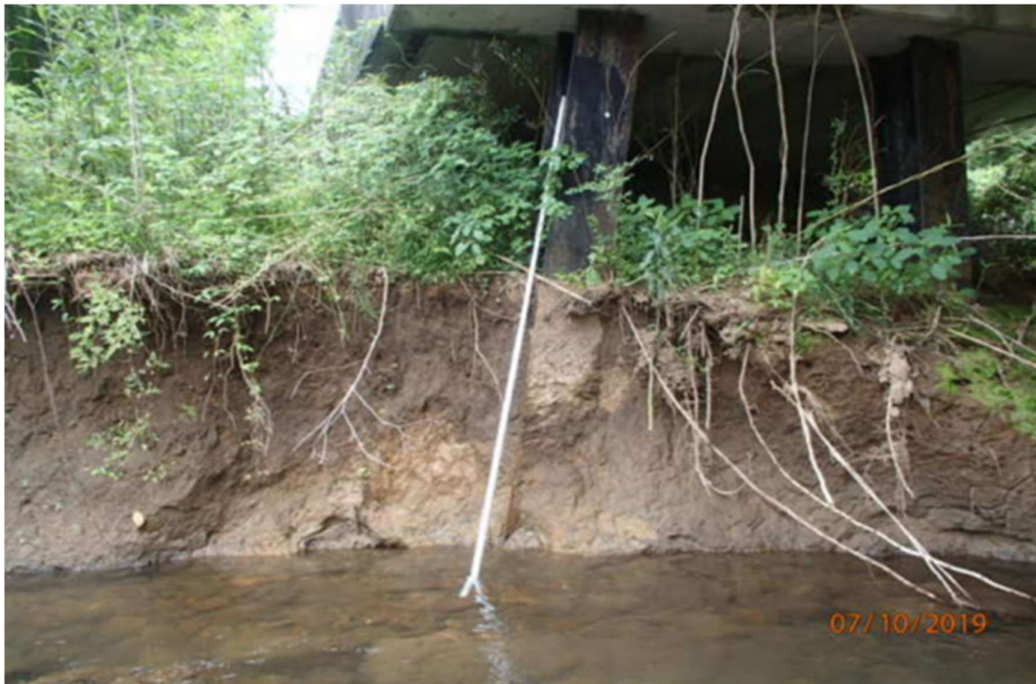
Figure 171 – Bridge 291-5026-0 Scour (GDOT, 2019)
