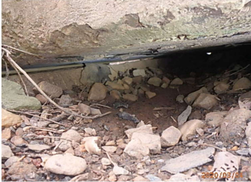
Figure 216 – Bridge 123-0036-0 Abutment Void (GDOT, 2020)
