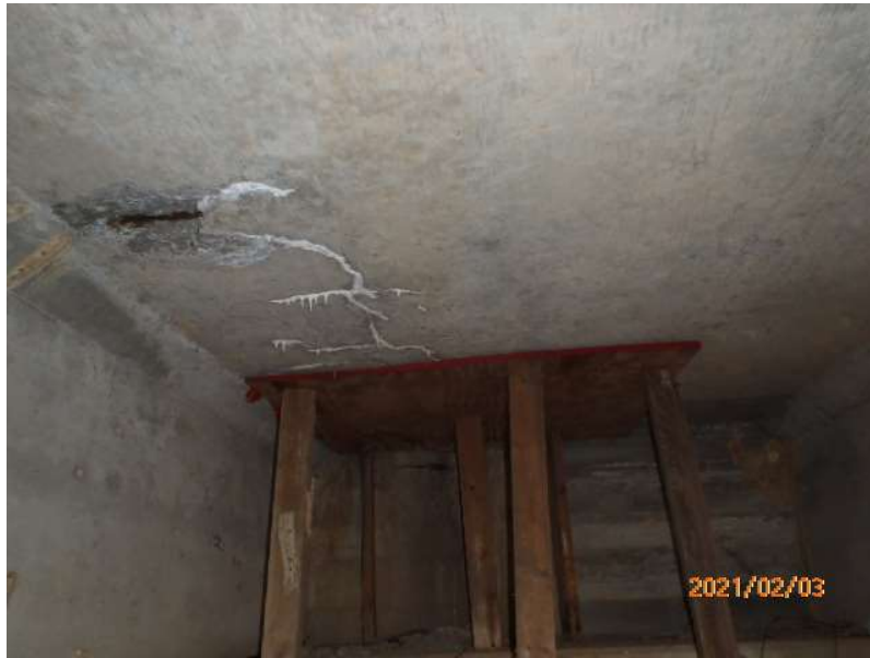
Figure 254 – Bridge 257-0008-0 Bridge Spalling Under Span 3 2015 (Top) vs 2021 (Bottom)
