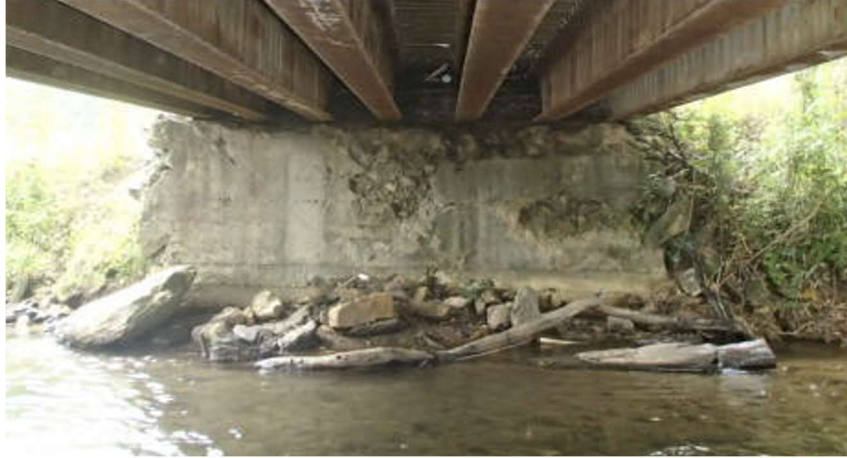
Figure 41: Concrete Spalling in Abutment 1 in 2014 (Left) and 2021 (Right)
