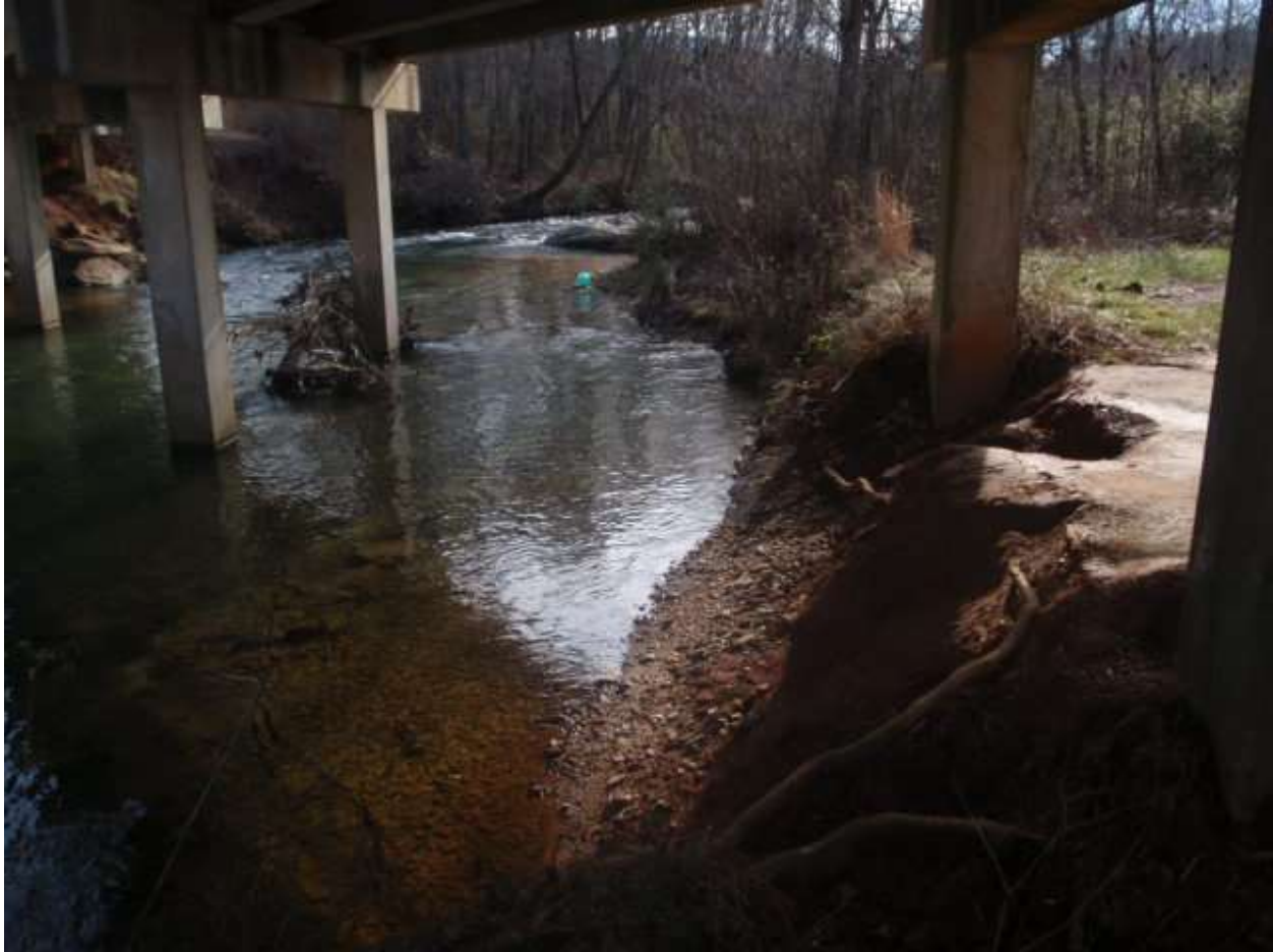
Figure 244 – Bridge 291-0018-0 Bridge Erosion (GDOT, 2014)
