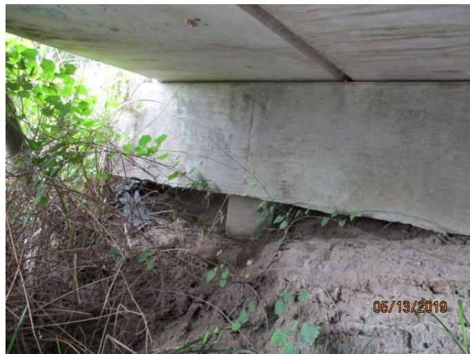
Figure 293 – Bridge 039-0051-0 Abutment Undermining (GDOT, 2019)
