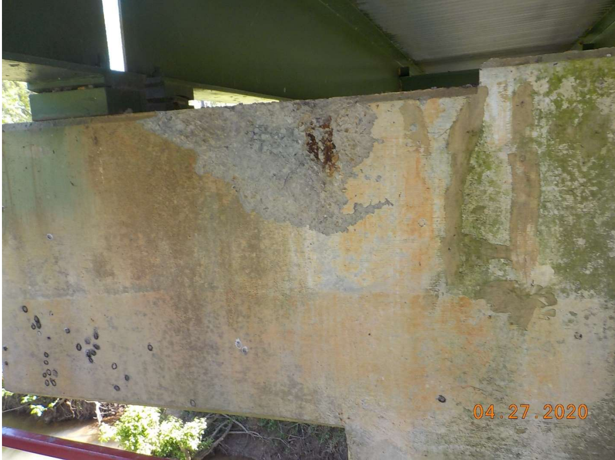
Figure 211 – Bridge 187-0016-0 Bent Cap 5 Spalling (GDOT, 2020)
