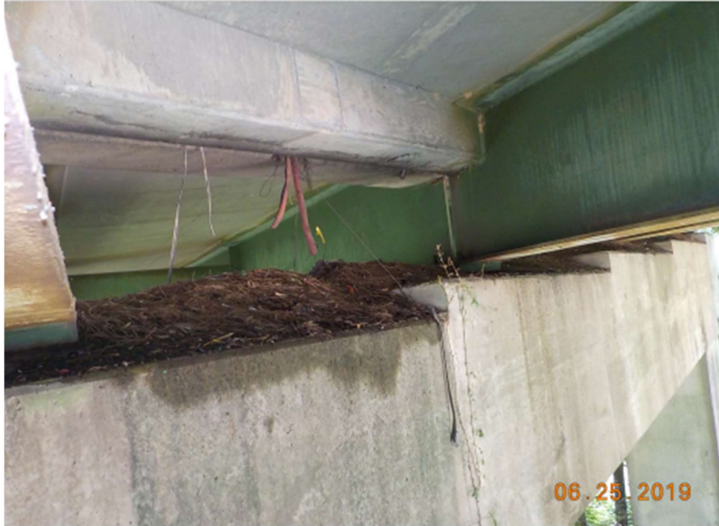
Figure 225 – Bridge 089-0131-0 Debris Build Up on Bent Cap 3 (GDOT, 2019)
