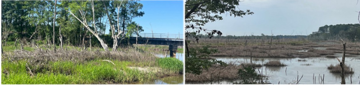
Figure 2.1: A healthy NI system dominated by salt-intolerant vegetation (left) compared to the same area affected by saltwater from the downstream after the damage of an existing gray structure (tide gate) by a storm event (right).
