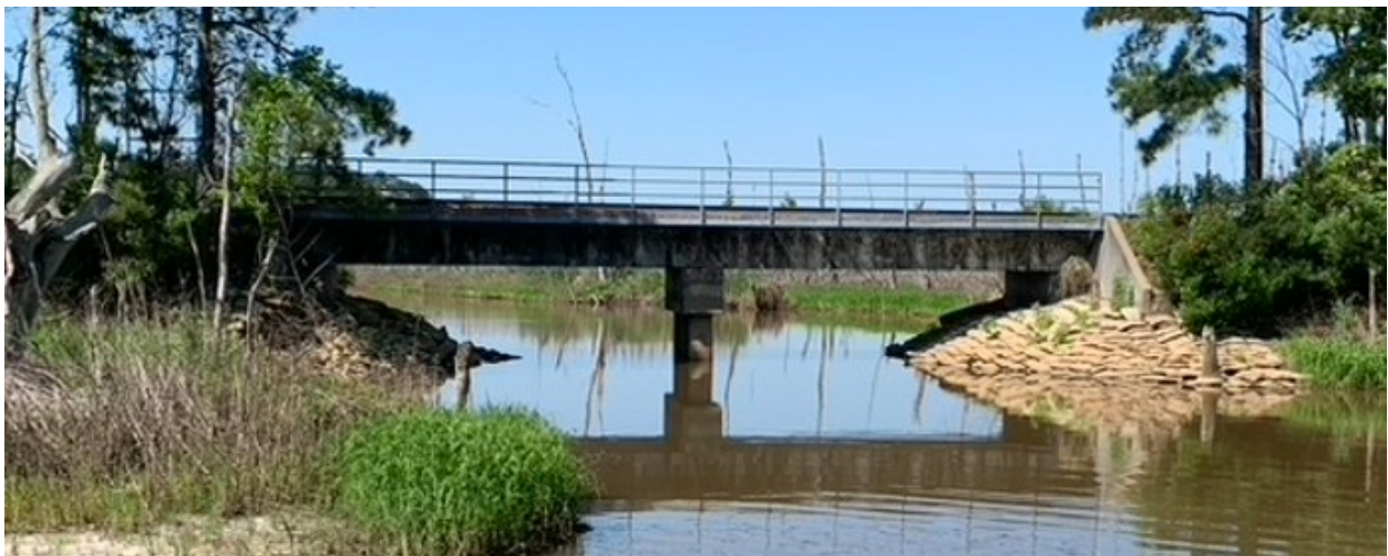
Figure 3.5: The railroad crossing at Hunter Army Airfield at the start of the field work, with sand bags at the base of the railroad crossing to protect the base of the structure from intense flow.
