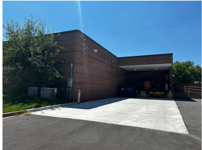
Figure B95: West elevation of the Overland Park Post Office (Haylee Rose, 2024).
