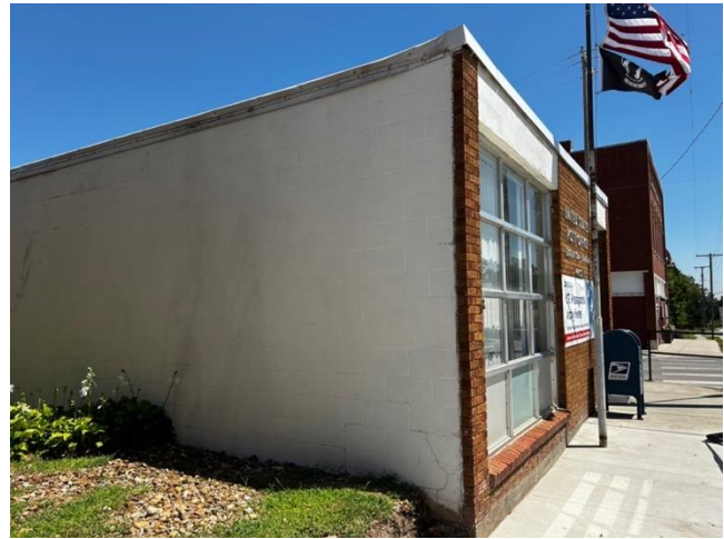
Figure B20: Eastern oblique of the Edgerton Post Office illustrating the concrete masonry unit construction on the side and rear elevations with a brick veneer on the front elevation (Haylee Rose, 2024).
