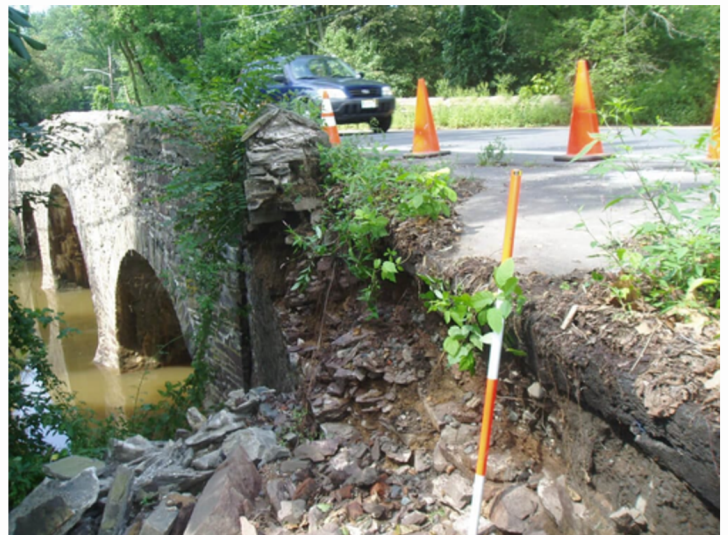
Figure 14. Failed abutment on historic bridge in the Northeast U.S. [16].
