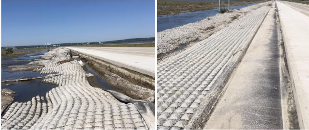
Figure 3.4. (Left to right) Failed Flood Protection Geomats, Asphalt Wedge Working to Maintain Geomat Stability, from Bowers & Gu (2021).
