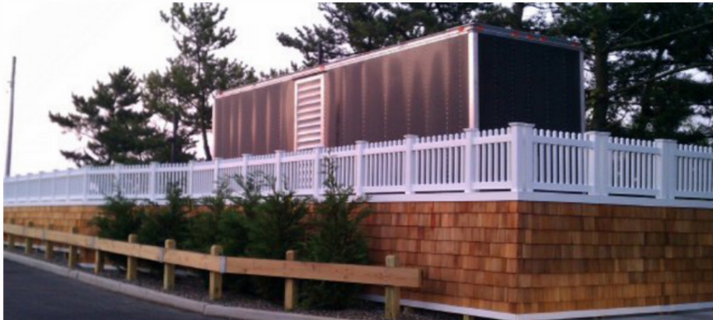
Figure 24. A mobile trailer for pump controls from South Monmouth Regional Sewerage Authority in Monmouth County, NJ [27].
