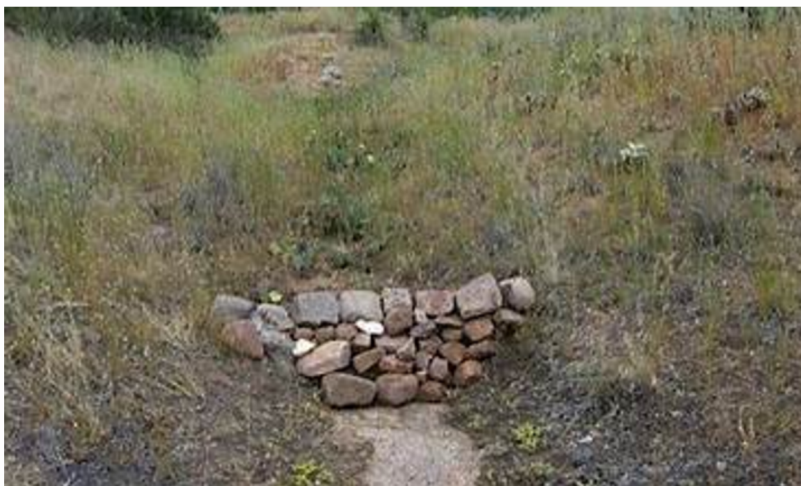
Figure 19. Small rock check dam [22].
