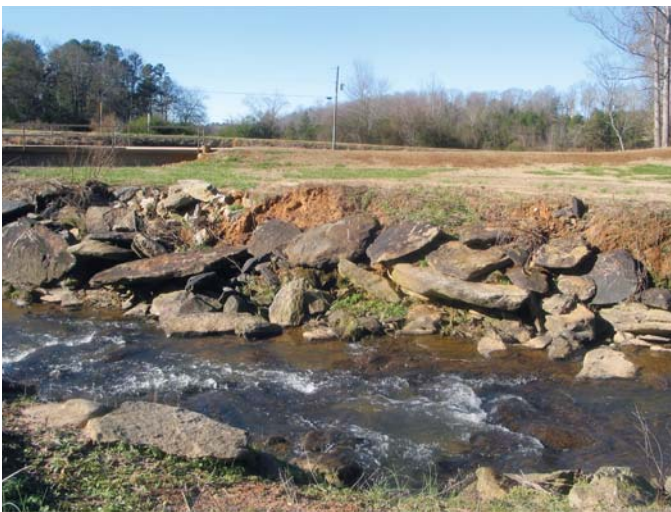
Bank erosion is the most common concern reported by riparian landowners (Hazel Creek).
