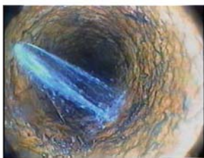
Figure 2. Casing leak in alluvial zone
