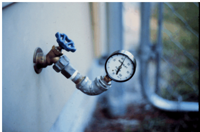
Figure 10. Pressure gauge on outside faucet.
