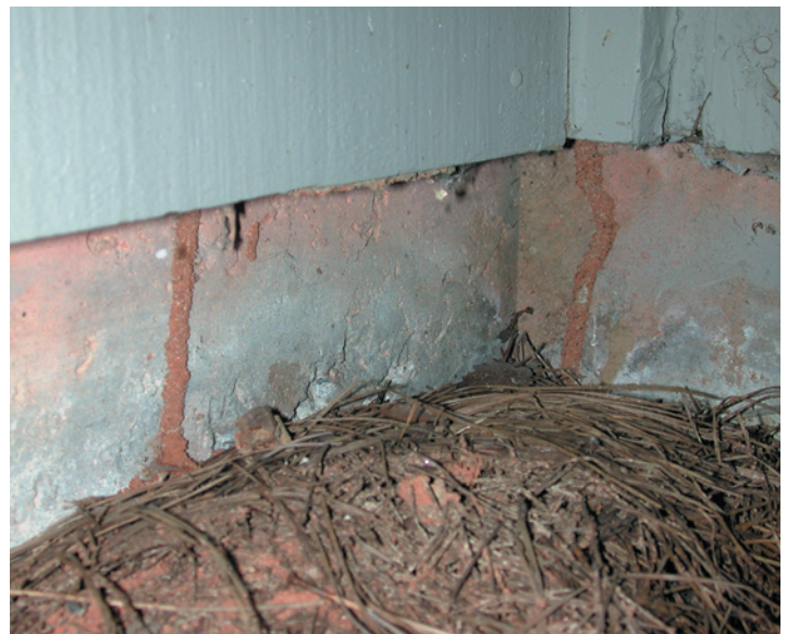
Figure 21. Property owners should keep mulch away from their building's foundation to allow inspectors to detect the presence of termites moving from the soil into the structure. In these pictures, mulch is piled next to the structure (top), and when removed exposes termites entering the structure through shelter tubes (bottom).
