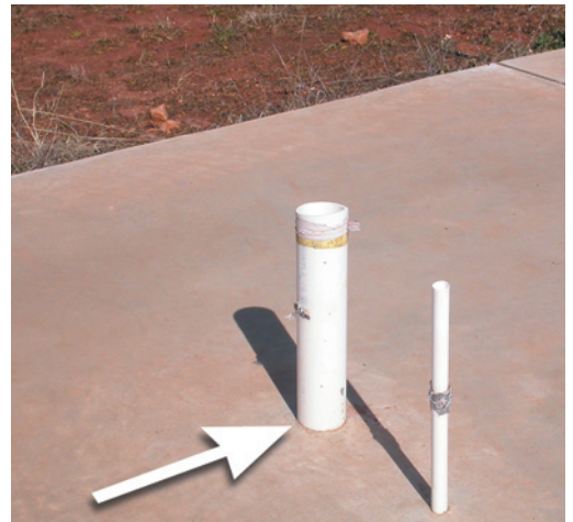
Figure 14. In slab construction, termites often enter the structure via gaps (arrow) that develop between utility pipe penetrations and concrete.
