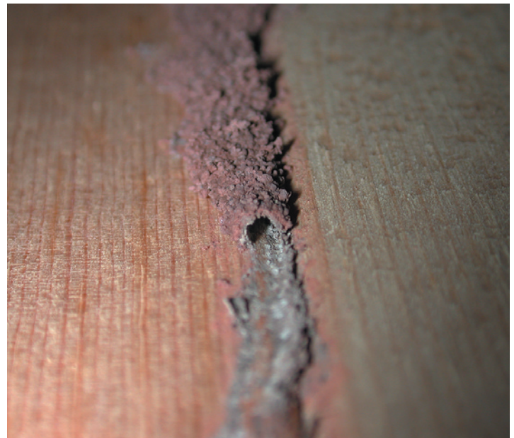
Figure 10. Termites move inside the path delineated by the shelter tube.
