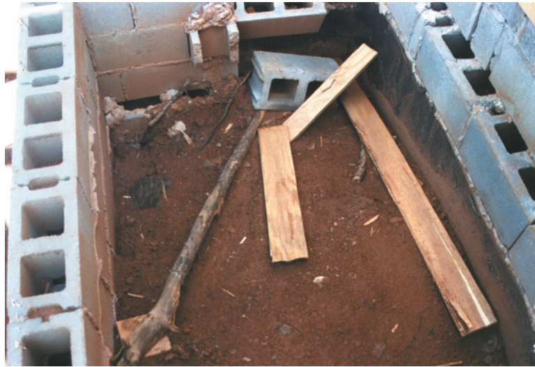
Figure 17. Often times, raised porches are used as dump sites by construction crews. Wood material dumped into these voids places at risk future wood elements in close proximity.
