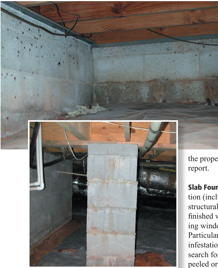
Figure 13. When inspecting raised foundations, look for evidence of termites on and in wood where it first interfaces with concrete construction elements—such as foundation walls (top) and piers (bottom).
