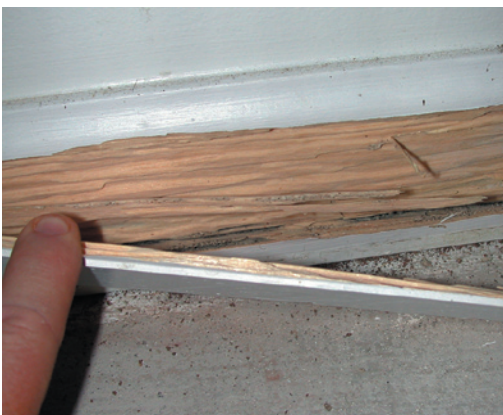
Figure 8. Subterranean termites will consume or damage structural wood (top) as well as door frames, paneling, carpet, and baseboards.
