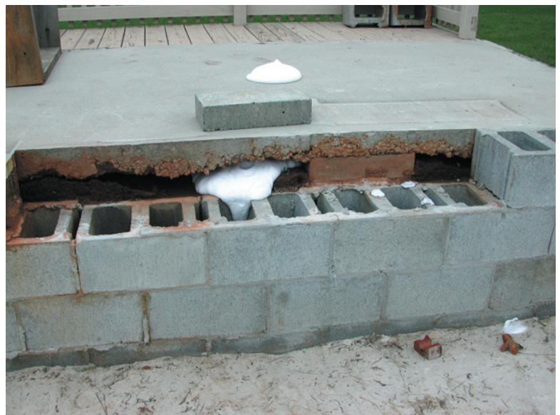
Figure 18. Foaming can be an effective treatment technique when treating areas containing voids, such as those under some porches (shown here) and inside walls, because the foam expands to treat all surfaces.
