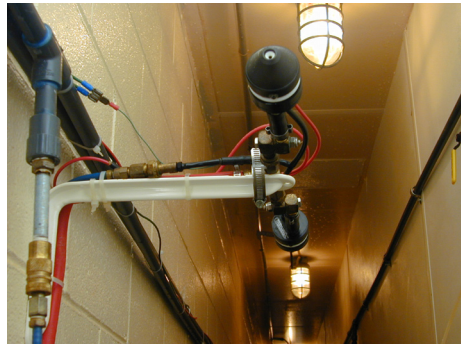
Figure 2. Electrostatic spray nozzle in a hatchery plenum.
