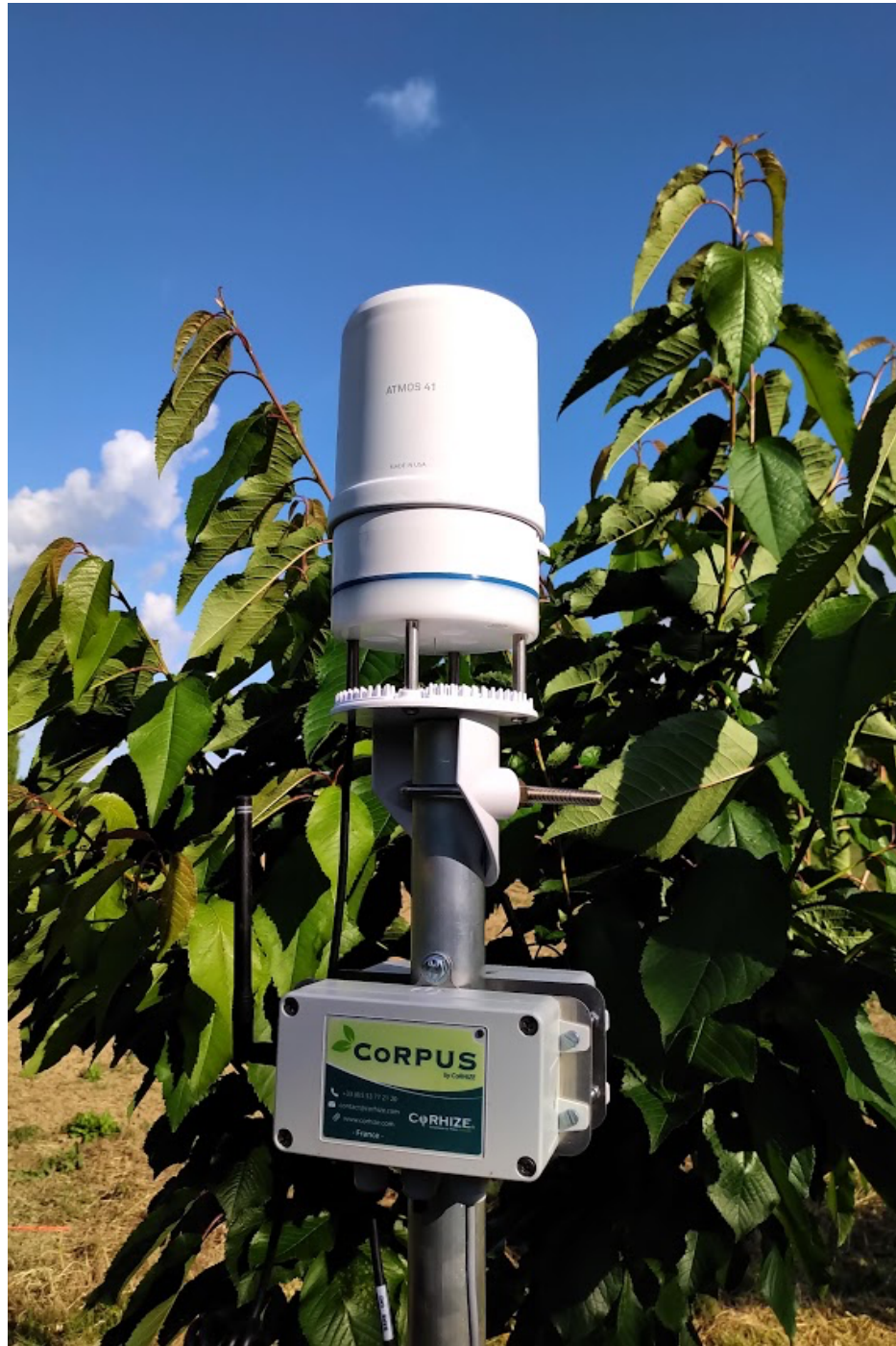
Figure 2.20. Installed ATMOS 41 weather station used to sense meteorological parameters.
