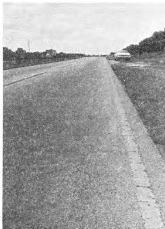
FIGURE 59. LONG. CRACKING IN LAKE WALES SAND-ASPHALT BASE SECTION AFTER 1.75 \times 10^6 EQUIV. LOADS - 3 IN. AC SURFACE AND 6 IN. BASE
