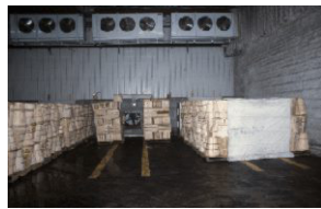
Figure 47. Commercial forced air cooling system.
