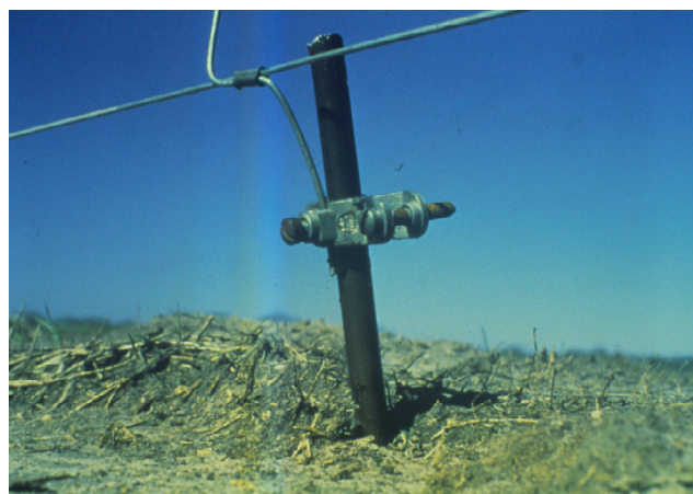
Figure 13. Driven ground rod for grounding an electric fence.
