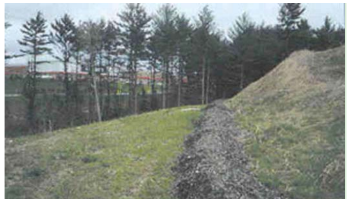
Ground wood waste being used in a berm for erosion and sediment control.
