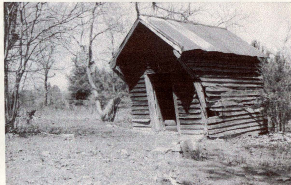
Fig. 4 – Small storage shed, showing signs of neglect.
