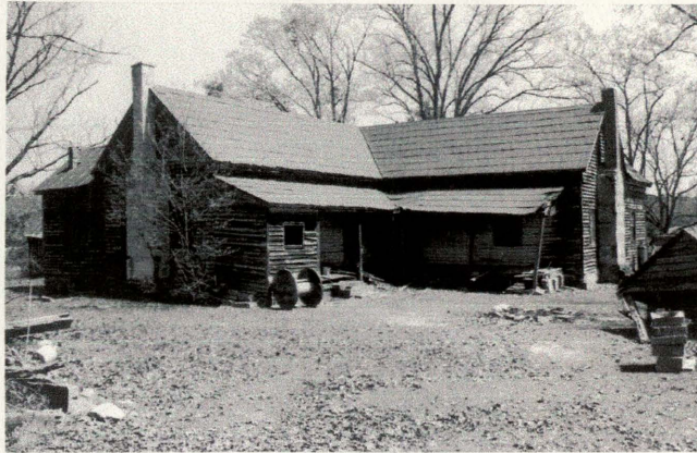
Fig. 8 – The house viewed from southwest. The collapsed smokehouse is visible at lower left; the well shed roof at the right. Note collapsed rear porch and broken window in the addition.
