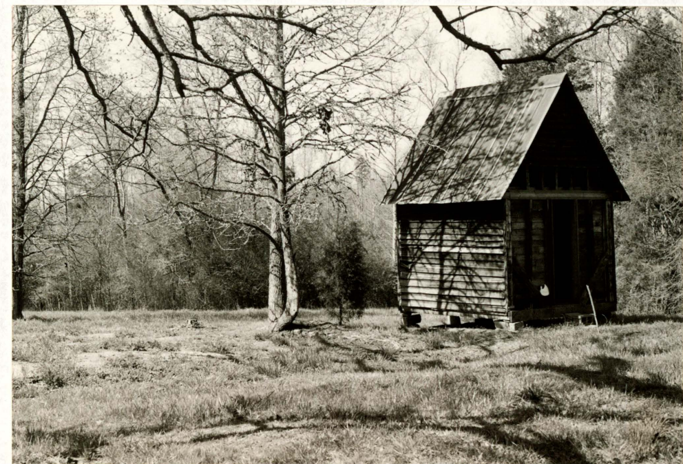
The location of the demolished Milking Shed and the Storage Shed. Note the missing weatherboard and new bracing.
