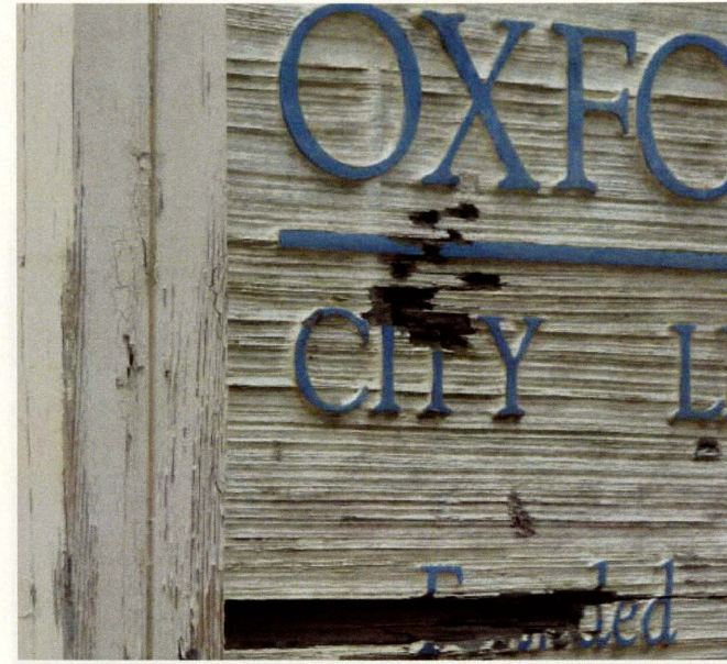
Poorly maintained welcome to Oxford signs
