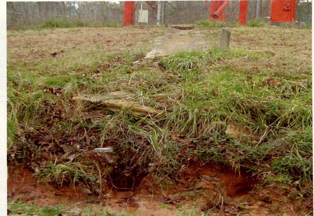
Erosion from pipe draining water tower
