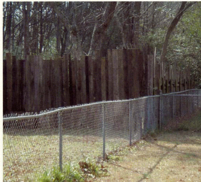
Proliferation of chain link fences that degrades and is rarely removed or replaced as well as privacy fences whether wooden or metal cause city to look clustered and inconsistent
