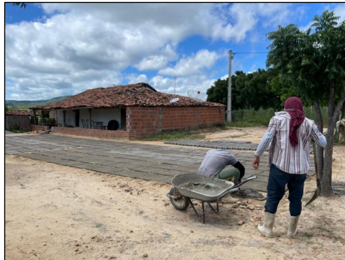
Figure 4.1 Two bricklayers finish forming the concrete slabs that were used to construct household rain-harvesting cisterns in Tunísia, Quixeramobim, Ceará in May 2022. (Source: Author)
