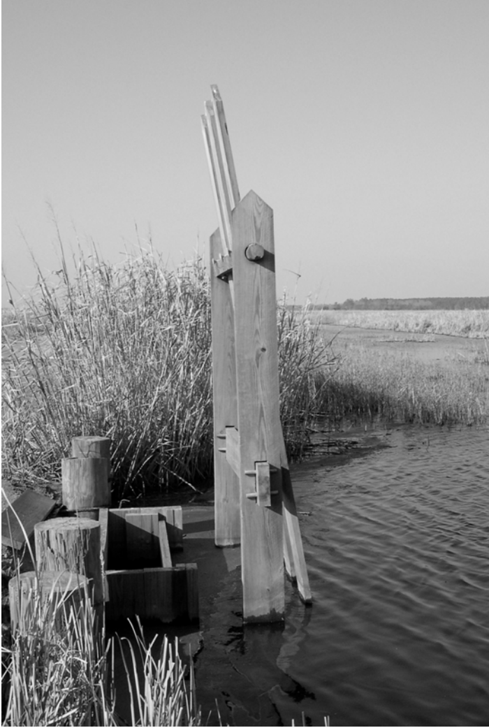
Figure 1.1. The flapgate and flashboards of a water control structure (ricefield trunk) used in impoundments managed for waterfowl. The trunk connects a managed impoundment to a natural water source such as a tidal river, or connects two impoundment compartment as shown here.
