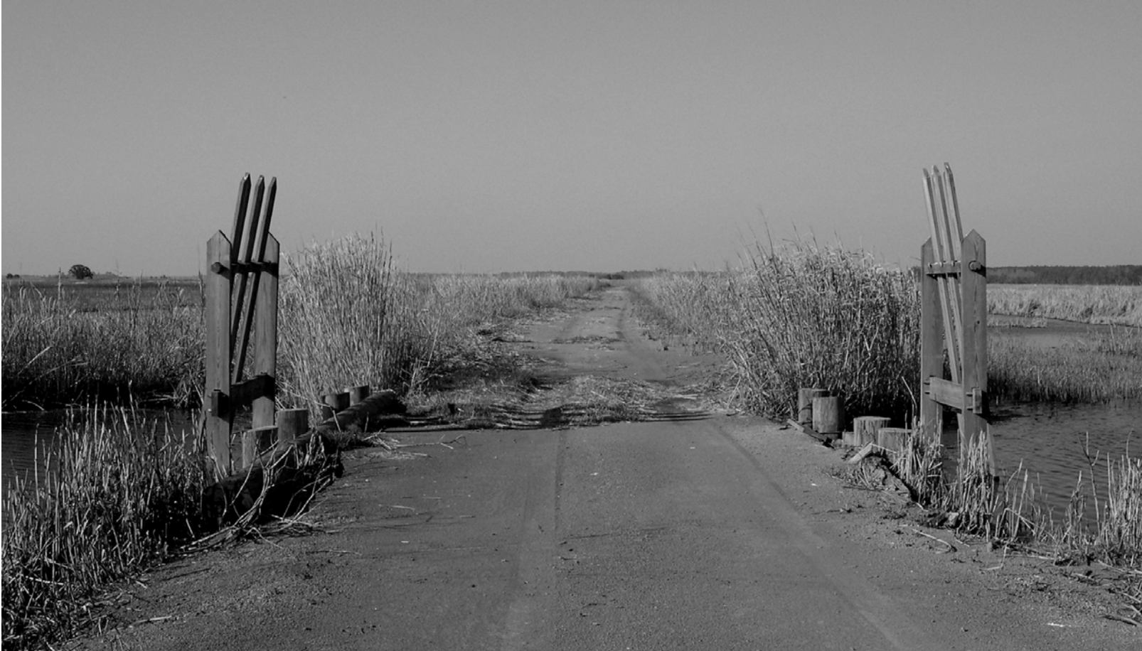
Figure 1.2. A water control structure (ricefield trunk) used in impoundments managed for waterfowl. To drain a managed impoundment, a manager opens the inside flap gate on the trunk to draw water out of the impoundment and into the natural water source, or between impoundment compartments as shown here.
