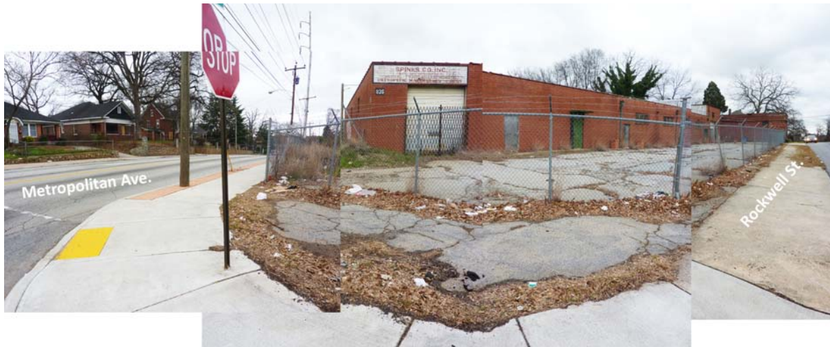
Figure 5. 47 Corner of Metropolitan Ave. and Rockwell St. (Landers, 2012p)
