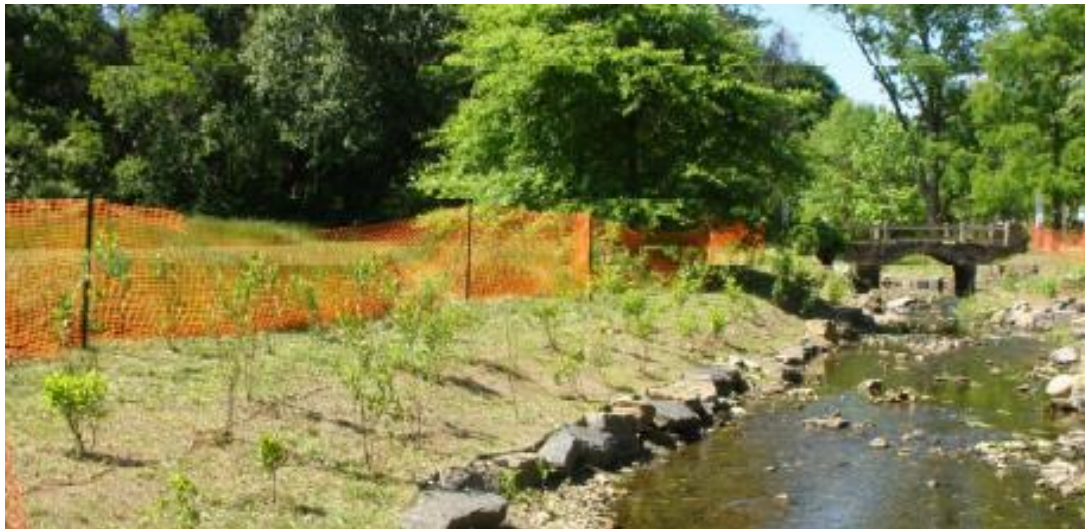
Construction of the first phase of Stream Bank restoration. "Shortridge Memorial Park Master Plan," Township of Lower Merion, 2014, p.24.
