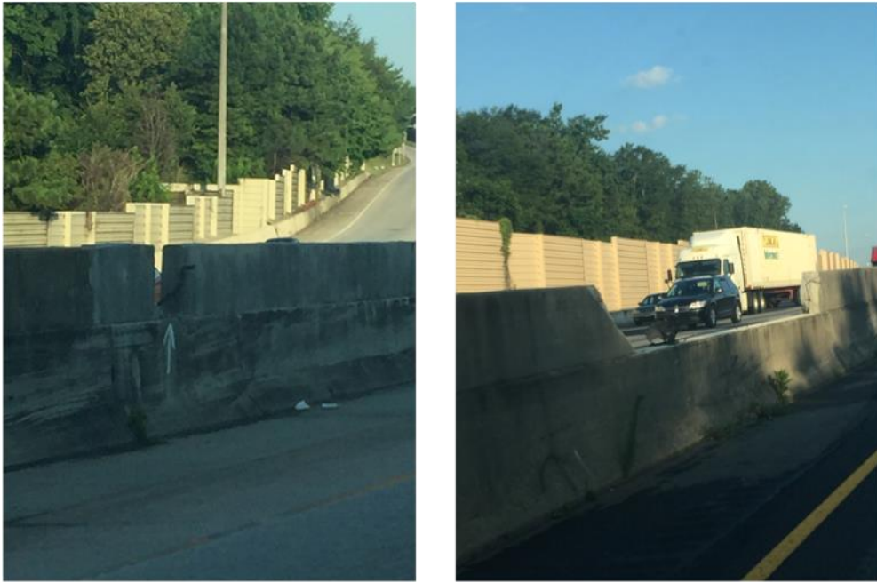
Figure 9-2: Damaged Glare Protection Concrete Sections on EB I-20
