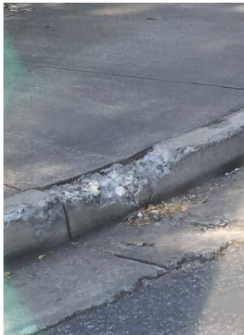
Figure 9-4: Concrete Curb Section Loss
