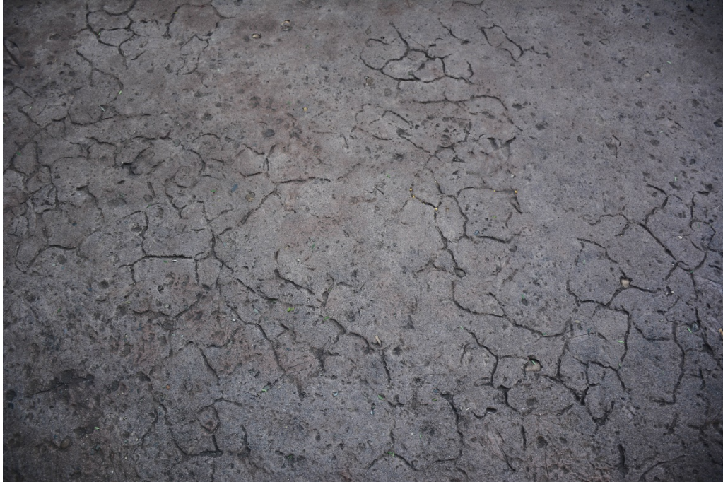
Figure 3.25: Cracks in Pandora pathway. Photo by author.
