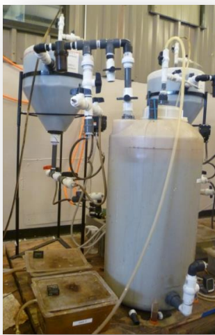
Two-stage pilot digester with bamboo biocarriers
