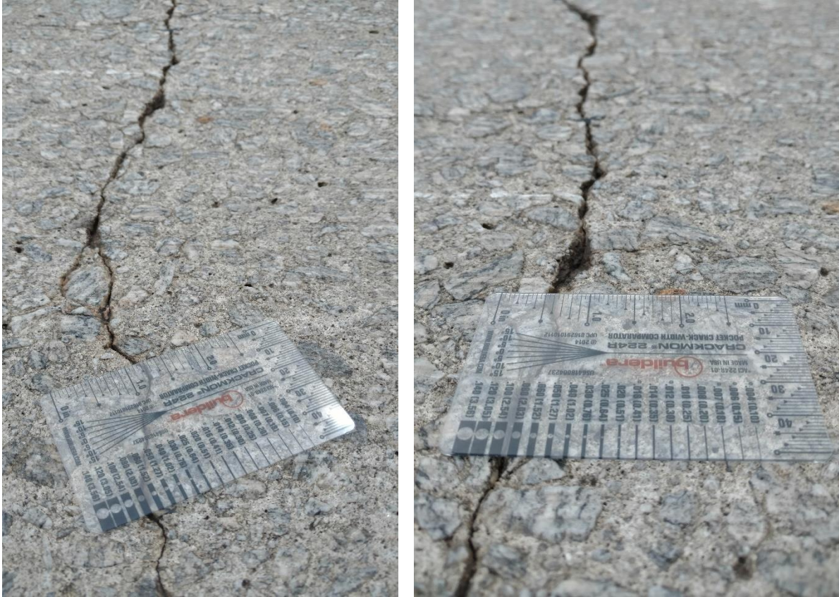
Figure 6.22 – The Measurement of Crack Widths at S3-a
