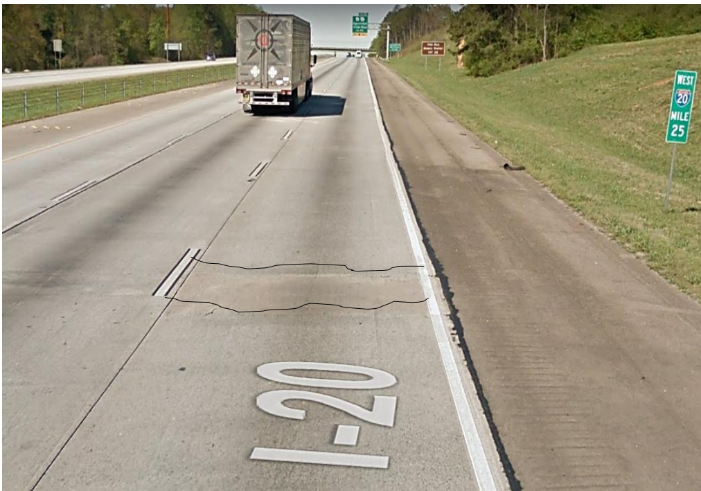
Figure 6.24 – A Patched Area at Outside Lane at S3-b (Google Maps, 2017)
