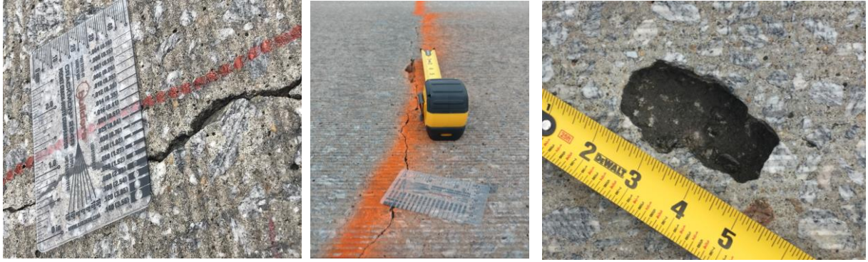
Figure 6.14 – The Measurement of Crack Widths at S2-a and S2-c
