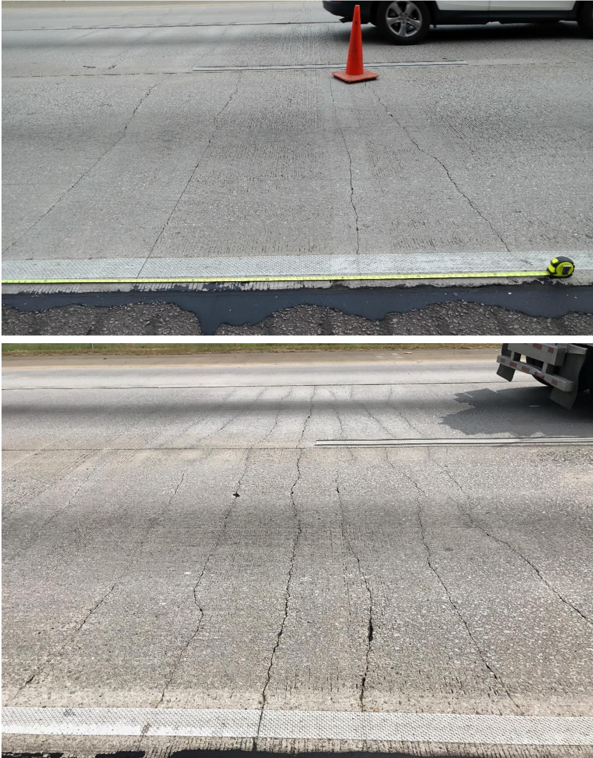
Figure 6.21 – Typical Cluster Transverse Cracks Pattern at S3-a and S3-c
