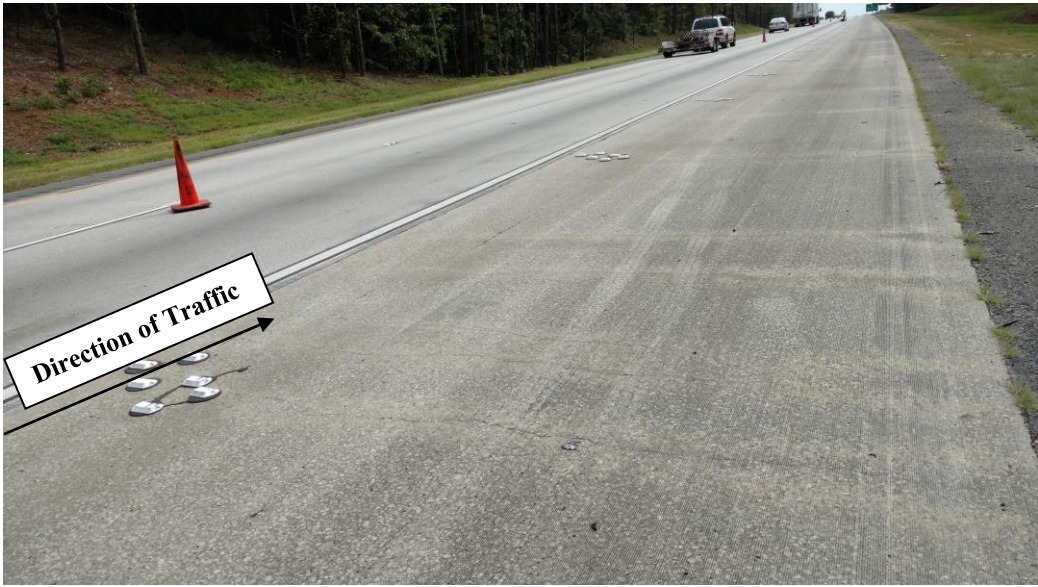
Figure 6.13 – Typical Cluster Transverse Cracks Pattern at S2-a and S2-c
