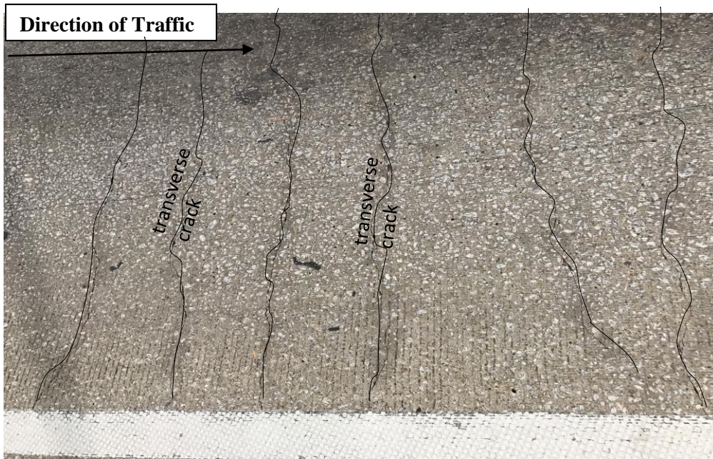
Figure 6.4 – Typical Cluster Transverse Cracks Pattern at S1-a and S1-b
