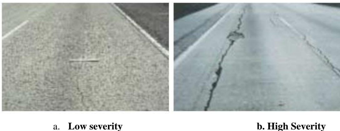
Figure 3.5- The examples of severity levels of longitudinal cracks (FHWA 2003)
