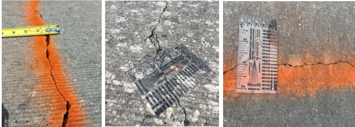
Figure 6.36 – The Measurement of Crack Widths at S4-a and S4-c
