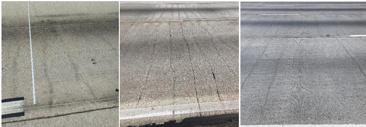
Figure 6.61 – The Density of Transverse Cracks in Sites 1, 3, and 5, respectively
