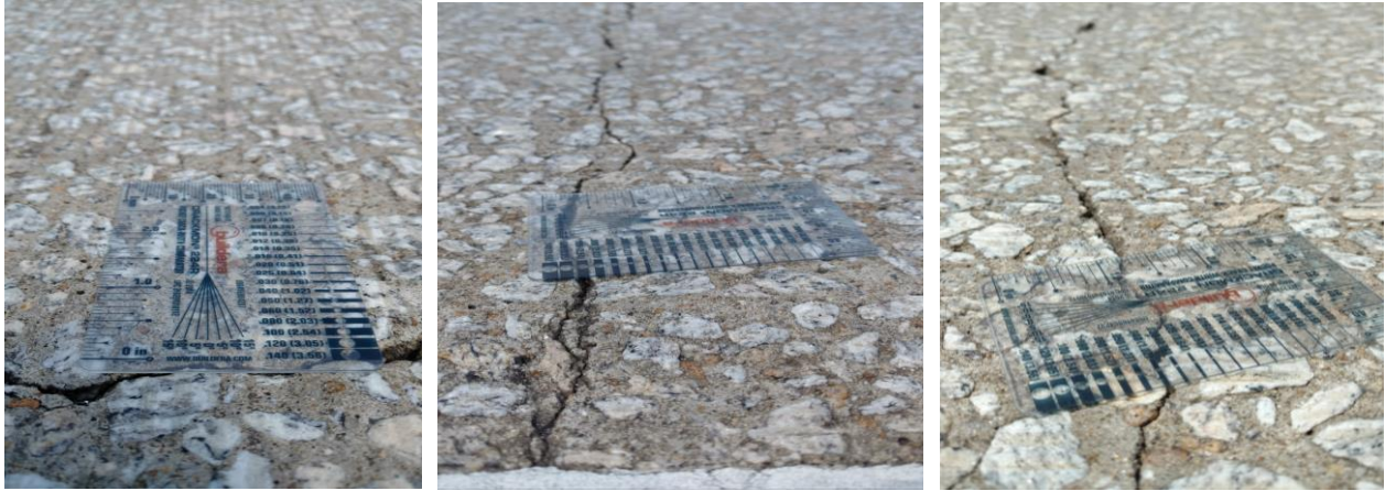
Figure 6.5 – The Measurement of Crack Widths at S1-b, S1-c, and S1-d
